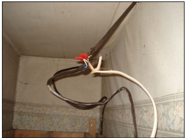
Open splice thingy in a closet.
