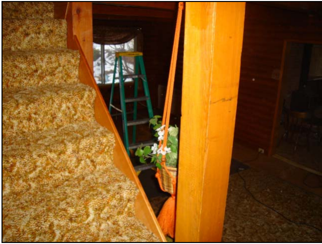
No guard rail for this interior staircase.
