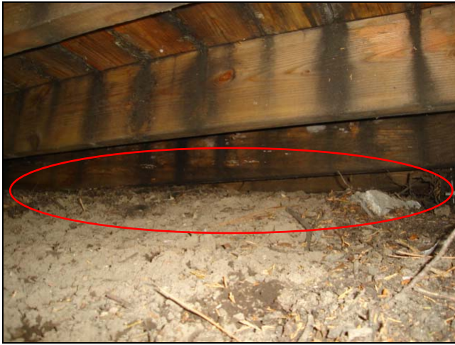
Wood to earth contact for these joists.
