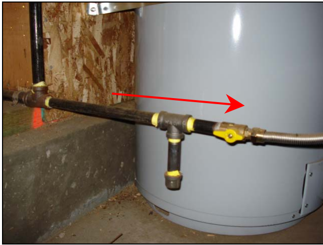
Improper drip leg installation.
