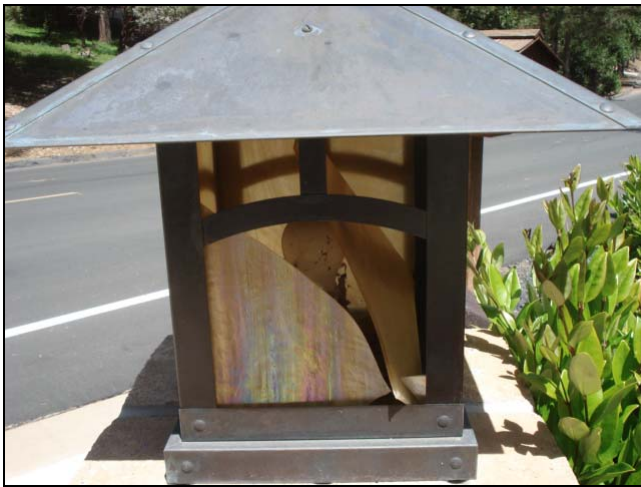
Cracked light fixture lens.
