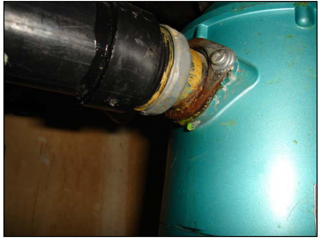
Leaking disposal plumbing fitting.
