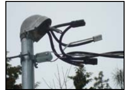
Mast, weatherhead, drip loops and anchor point.
