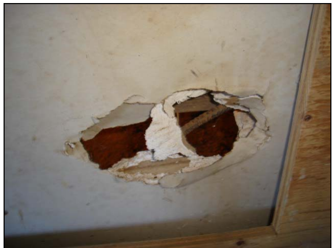
Big ugly hole in the wall.
