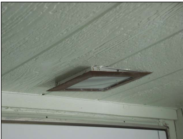
Loose light fixture.
