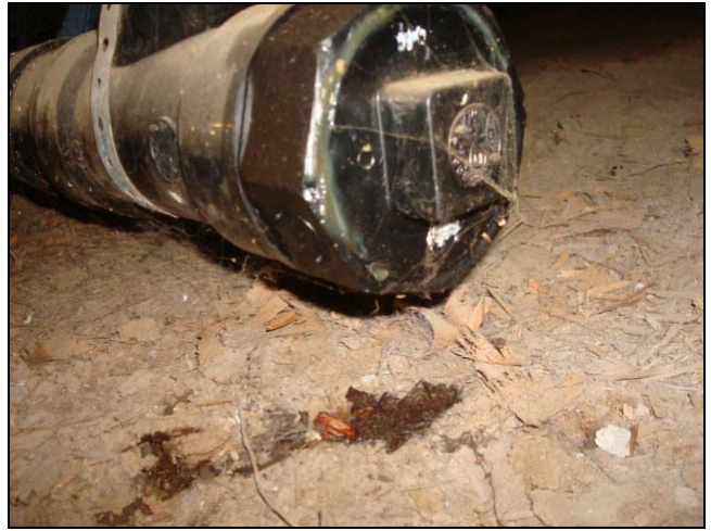
A water leak at a waste pipe cleanout cap.
