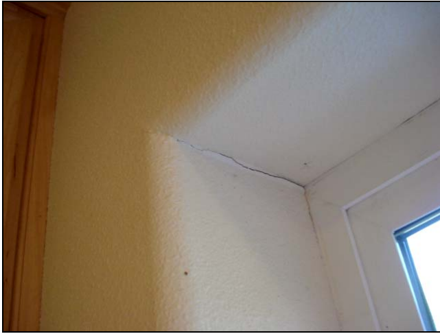
A common settlement crack.
