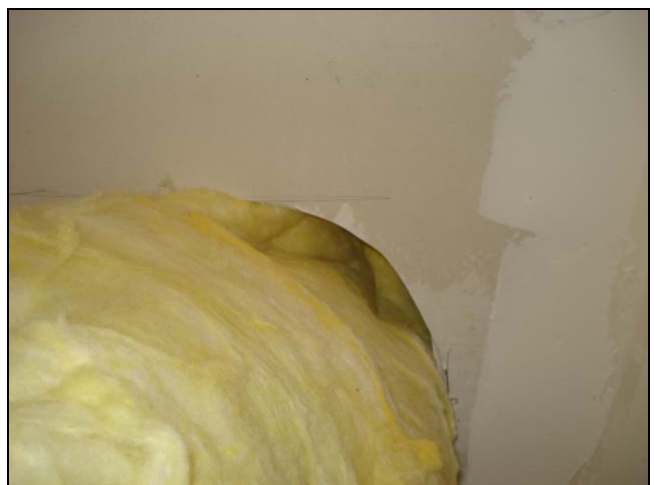
This heater ducting was not properly sealed.
