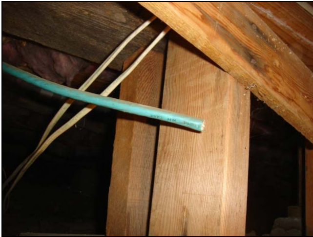
Is this open cable hot?
