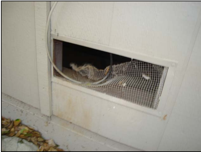
Damaged vent screen.
