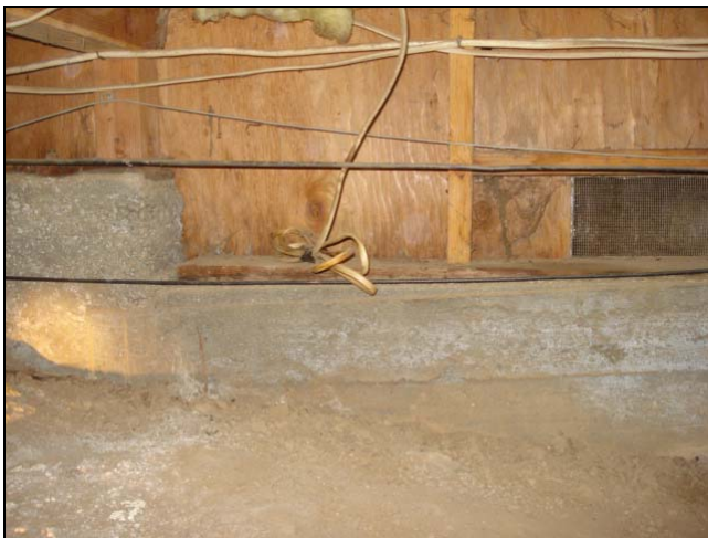
A loose wire.
