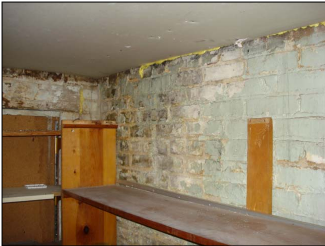
Stains and possible mold.
