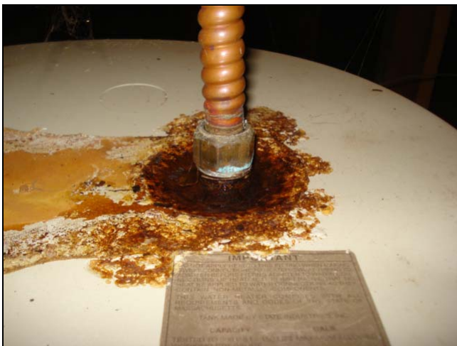
Nipple fitting leak.
