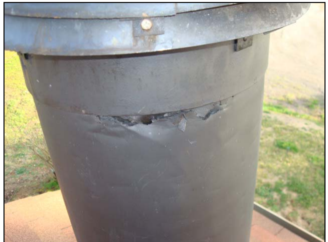
Deterioration in the flue pipe.
