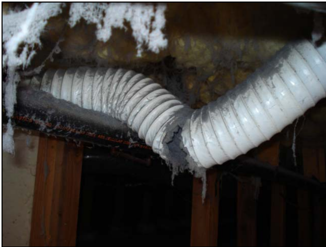
Damaged dryer vent pipe.
