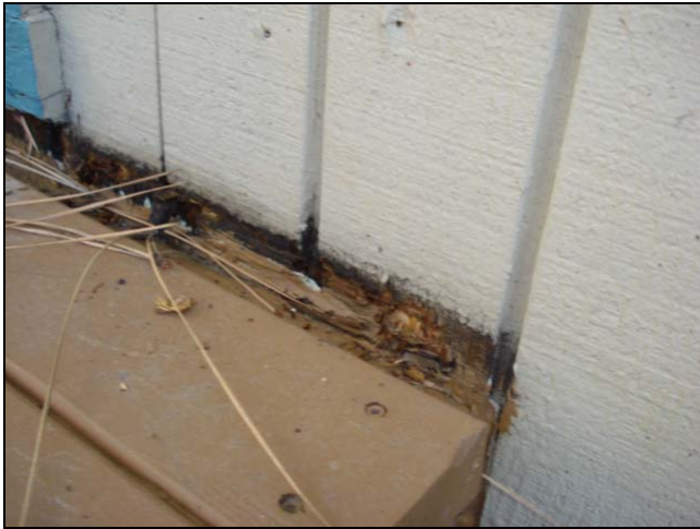
Deterioration between the decking and siding.
