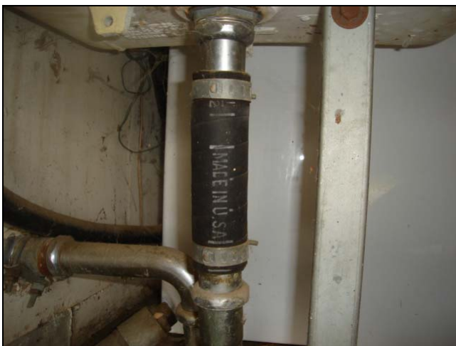
Automotive radiator pipes do not comply either.
