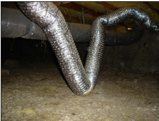
This vent pipe should run in a straight line. The saddle will collect lint. Ideally the pipe would have a smooth, continuous inner surface.
