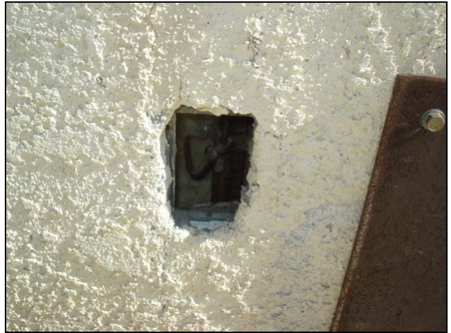
This hole should be plugged to prevent the entry of water, bugs and other unsavory things.
