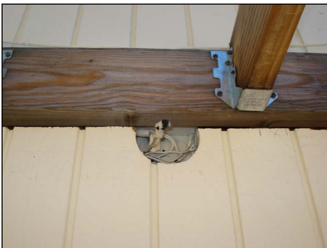
Blocked and open junction box. Not sure how to cover this one. Cut the plate in half?
