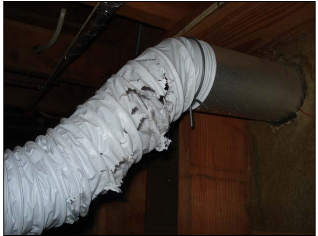
Damaged plastic dryer vent tube.
