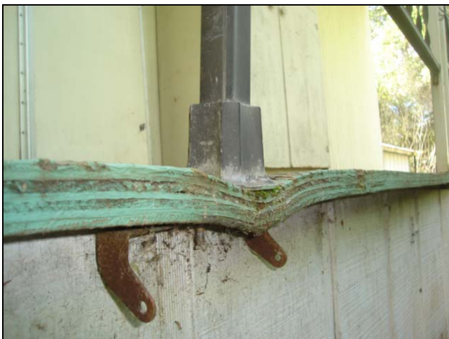
Deteriorated "Florida Room" porch on a manufactured home.
