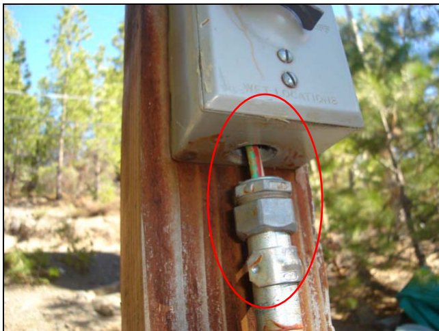
Loose conduit clamp at an exterior light switch.
