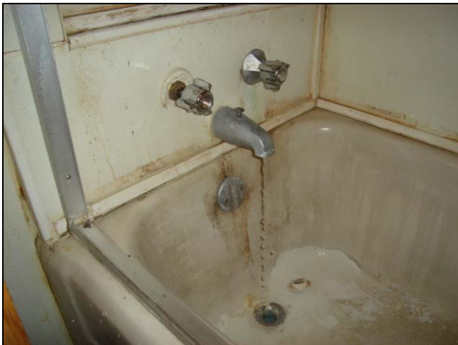
Leaking tub spout, and, eh, other stuff.
