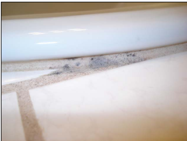
Possible organic growth in the basin grout.
