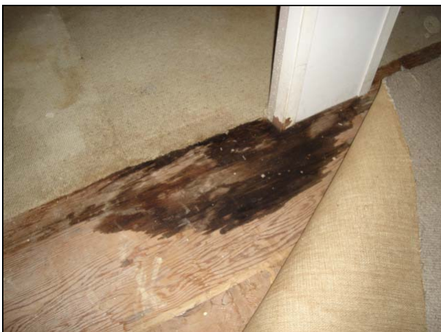
Water intrusion in a utility room.
