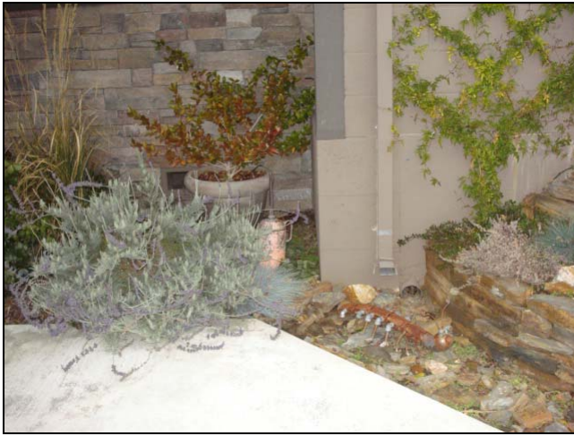
This downspout drains into a low area. No route was provided for water to evacuate.
