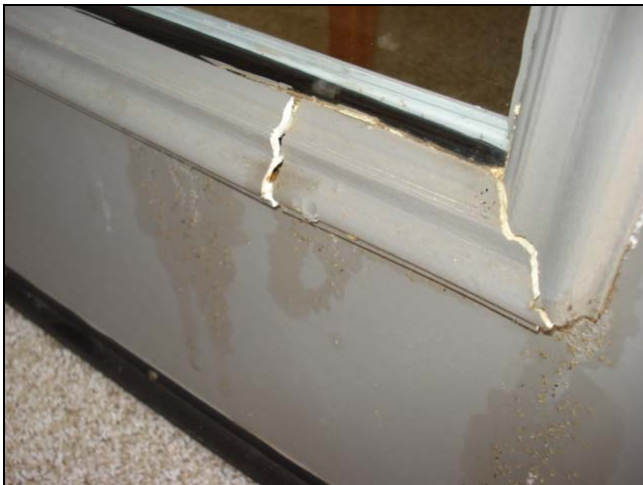
Cracked plastic window trim around the glazing in a full light "French" door.
