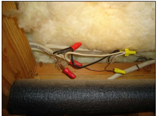
Another open splice.
