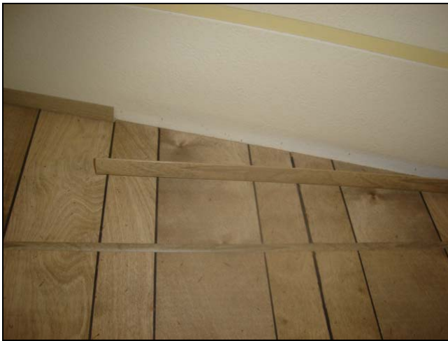
Loose crown molding wood trim.
