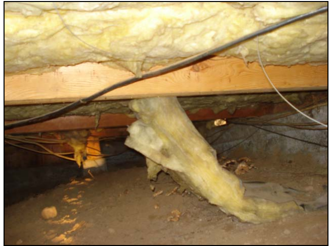
Loose fiberglass batting.
