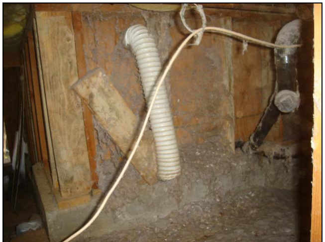
The dryer vent pipe terminates under the building.
