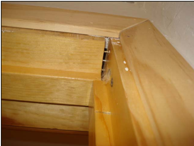
Jamb split open.
