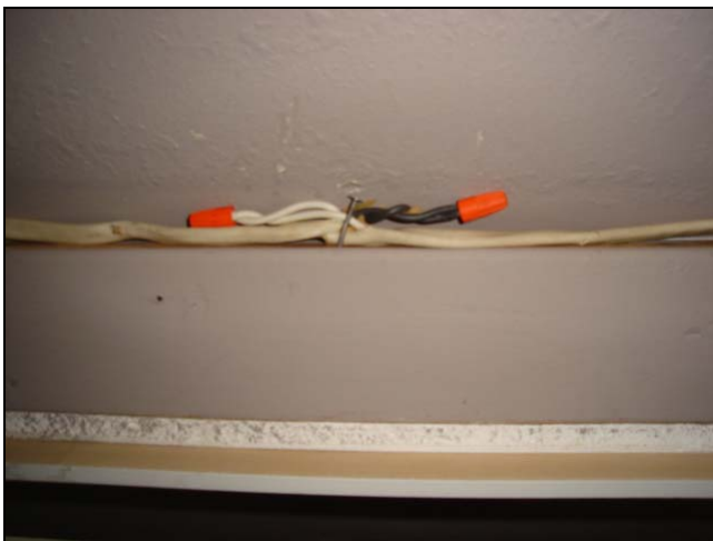
Open splice over a garage door.
