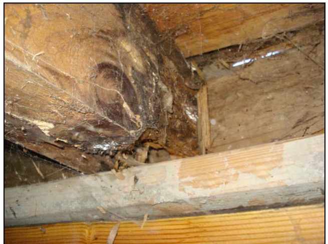
Severe deterioration in the beam.
