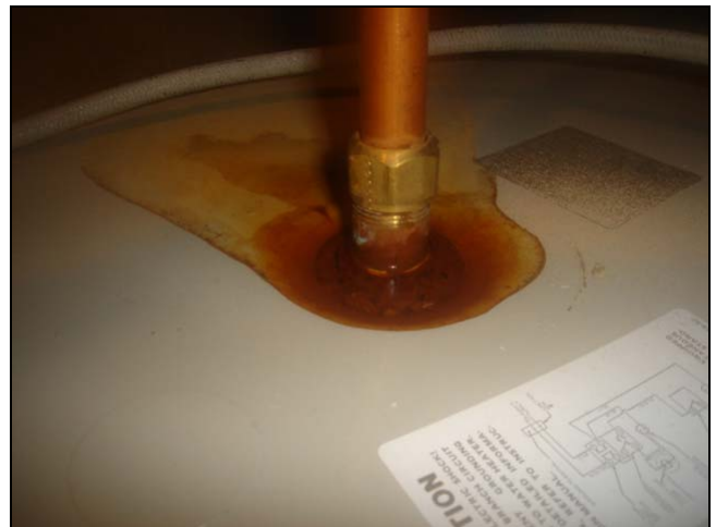
Severe water leak.
