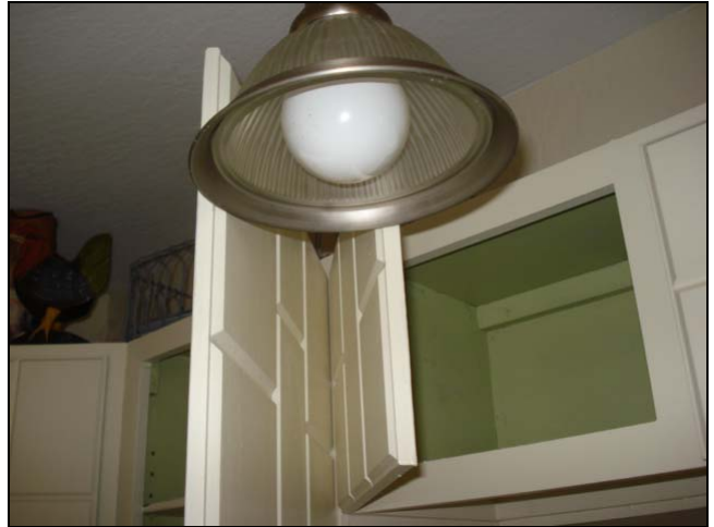
Two doors are hitting this light fixture.
