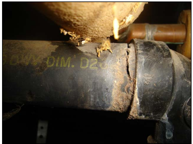
A cracked drainpipe.
