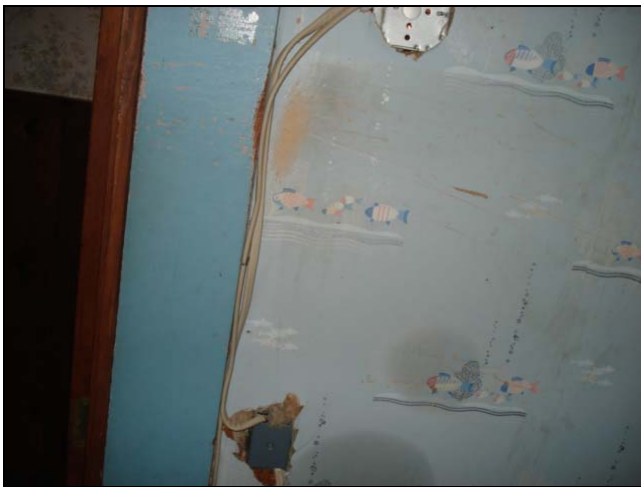
Exposed wiring in a closet of the kids room.
