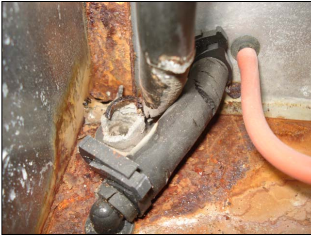
Corrosion and rust in the drip pan.
