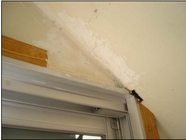
Patching over a patio door.
