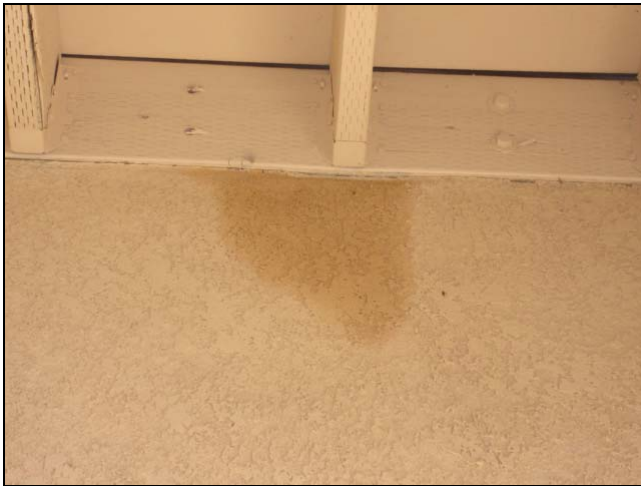
Stucco stain from an unknown source.
