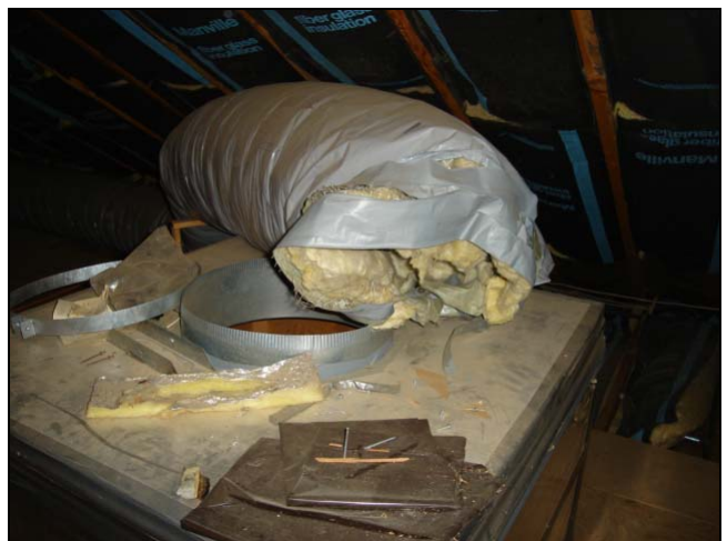
Loose HVAC ducting is a waste of energy.
