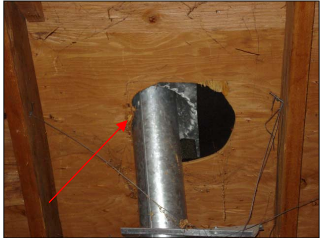
Insufficient clearance to flammable materials.
