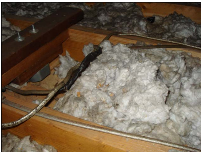
Open splices were allowed on knob and tube, but not here.
