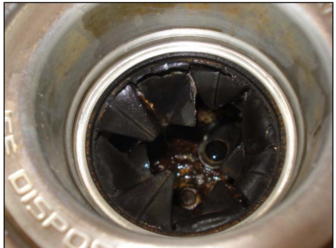
Damaged weir gasket.
