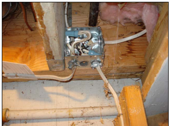
Missing cover plate.
