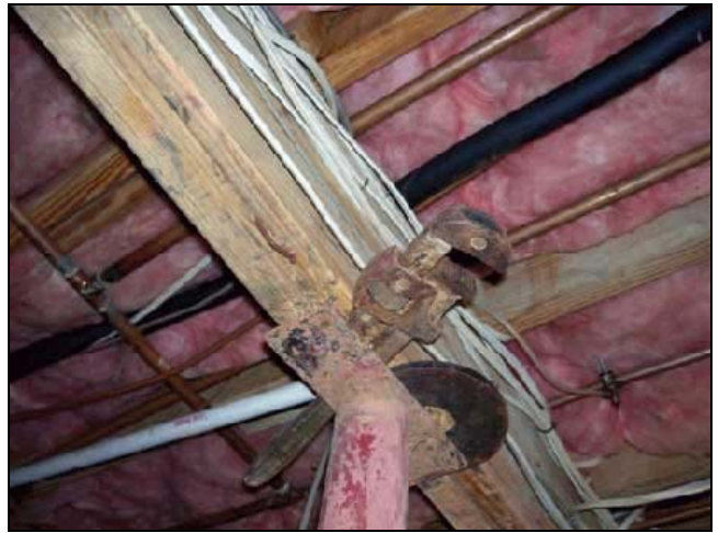
Monkey wrenches are not a proper shim.
