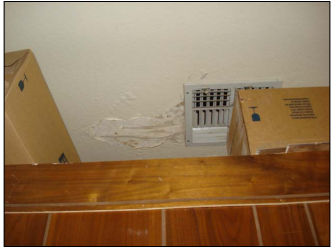
Peeling paint and water stains at a heater register.
