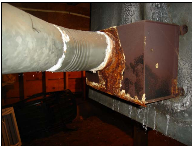
Rather severe corrosion.
