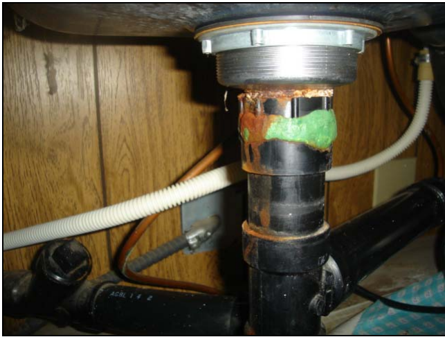
A leaking sink drain.
