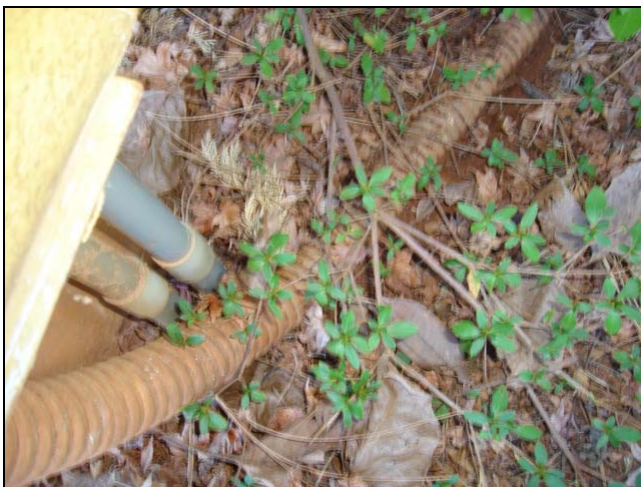
Metal conduit common around manufactured housing should be elevated above the soil.
