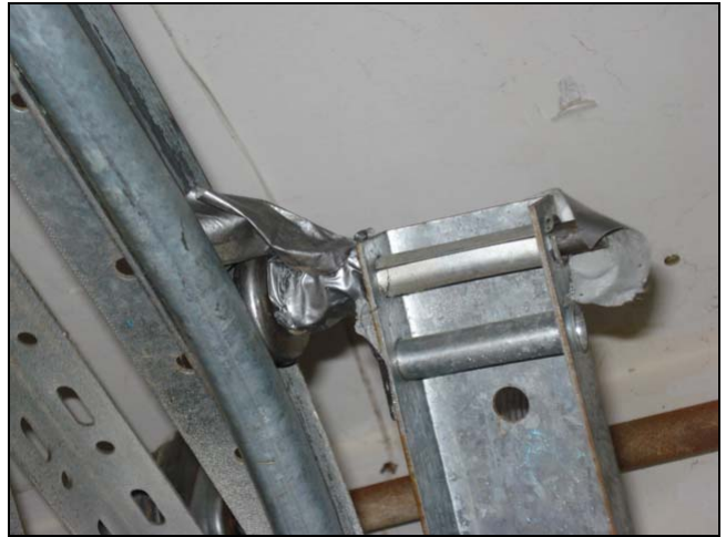
This roller refused to stay in the track. There may be a problem with the counterweight system.
