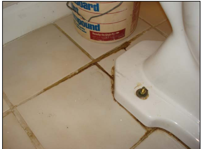
Appears to have a leaking wax seal. The toilet will have to be pulled and the sub floor needs to be checked.
