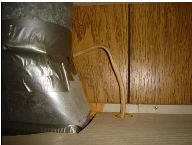
Exposed wiring in the cabinet over the stove exhaust fan. By the way, the vinyl duct tape is not the proper material for sealing a heated metal pipe.
