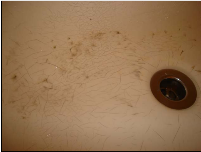
Hairline cracks in a fiberglass tub. They are surface cracks that do not penetrate or leak but are unsightly.
