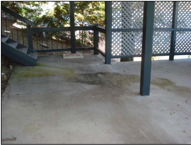
Water stains and green slime are a good indicator of water intrusion.
