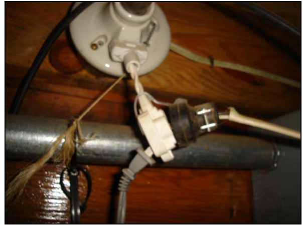
Let's see. Zip cords for permanent wiring, wiring being used as an extension cord, no ground for whatever this thing goes too. Fun.
