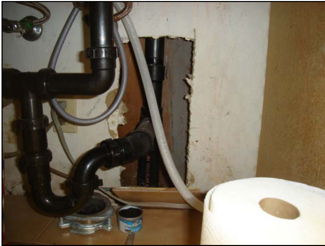
Cut out under a bathroom sink.
