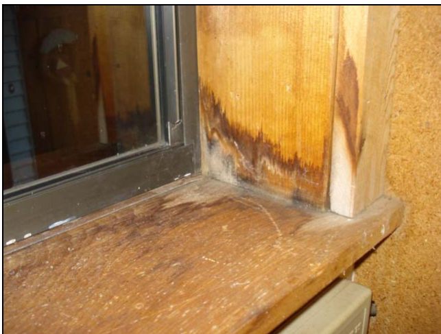
Water stain due to condensation.
