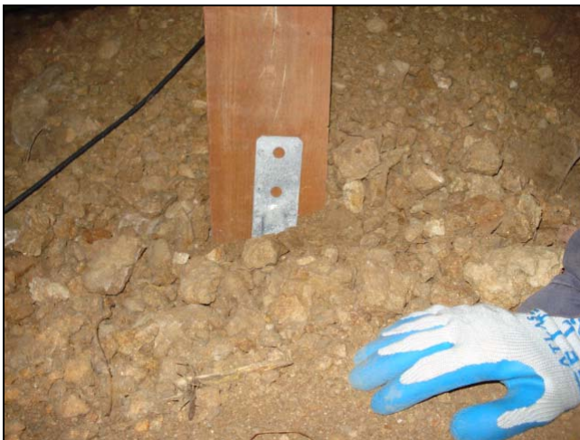
Wood to earth contact at a post. Where is the concrete pier? Buried in the dirt.
