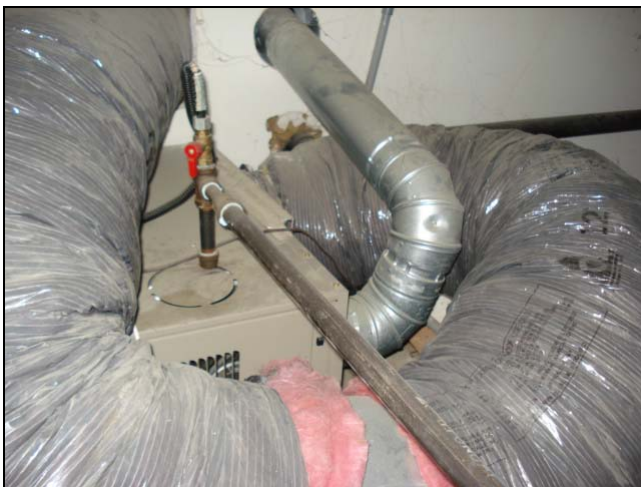
It won't be long before the hot flue pipe melts the ducting.
