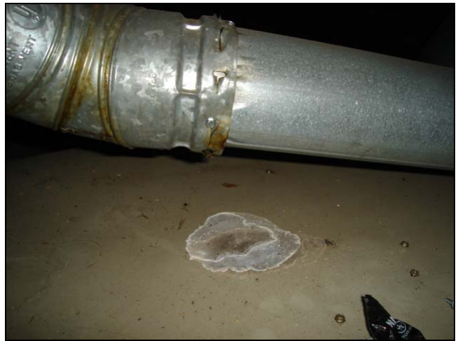
A condensate leak at a flue pipe.
