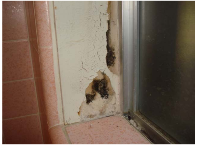
Organic growth and deterioration.
