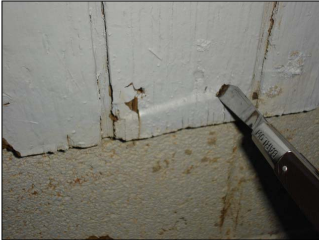
Deterioration in the T1-11.
