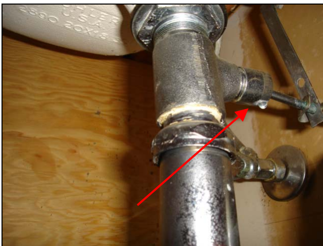
A leaking drain stopper control rod nut.
