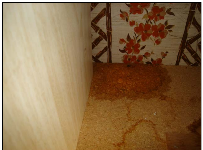
Water intrusion in a manufactured home closet.
