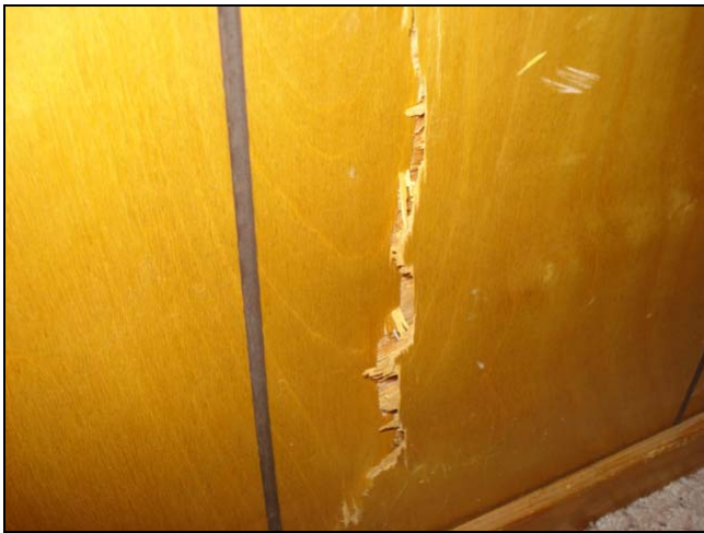
Cracked wood paneling.
