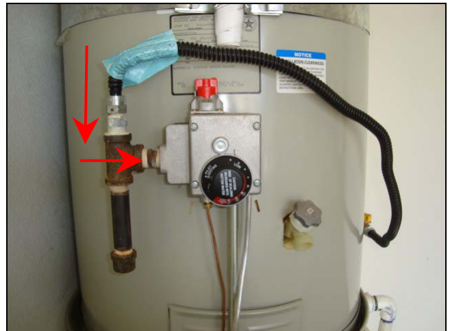
A proper installation. The gas changes direction.
