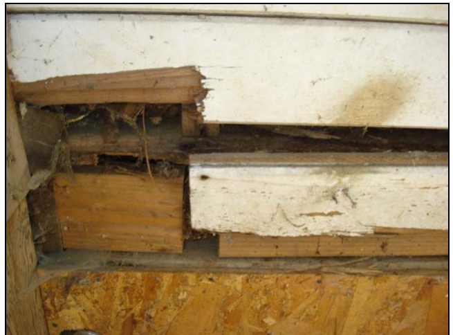
Advance stages of deterioration.
