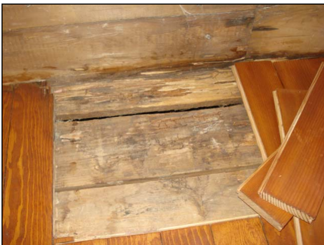
Damaged subfloor was being covered with new laminate wood floor. Opps.
