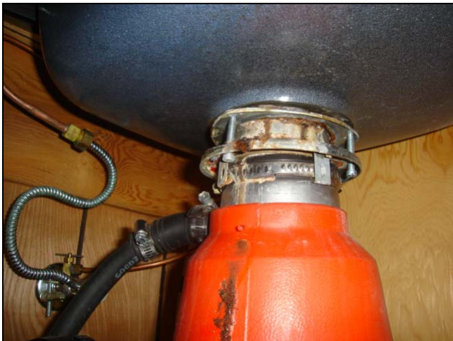
A loose garbage disposal connection.
