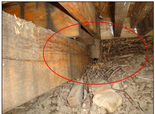
Wood to earth contact for these joists.
