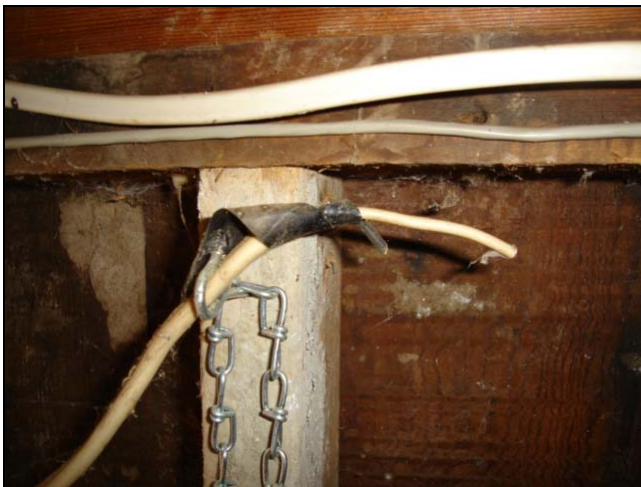
Is this open cable hot? Why is it just hanging there? What does it go to? If I have questions, so will the buyer.
