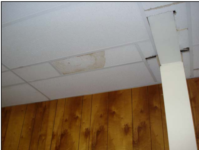
Water stain in a lower floor. This problem was from a sink leak in a room above.
