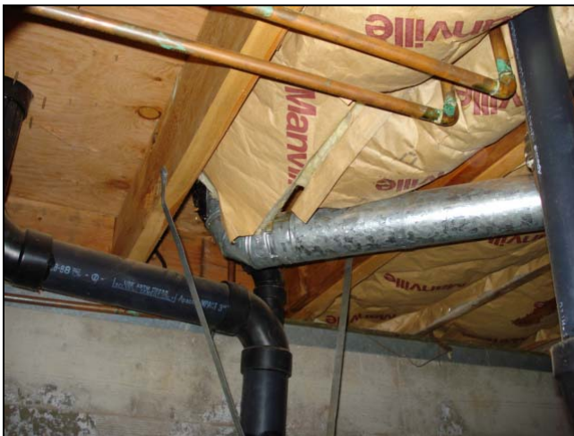
The insulation was installed upside down and in direct contact with the heater flue pipe.
