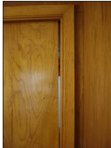
A pocket door that did not fully close at the top may need the track repaired.
