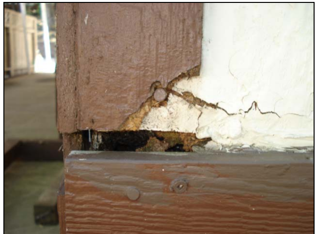
Severe deterioration in this hardbaord material. Notice the flat topped trim board.
