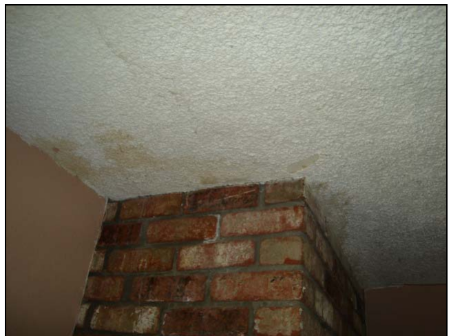
Stains around a fireplace usually indicated a problem with the flashing around the chimney.
