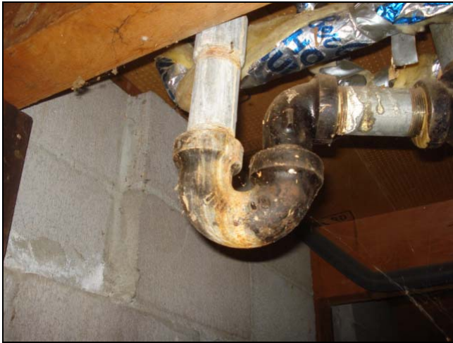
“P” traps under the building are for the tubs and showers. This one had a leak at one time. A little paint and this note goes away. Hint hint.
