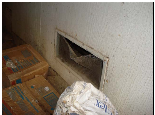
Damaged ventilation screen could allow for the entry of vermin into the crawl space.
