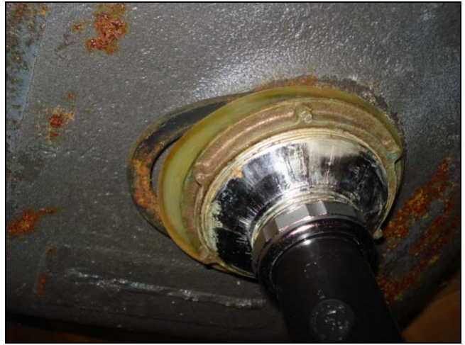
Slipped gasket on the sink connection. Rust on the steel sink bowl. Porcelain on steel sinks will eventually rust out.
