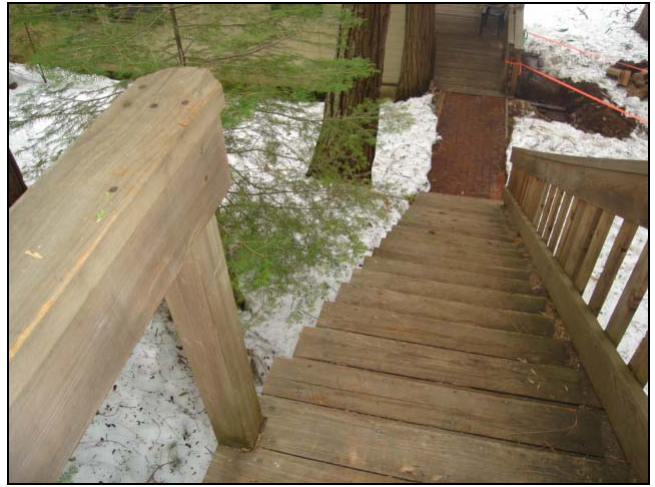
No guardrail. It could be argued that there is a railing on the right and the ground is not 30 inches down. At least a graspable rail ought to be installed. It's a gray area. Some inspectors will call it, others won't.
