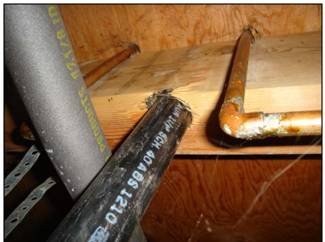
A very precise boring job by this plumber. This beam has lost over half its support capacity. This beam was under a bathtub. Bathtubs hold between 65 and 80 gallons of water. Water weighs 8.6 lbs per gallon. Do the math.
