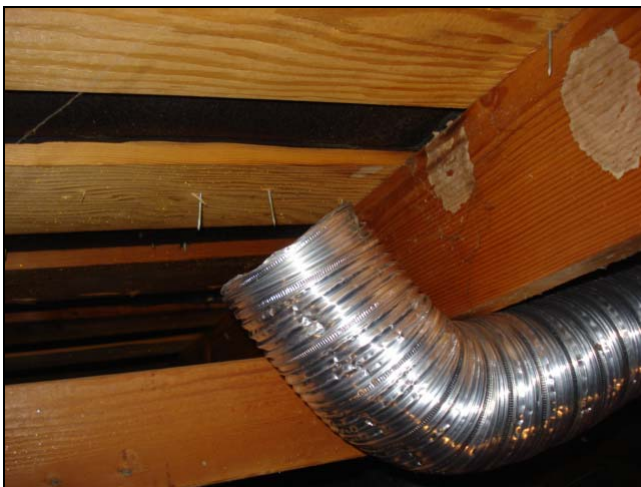
This vent blew right into the roof skip boards and felt paper.
