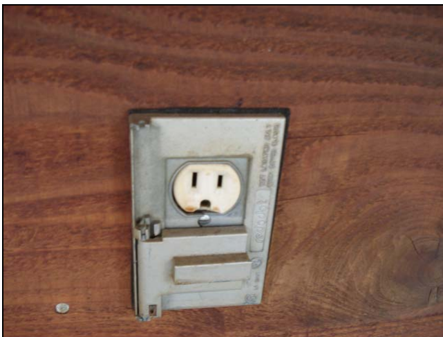
Defective weather cover.
