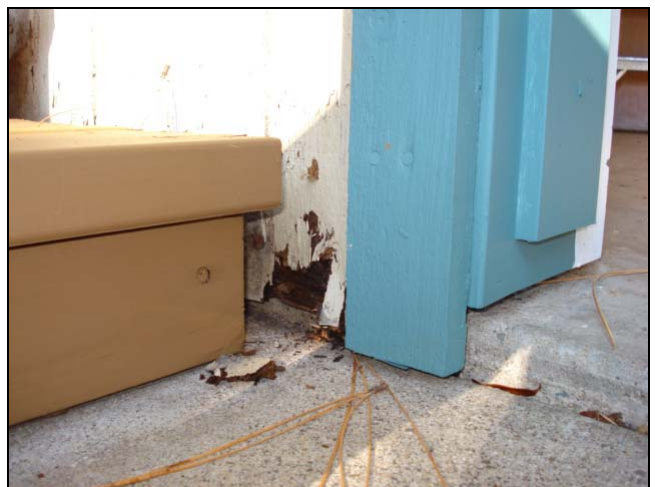
Deterioration in the T1-11.
