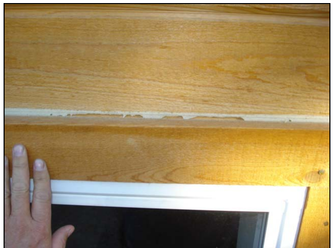
Another view. It is unknown if there was proper moisture wrap around these windows. After a few storms and we will know.
