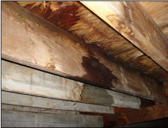
Severe water leak from above.
