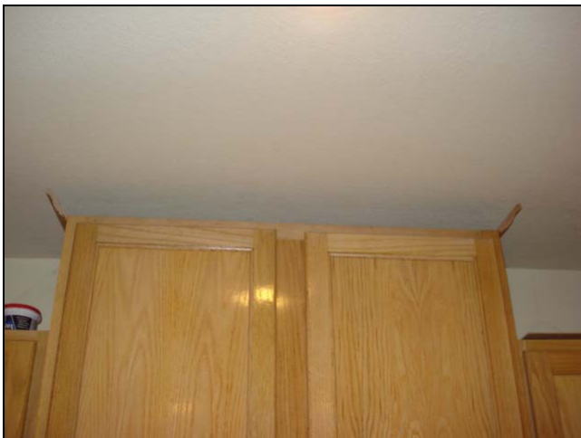
Missing crown molding.
