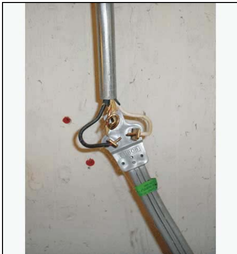
Homemade splice job for a 220-volt cord.
