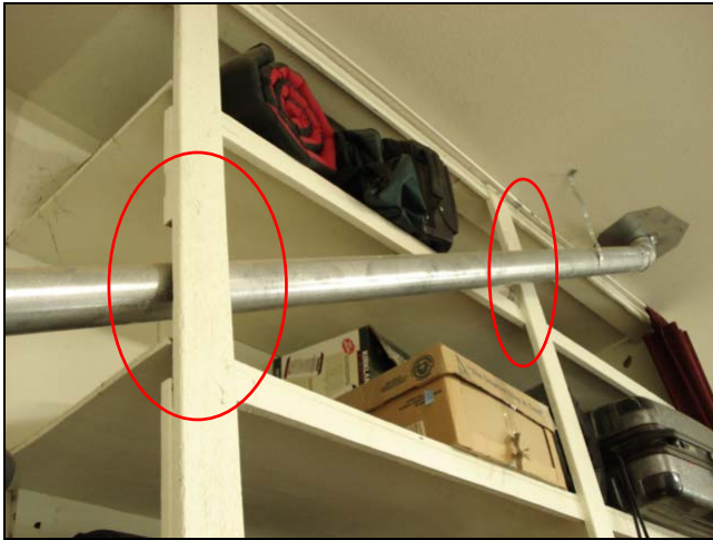
Insufficient clearance to flammable materials.
