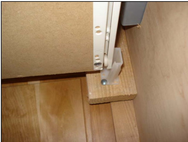
This track was off the guide.
