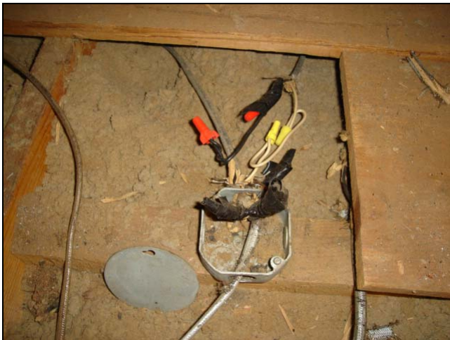
Open junction box and open splices.
