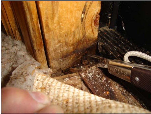
Deterioration in the jamb under the carpet.
