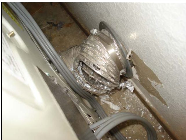
Damaged vent pipe.
