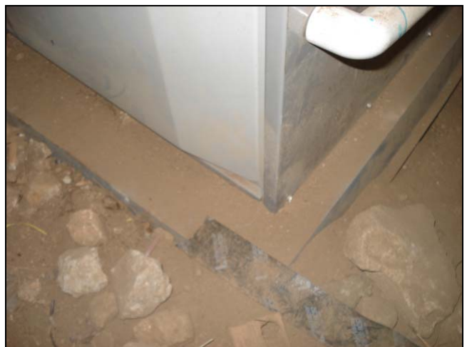
Dirt around the furnace housing.
