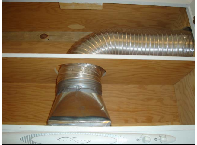
Corrugated vent pipe.
