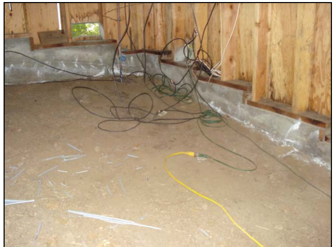
Here is a look from the other side of the vent.
