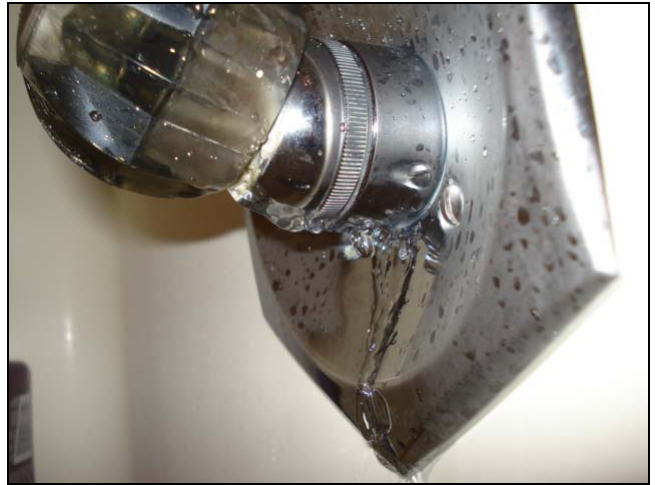
Leaking shower control valve.
