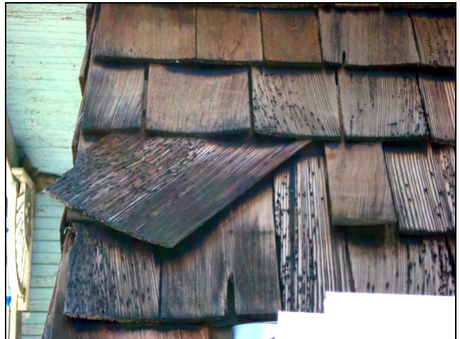
A slipped wood shingle.
