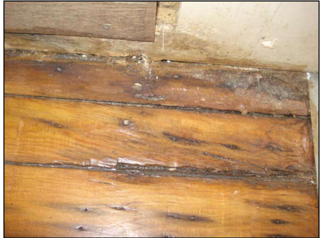
Old water stains at a patio door.
