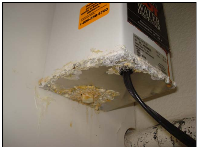
Corrosion under this instant hot water dispenser.
