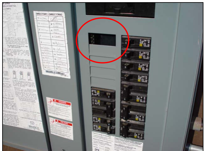
All open blanks should be plugged.
