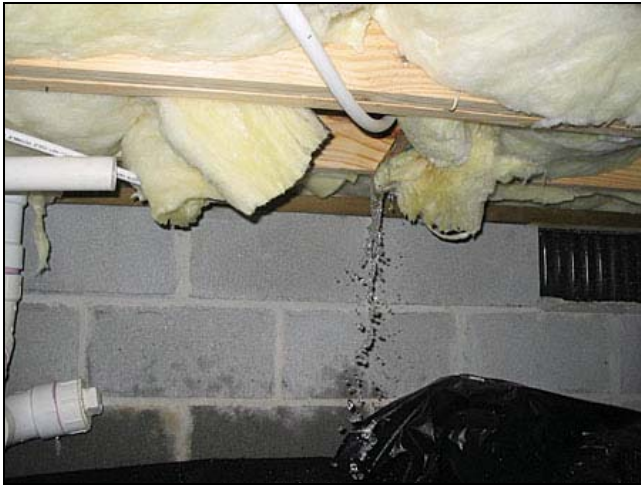
A leaking water supply line.
