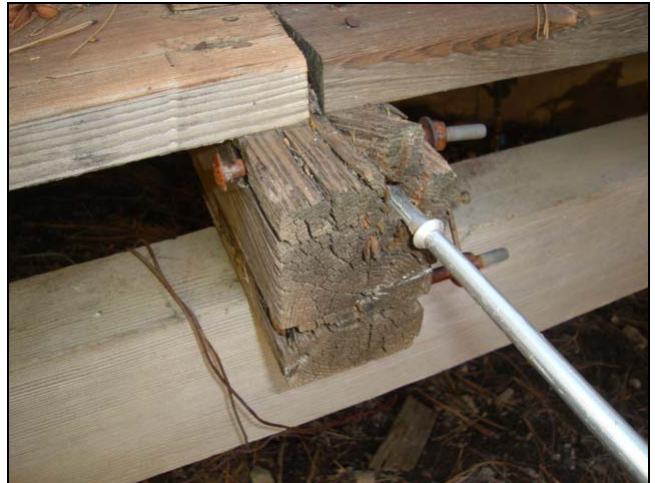
Decay in a beam.
