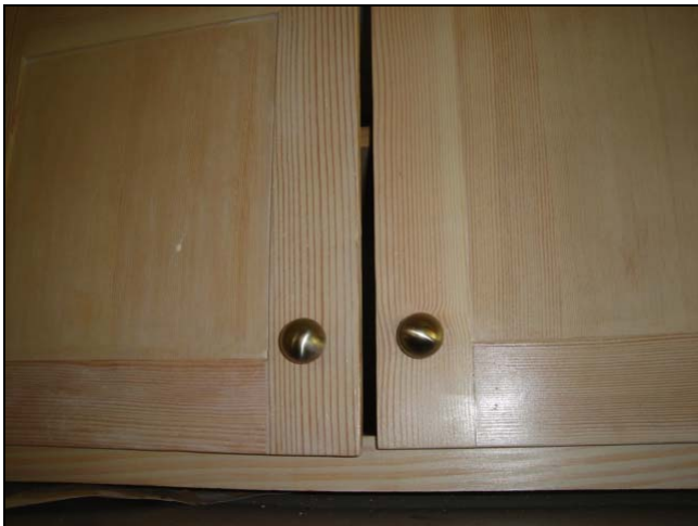
The doors were poorly fit.
