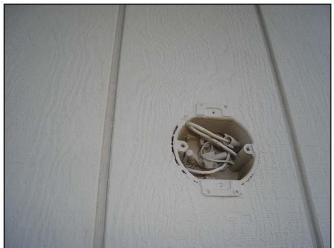
Open junction box.
