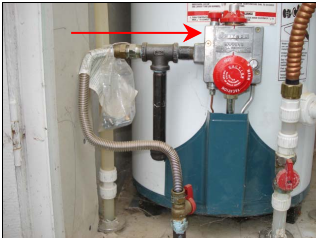
Improper drip leg installation.
