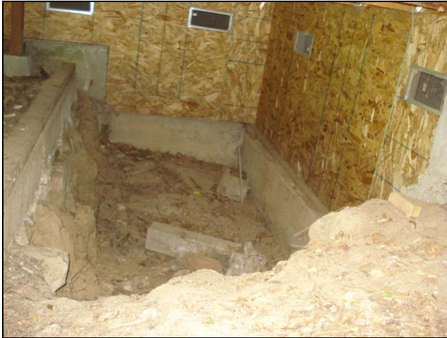
This pit under a deck will be a become a pool in wet weather. Water could rise as high as the OSB siding materials and cause serious damage.
