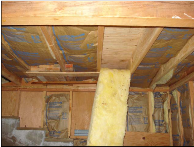
Loose insulation fiberglass batting. The insulation was installed upside down. The vapor barrier (kraft paper coating) should face towards the living space above.
