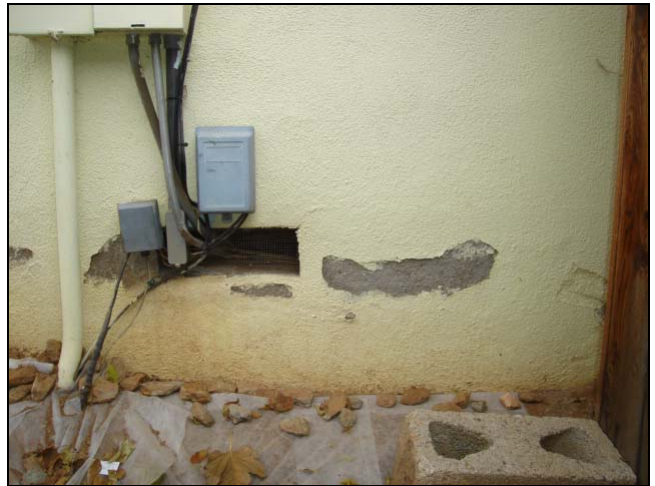
Peeling and flaking stucco and paint. That vent screen should be repaired also.
