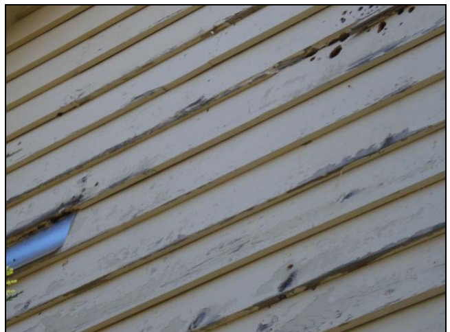
Peeling paint on this metal siding.
