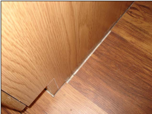
Flooring material shorted at a cabinet. A piece of trim could have solved this.
