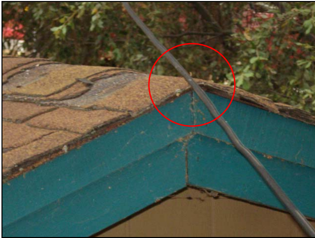
This wire was indirect contact with the coarse shingles of this garage roof. Lookslike the roof needs attention as well.
