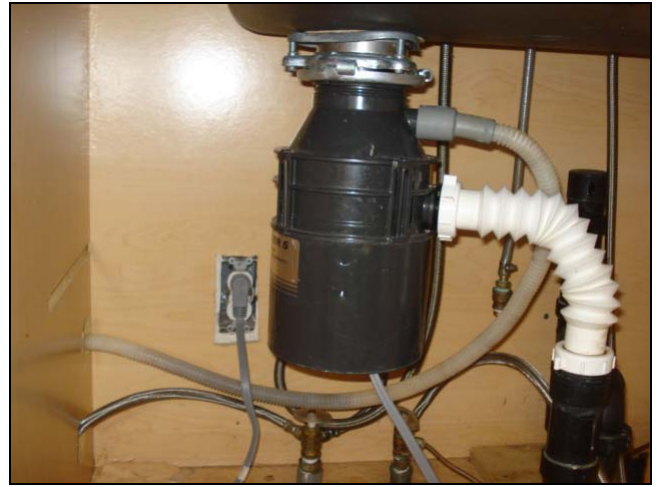
This corrugated material comes in all sizes. Do you think waste from the disposal will eventually clog this pipe? The dishwasher drain pipe did not have an airgap or high loop. Do you see a 3 rd issue? Think electrical.
