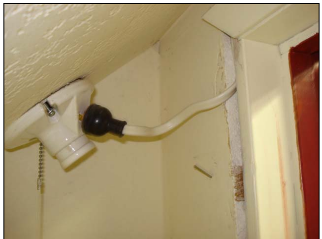
Electrical wiring being used as an extension cord. Probably shouldn't run through a door jamb either.
