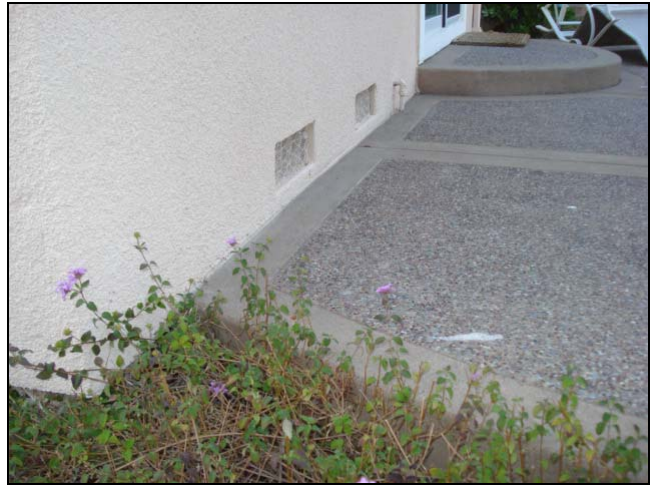
The weep screed is sealed in concrete at the bottom of this wall.
