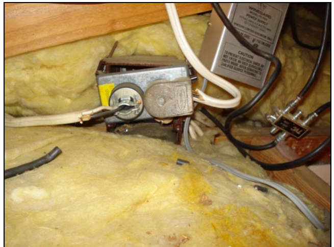
Is there an exception for using non-metallic sheathed wire as an extension cord in an attic? NO.
