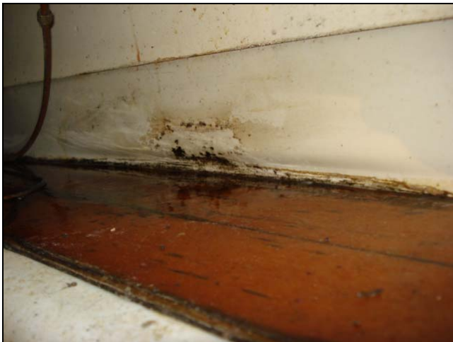
Standing water and organic growth in a baseboard.
