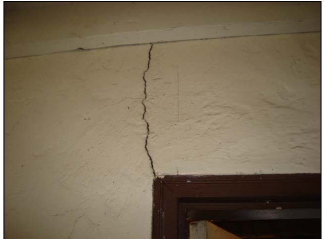
A stress crack.
