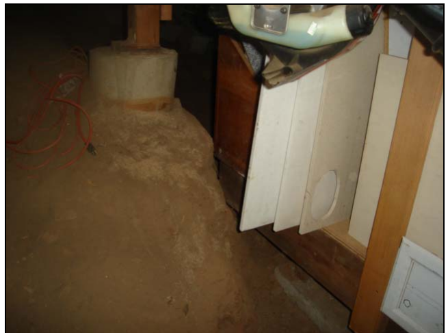
Excessive soil excavation. Wood to earth contact at the platform joist.
