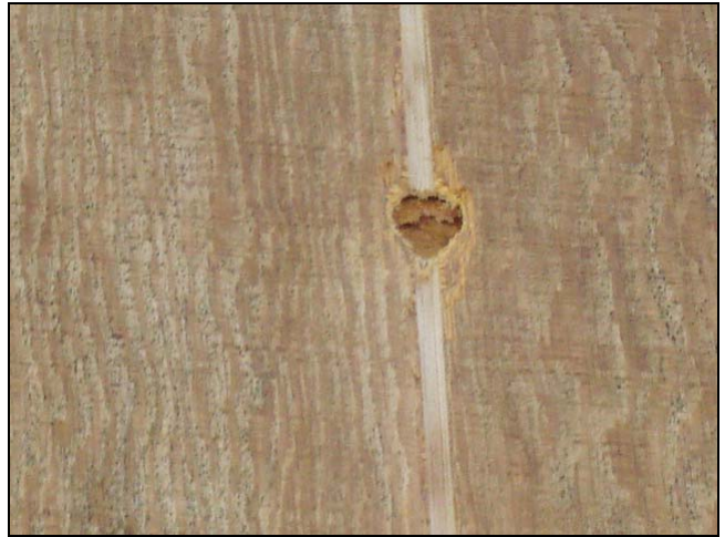
Wood pecker damage.
