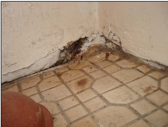
Deterioration in a bathroom.
