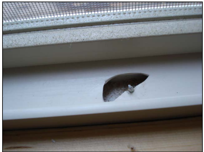
Installation error. Notice the nail sticking up from below. Why did the installer force the window in this hole without bending down the nail first???
