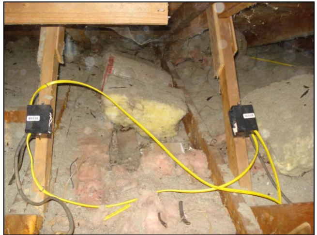
Open junction boxes.
