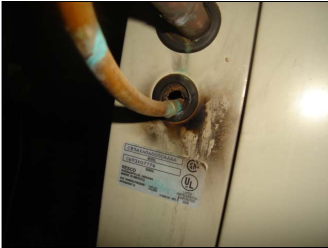
Air leaks around the A/C line grommets were common.
