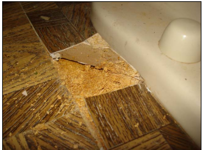
Deterioration in the vinyl and underlayment at a toilet.
