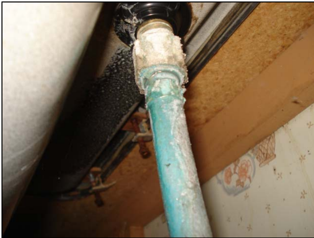
A leaking water supply line.
