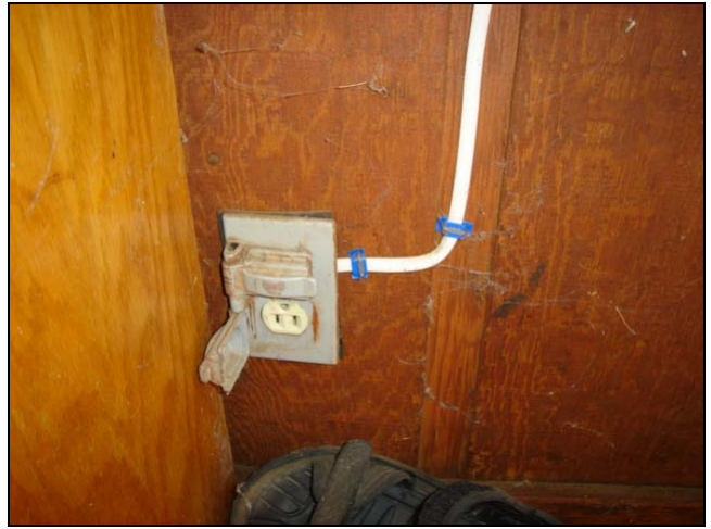
More exposed wiring.
