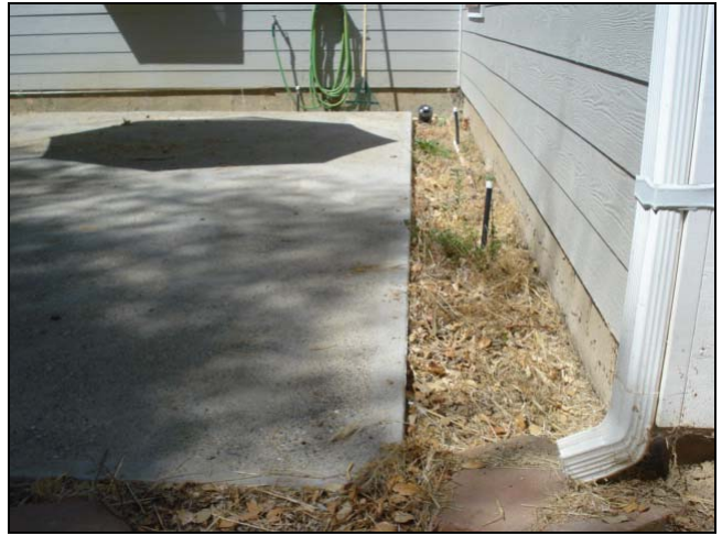
There was nowhere for water escape from around this patio.
