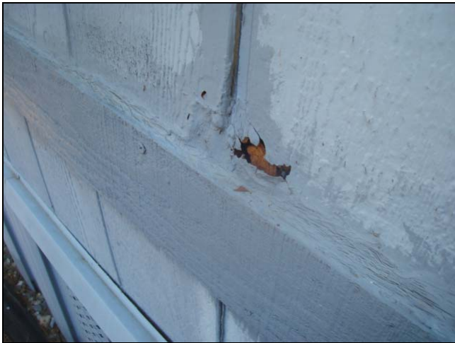
Hardboard deterioration. Notice the flat topped trim board.
