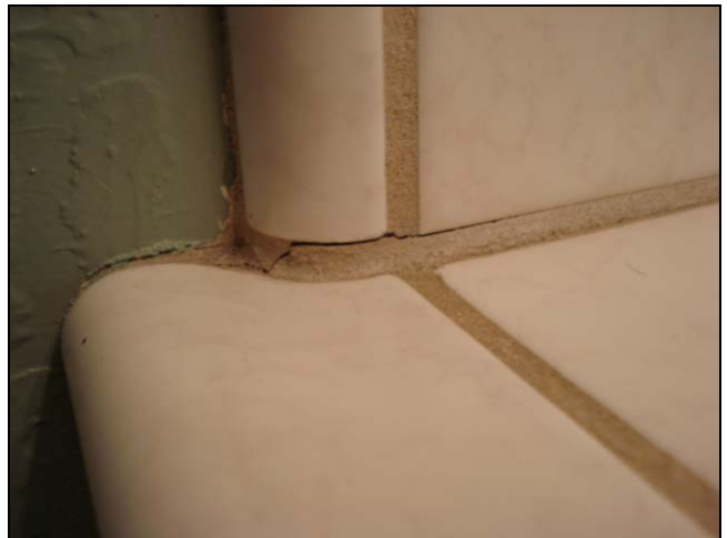
Cracked grout at a side splash.
