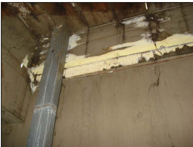
Possible fungus between the decking material and the siding.
