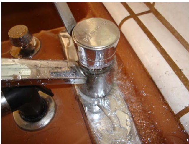
A leaking control lever.
