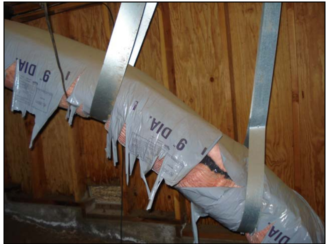
Shredded duct cover.
