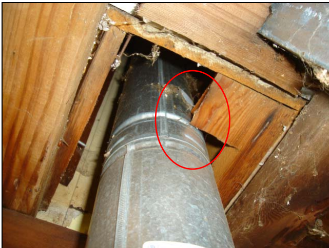
Insufficient clearance to flammable materials.
