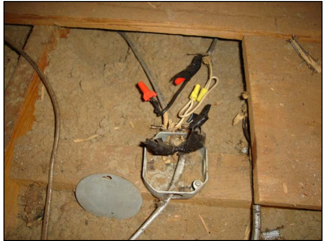
These splices didn't quite reach the box.
