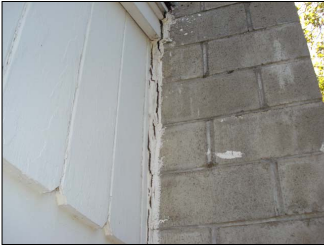
This chimney is pulling loose from the wall.
