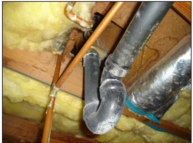
Some black spray paint on a repaired plumbing pipe might help lower the impact of the report. Just a thought.
