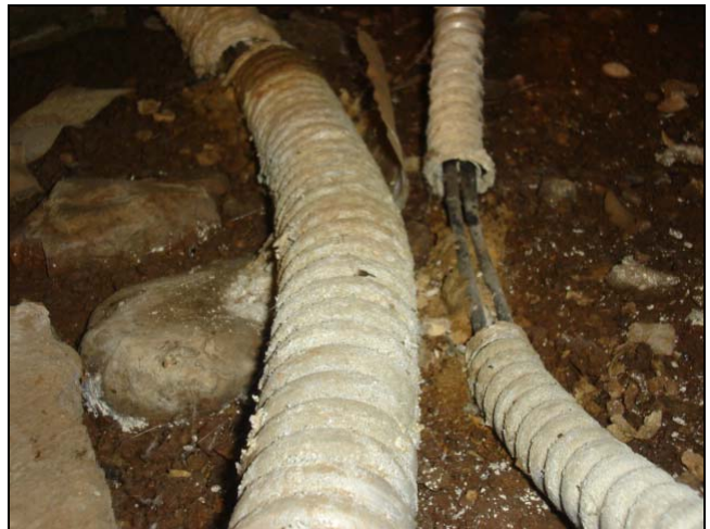
This metal conduit has completely deteriorated. The wiring inside is exposed to the elements.
