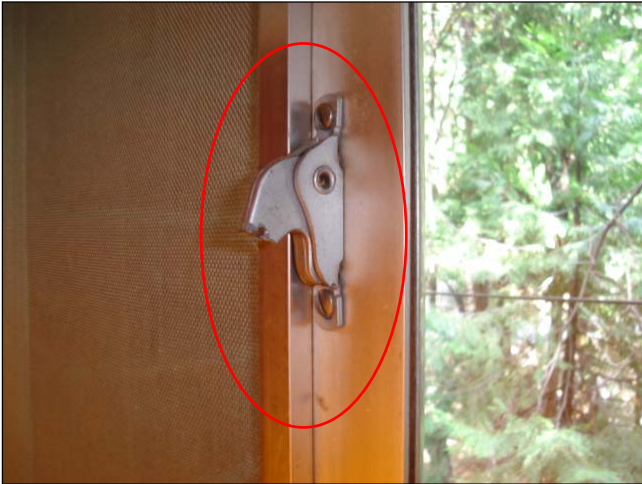
Broken latch. Hard to unlock if an individual needs to exit in a hurry.
