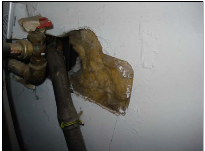
Hole in the wall behind the washer in a garage. These will be discussed in greater detail in the chapter on garages.
