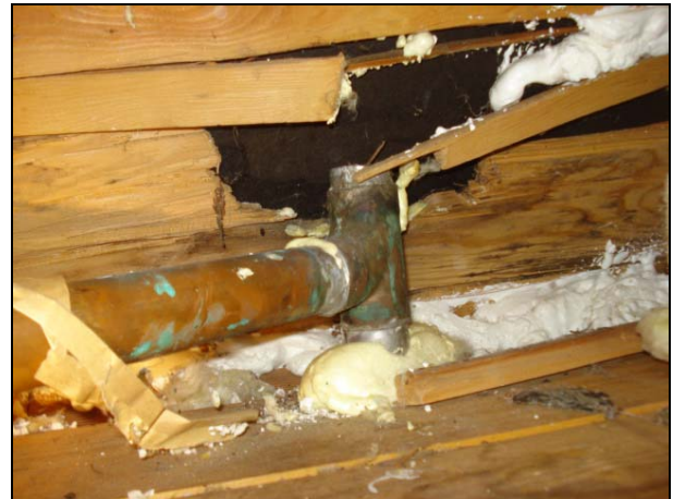
When the new roof was installed, this plumbing vent pipe was forgotten. Septic gasses were allowed to vent into the side attic access space of this "A" frame cabin.
