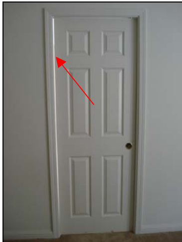
A pocket door reveal exposed at the inside edge. The frame must be oversized as compared to the door. The door did not fully fill the doorway.
