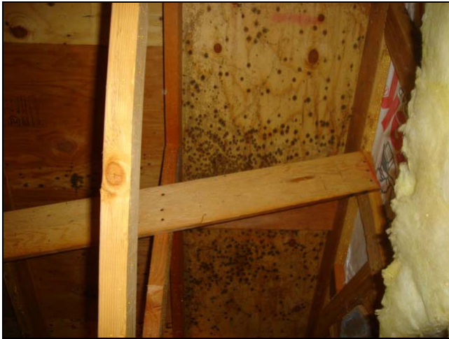
The black sploching is the wood mold that probably was dormant in the plywood sheathing materials. Poor attic ventilation will allow a build up of moisture in the attic space. Moisture that is not vented will activate the wood mold spors.
