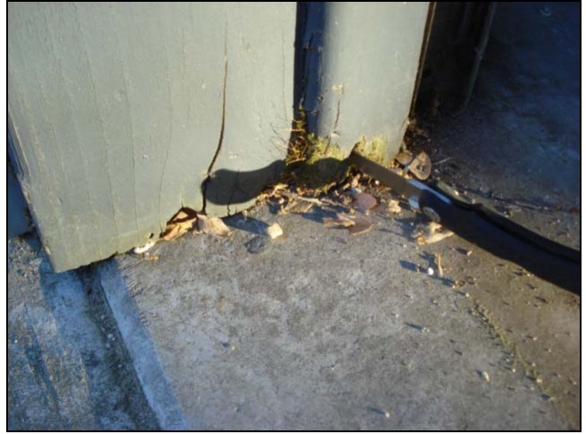
This type of deterioration is common at the base of the big door's side trim.
