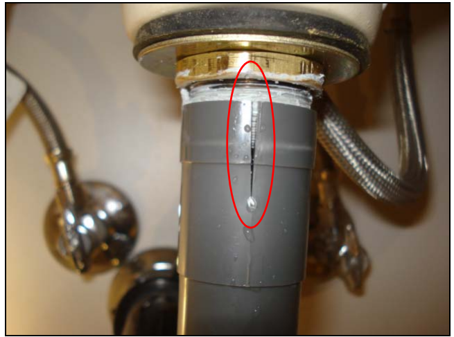
A cracked sink tailpipe and missing collar nut.
