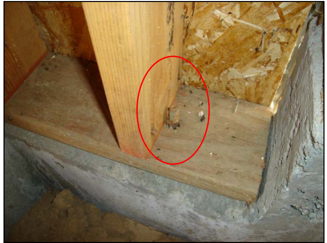
Missing anchor nut and washer.
