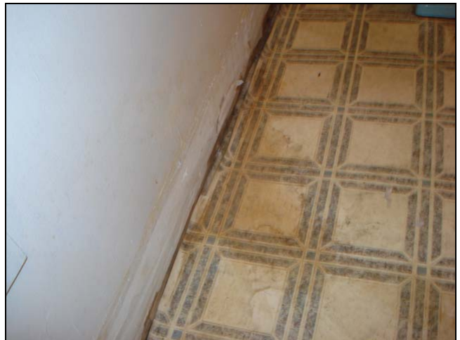
Discoloration and evidence of water intrusion.
