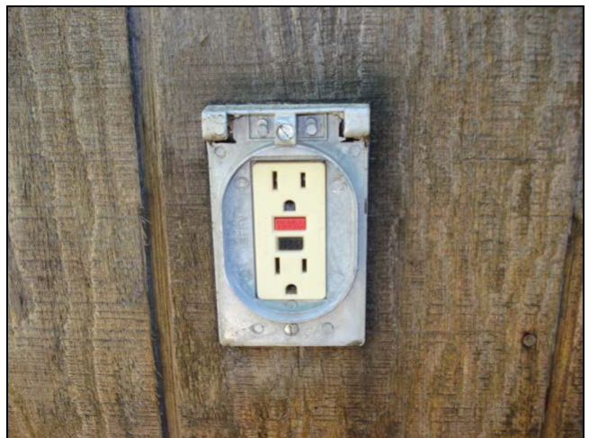
Missing weather cover for a G.F.C.I. outlet.
