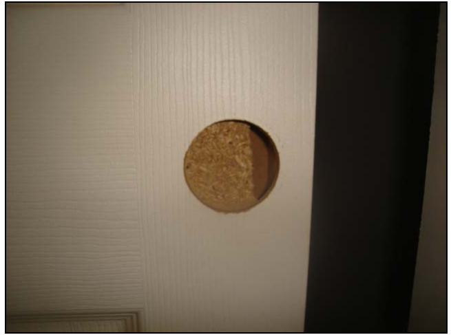
Missing finger pull on this closet door.
