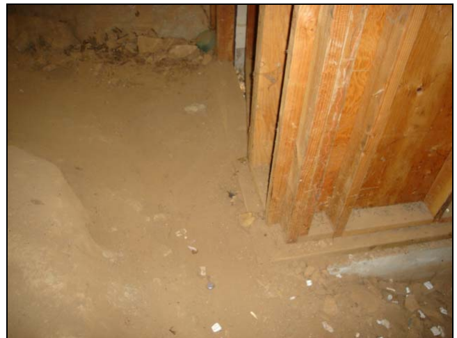
Wood to earth contact at this room addition.
