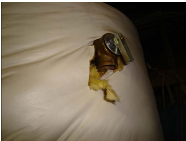
TPR valve with no pipe.
