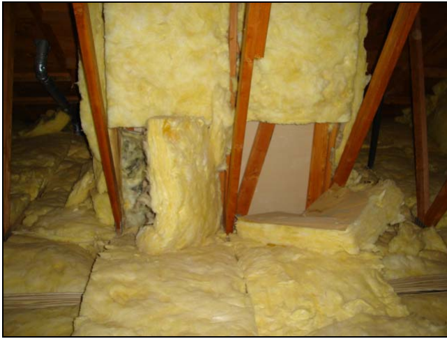
Loose batting on a channeled skylight housing.
