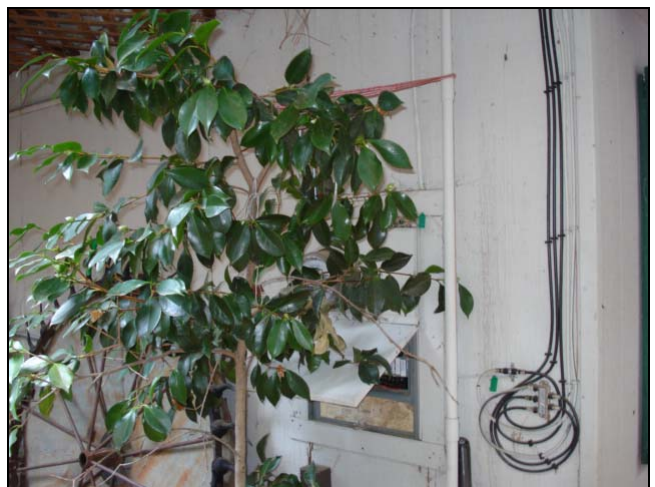
The tree prevents proper access.
