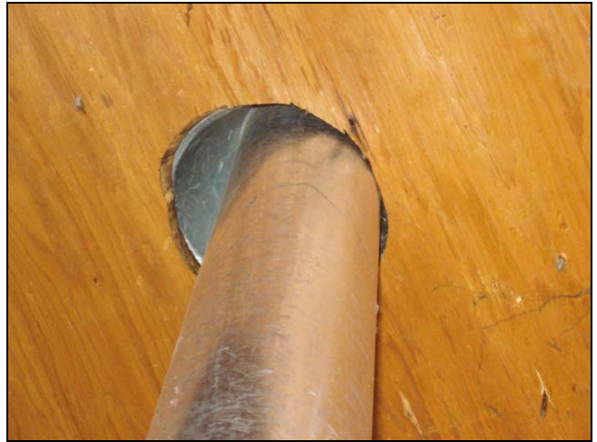
Insufficient clearance to flammable materials.
