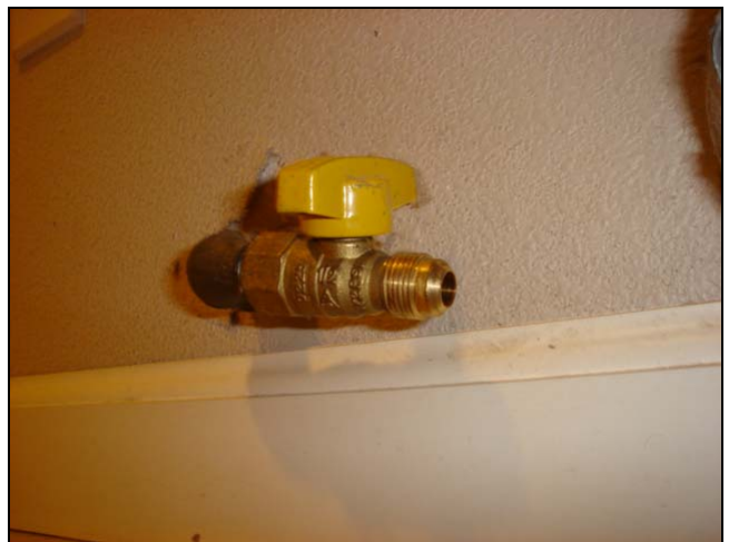
Missing gas valve cap.
