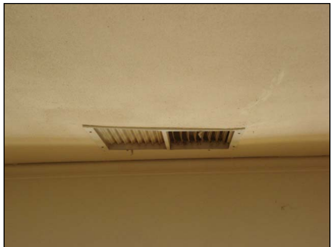
Sagging ceiling material.
