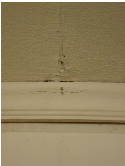
Patching, cracks, rusting nails and organic growth.
