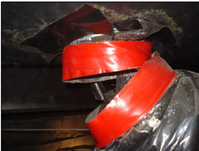
A loose duct.
