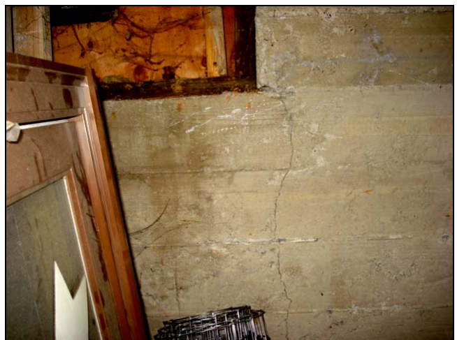
Foundation crack. Appears to be stable.
