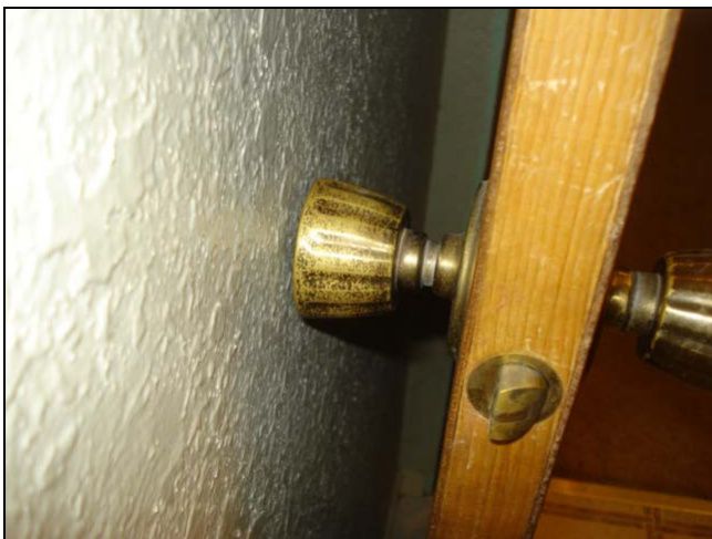
No doorstopper. The knob hits the wall.
