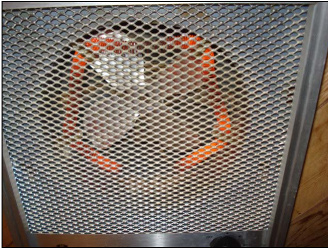
This electric bathroom heater worked but the blower fan didn't.
