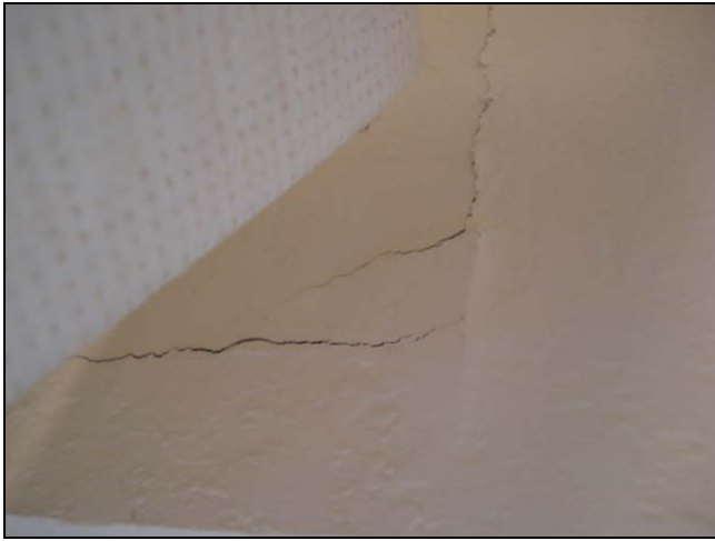
A classic stress crack.
