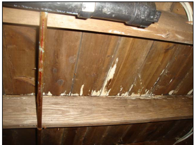
“Possible” fungus growing in the sub flooring.
