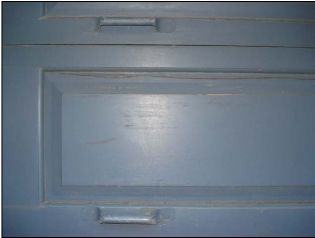
These wood panels were cracked.
