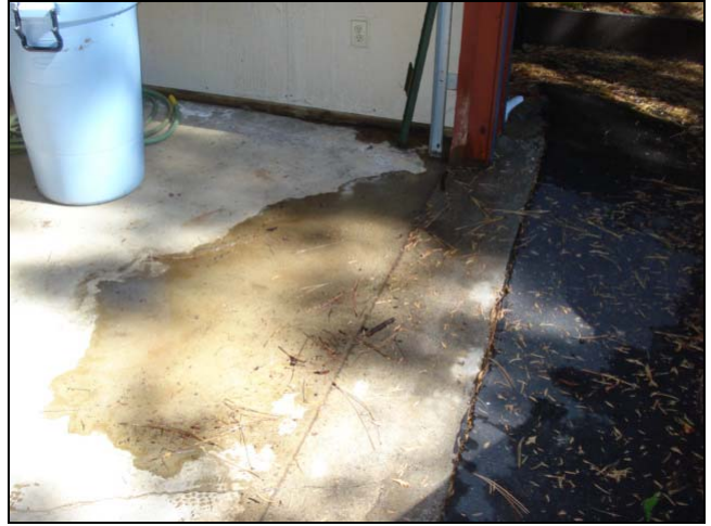
Water intrusion under a garage door.
