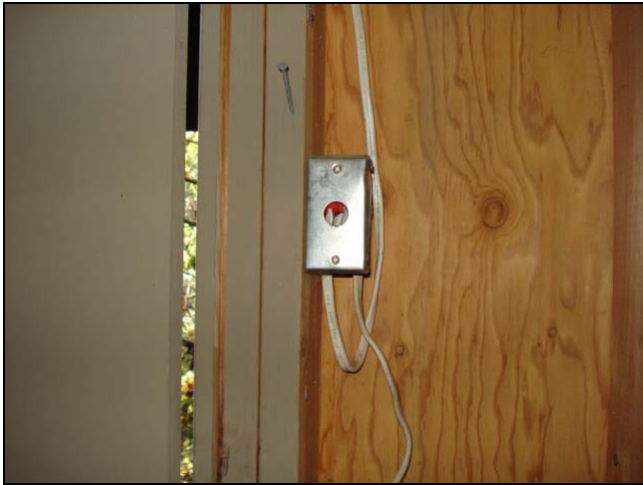
The all too common exposed wiring.
