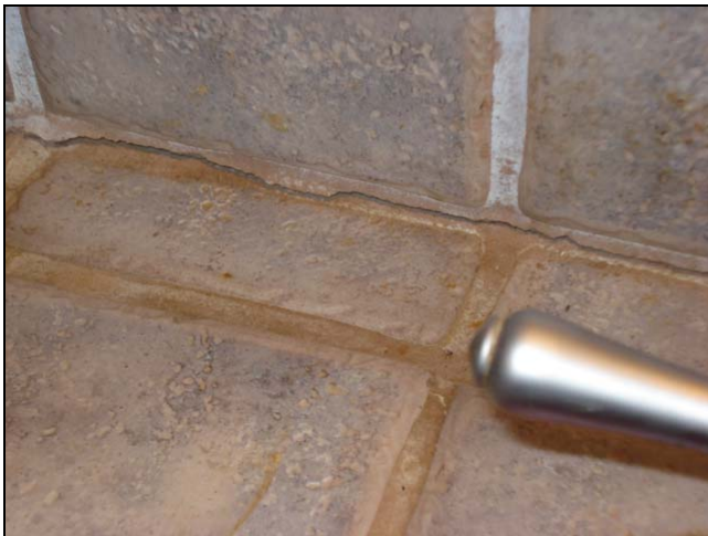
Cracked grout at a backsplash.
