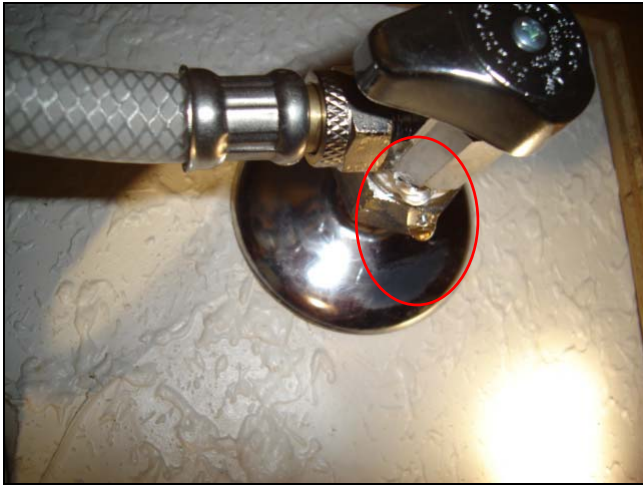
A leaking angle stop valve.
