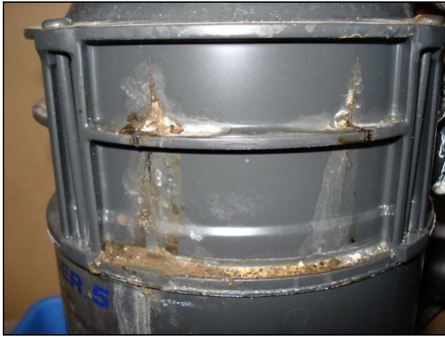
Leaking garbage disposal casing.
