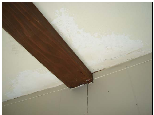
Patching after a water leak repair.
