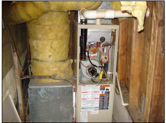
This high efficiency system looked good but for the lack of a gas drip leg.
