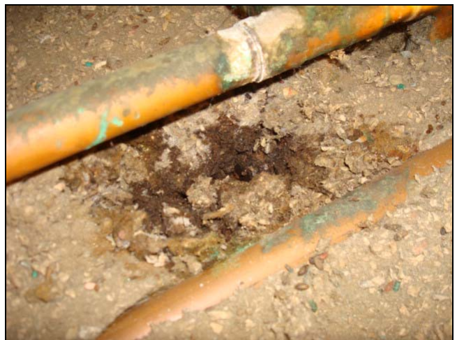
Leaking copper water pipe. Water pipes in attics are common in homes with a slab foundation.
