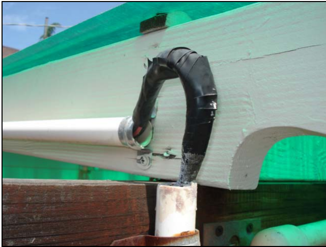
The conduit will eventually fill up with water. A junction box needs to be installed here.
