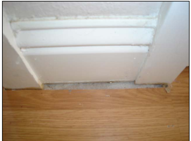
Flooring shorted at a closet door. Do it yourself job that wasn't quite done.
