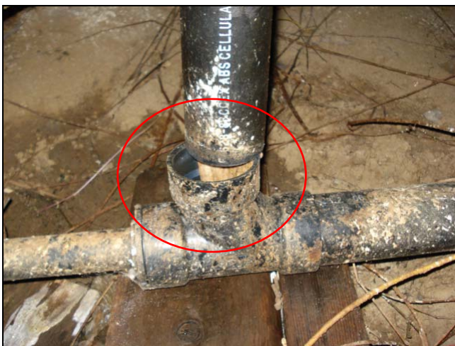
A loose waste pipe downstream from a toilet. This is a HAZARD for inspectors and occupants.
