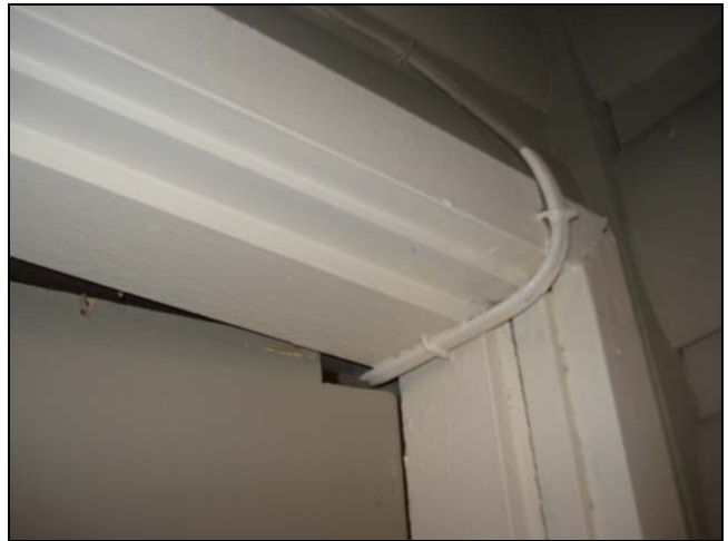
The exterior door was notched to provide a clear path for this exposed wiring to exit the building.
