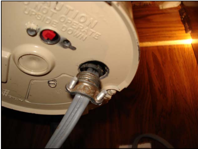
Loose clamp at the base of the garbage disposal. More about this in a coming chapter.
