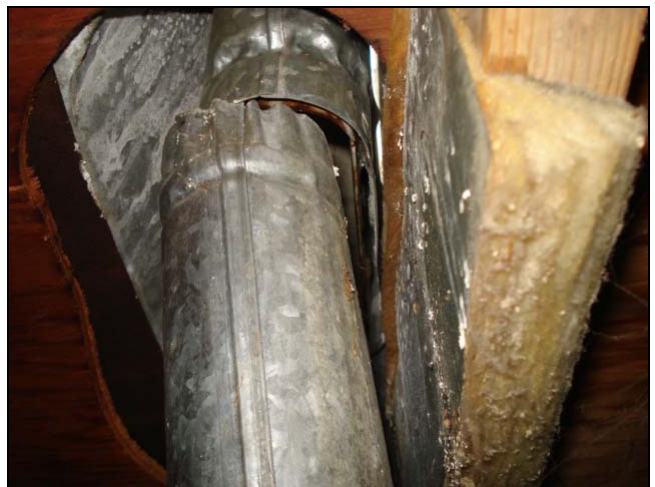
This loose stove pipe could allow toxic flue gasses to vent in the attic.
