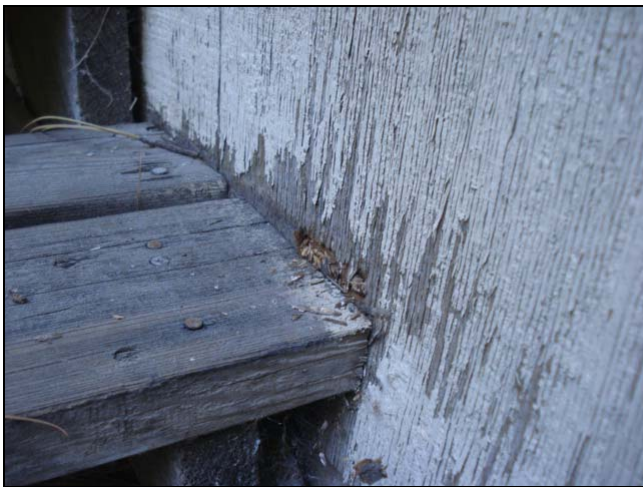
Deterioration in the T1-11. There was no place for the rain water to go but to sit on the step and penetrate into the siding.
