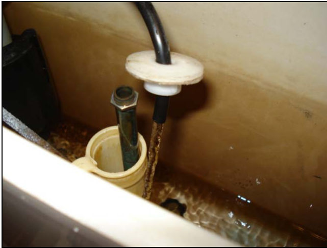
The toilet bowl supply line was loose. The toilet kept on running.
