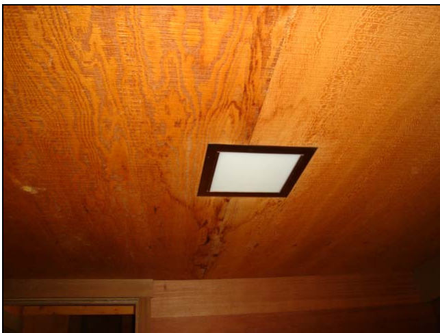
Stains around a light fixture in a wood paneled room.
