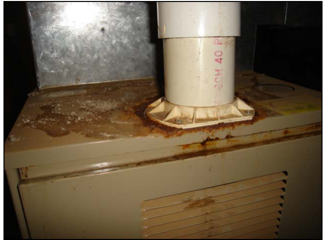
Rust on the top of a furnace housing.
