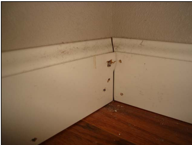
Cracked and swelling baseboard.
