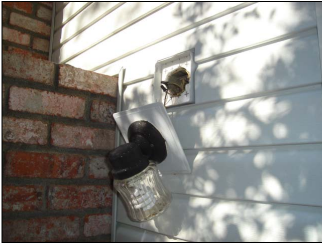
A very loose light fixture.
