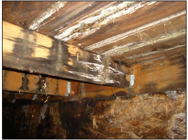
Organic growth and deterioration for the boards and joist.
