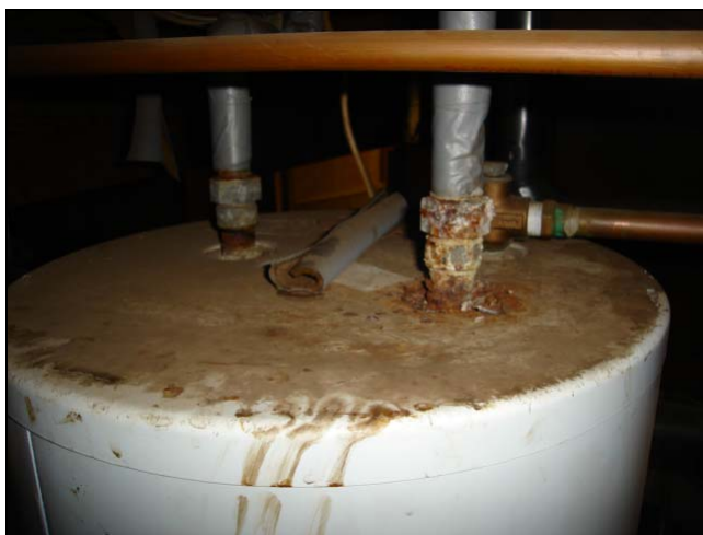
Corrosion, rust and dirt
