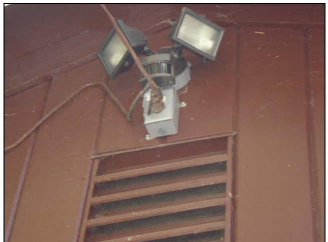
Permanent use of an extension cord.
