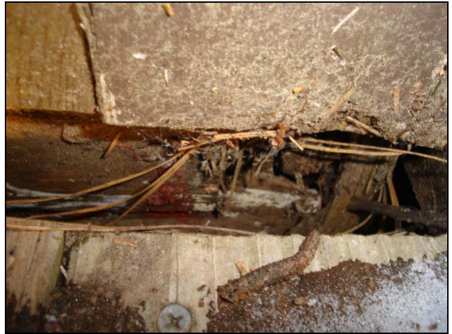
Deterioration between the decking and siding.
