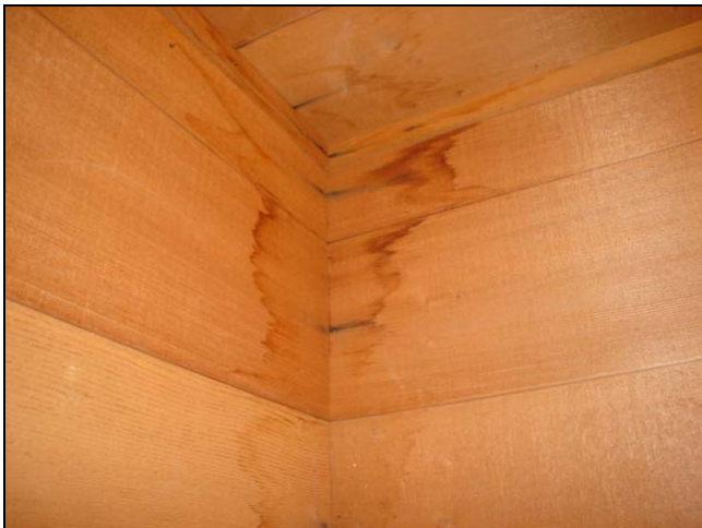
Water stains in wood plank interior siding.
