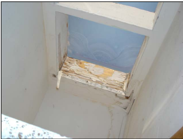
Active water intrusion at a skylight.
