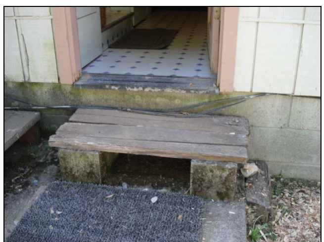
Unsafe construction practices.
