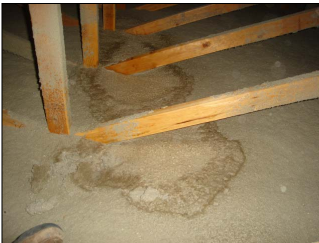
An obvious roof leak.
