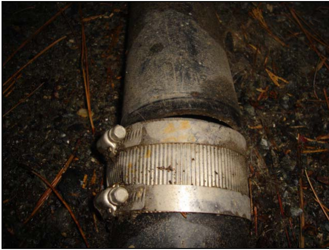
An open sewer pipe.
