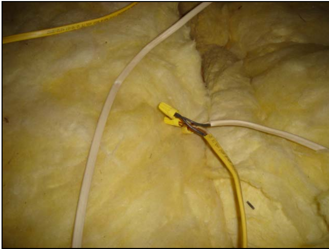
Open splice that should be in a junction box.
