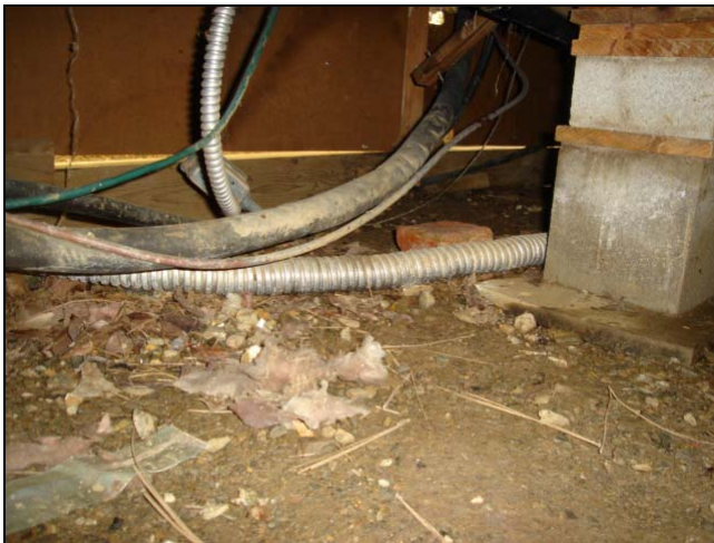
This metal conduit should be suspended above the soil.
