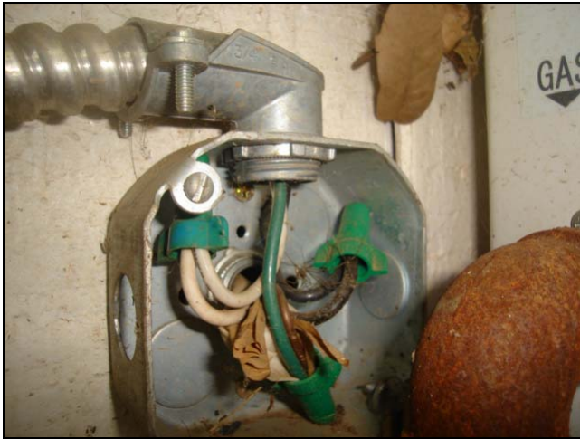
Open junction box.
