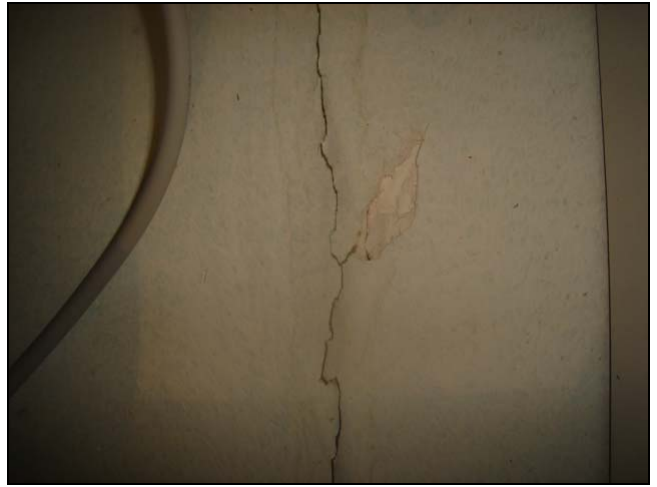
A stress crack.
