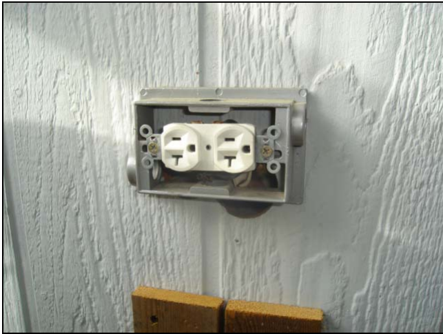
Missing weather cover plate.
