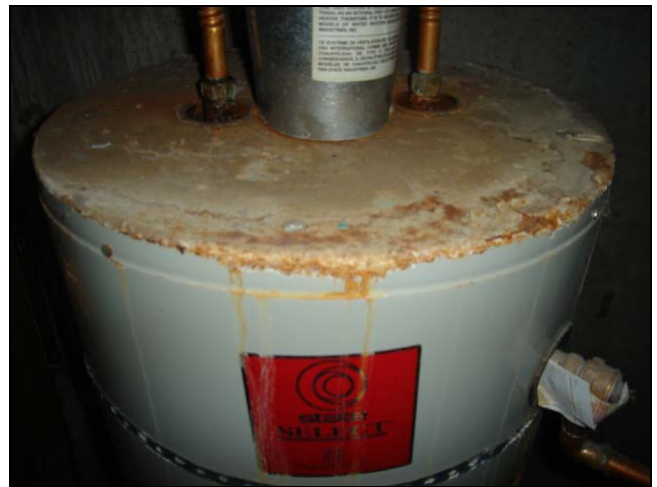
Rusted tank from leaking fittings.
