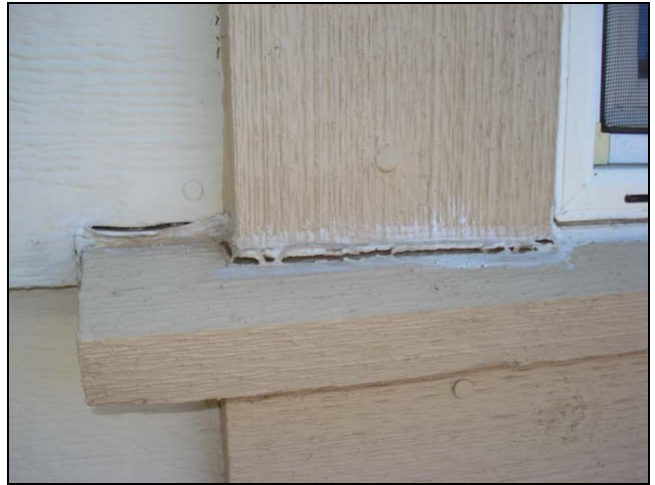
Trim damaged with a flat topped trim board.
