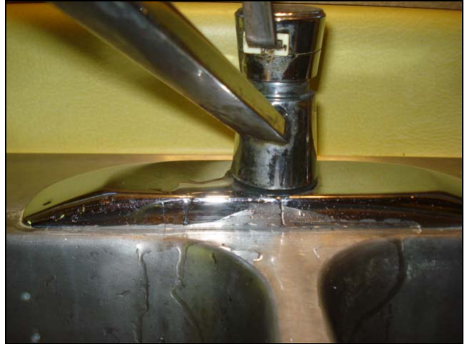
Leaking faucet swivel base.
