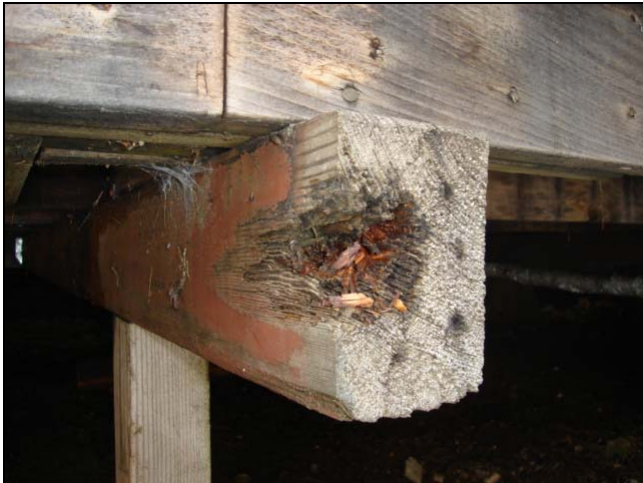
Decay in a beam.
