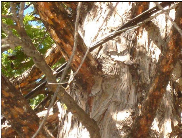
The service drop is grinding into this tree.
