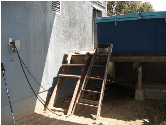
No guard rail, no steps.
