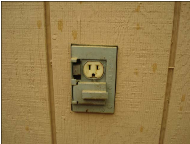
Missing cover on an exterior weather proof cover.
