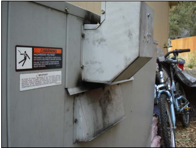
Soot at the exterior of the furnace housing.
