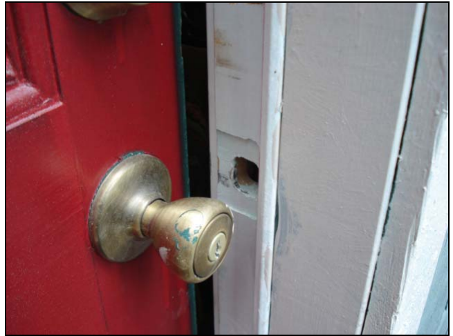
Missing striker plate.
