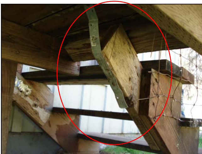
Unusual stair step construction practices.
