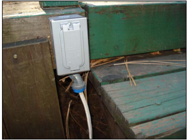
Exposed wiring should be in conduit.
