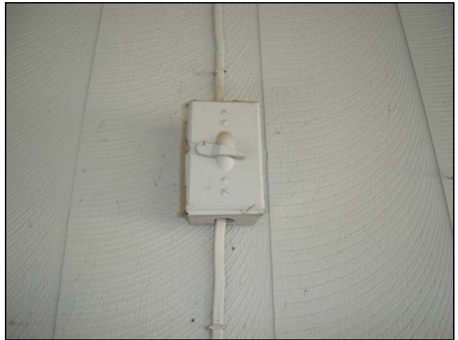
Exposed wiring at an exterior switch.
