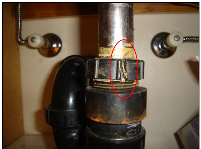
A cracked collar nut.
