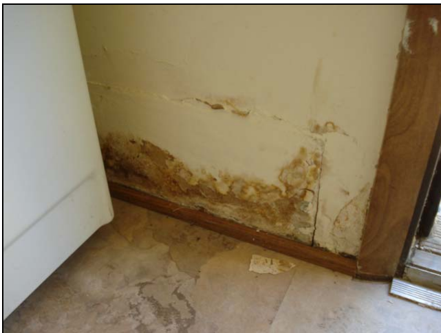
Water damaged wall in a laundry area.
