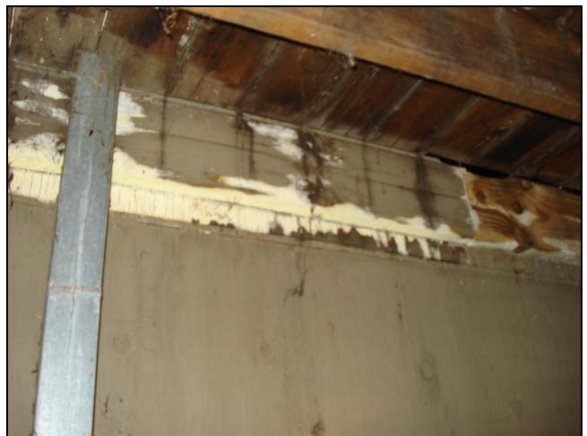
Possible fungus between the decking material and the siding.
