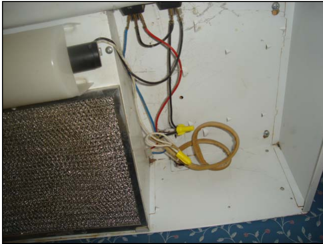
Exposed wiring under a stove hood fan.
