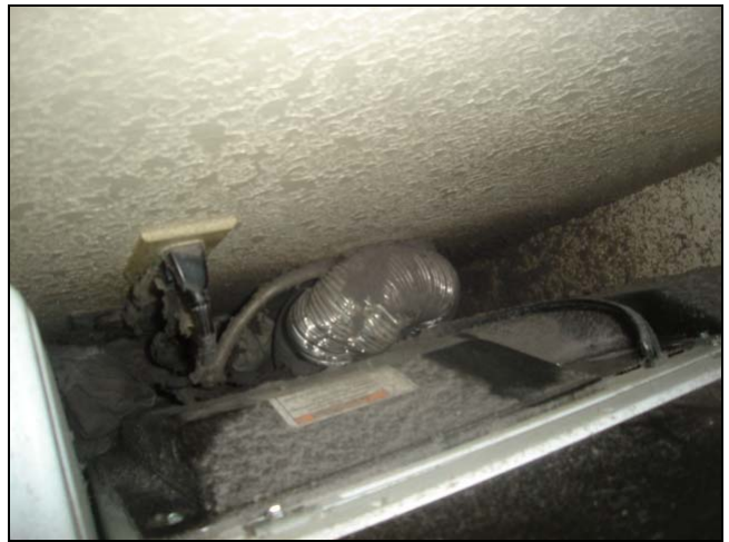
Damaged vent pipe and excessive lint build-up.
