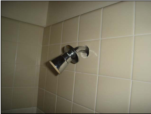
A loose escutcheon plate at the showerhead.
