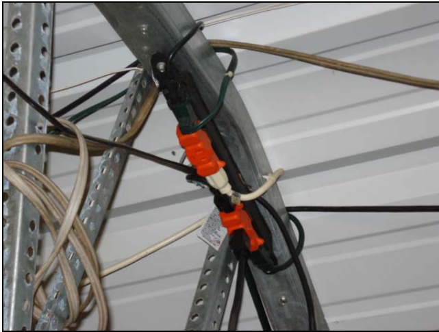
Classic extension cords for permanent wiring case.
