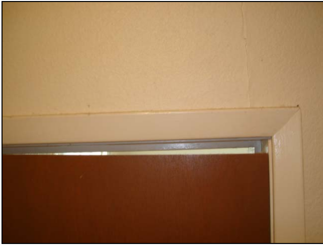
Reveal issue at the top of a door.
