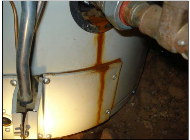
Drain valve leaking.
