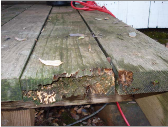
Deck board decay.
