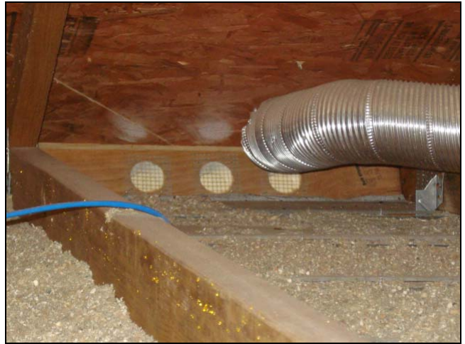
Here is another way contractors route the vent pipe.
