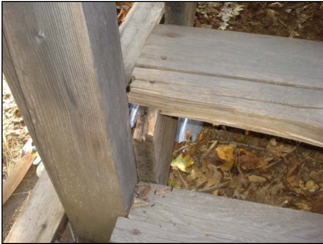
A broken step.
