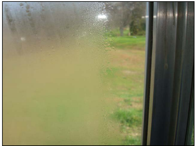
Condensation in a blown window.
