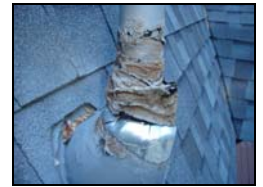
A damaged plumbing vent boot.
