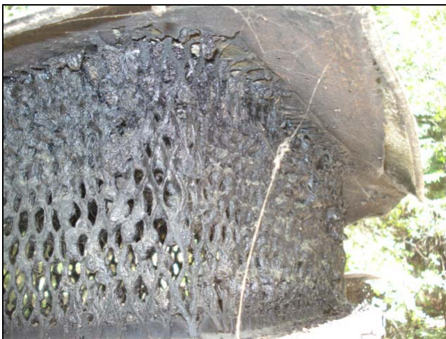
Excessive creosote build up is a major cause of chimney fires.
