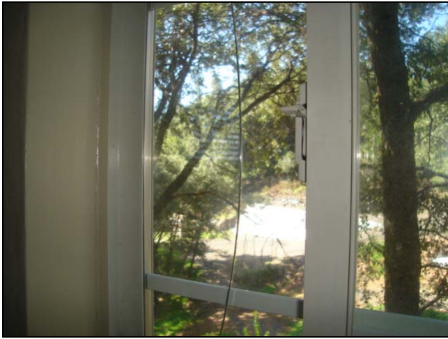
Cracked inner pane of a dual pane window.
