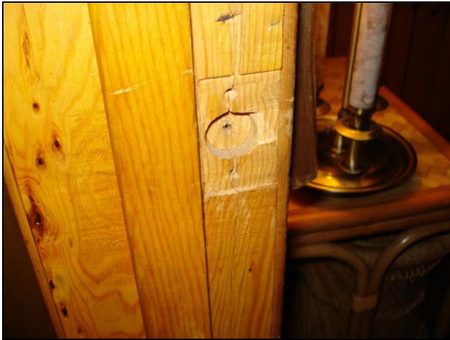
Missing striker plate.
