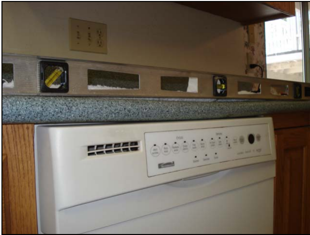
Warped granite countertop.
