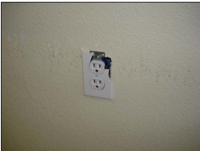
Cracked cover plate.
