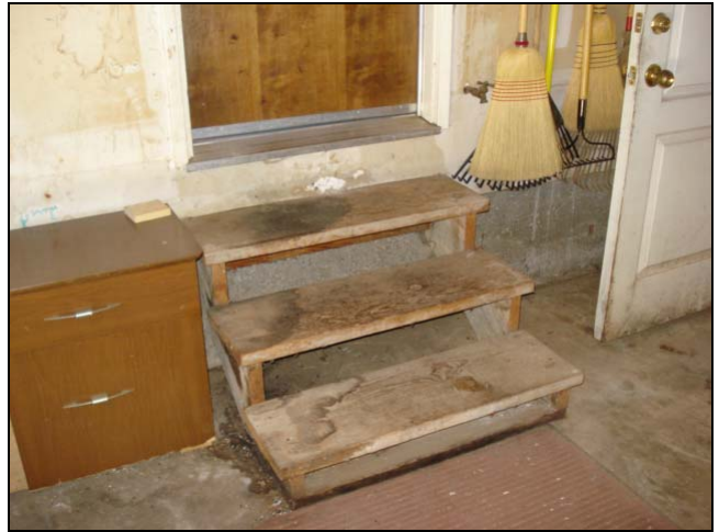
No railing for these 4 steps.
