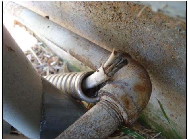
Let's see. Hot wires, open conduit, metal pipe. Not good.
