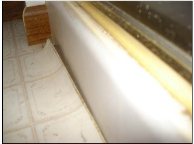
Loose vinyl at the base of a shower. Fix and seal this area and guarantee a note is eliminated.
