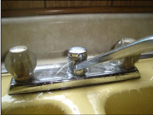
Leaking faucet at the swivel base. Grasping hold of the faucet, knobs of control levers and lifting or twisting them should not produce a leak.
