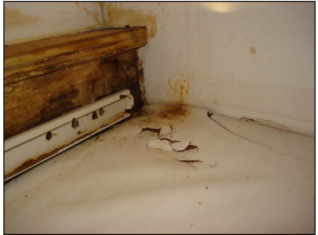
Damage from a water leak. This problem was largely obstructed from view until the pullout drawer was extended.
