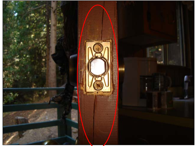
Cracked door edge at the deadbolt latch. This is often caused by not pre-drilling a pilot hole before running in the screws for the latch.
