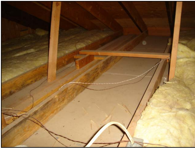
Missing insulation. This condition happens a lot. Particularly when lighting upgrades have been done.
