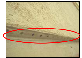
Weep screed holes at the base of the wall allows moisture to evacuate.
