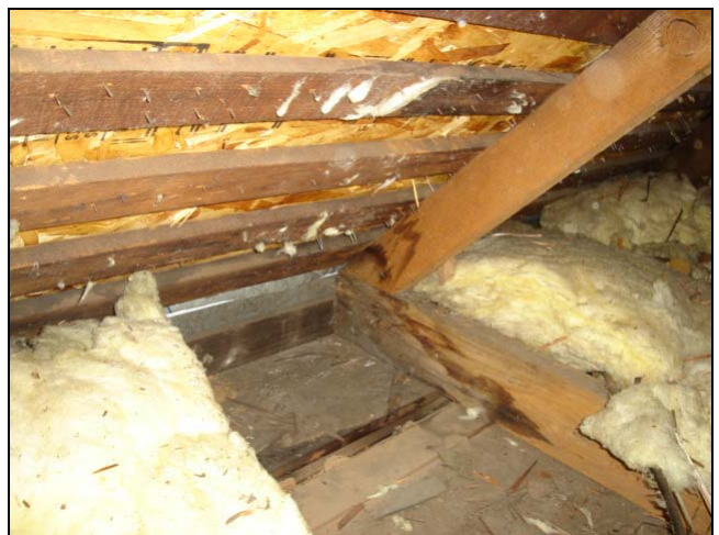
Water intrusion at the roof and missing insulation. Notice the OSB sheathing? Looks like a new roof was installed. This is probably an old stain and the reason for the new roof.
