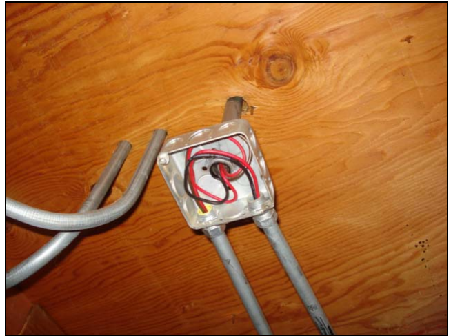
Open junction box. A cheap cover on these will eliminate a note every time. Another “over and over again” issue we see constantly.
