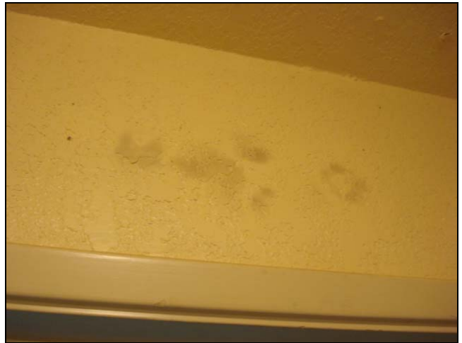
Discoloration over a bathroom doorway. The source of moisture was a damaged grommet at a plumbing vent pipe that penetrated the roof. You will see an example of this in the chapter on roofs.
