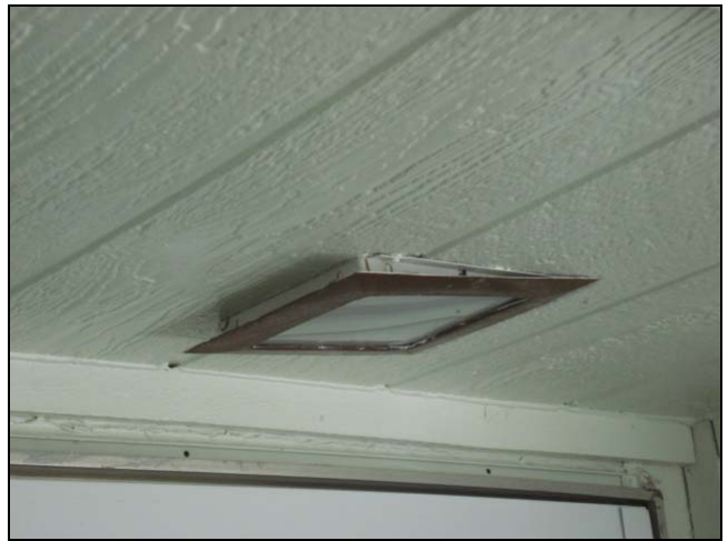
Loose can light fixture.
