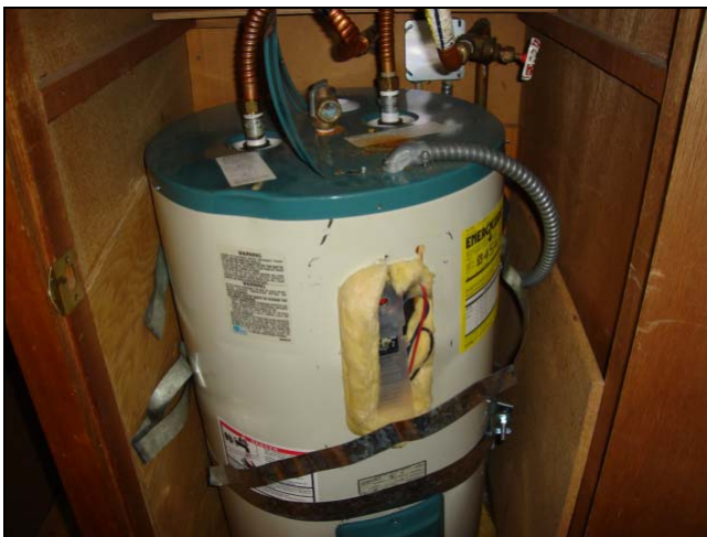
Missing cover plates exposes 220 volts for the children to discover.
