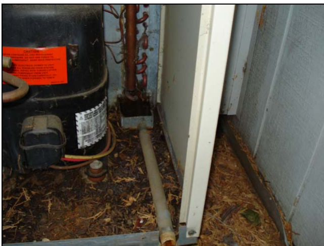
Debris inside an A/C condenser.
