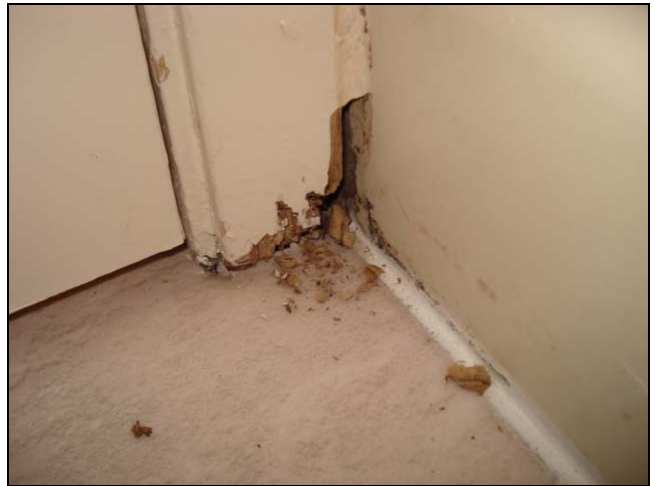
Deterioration at an exterior door.
