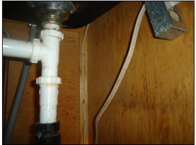
Exposed wiring under a sink.
