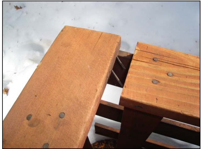
A loose guard railing.
