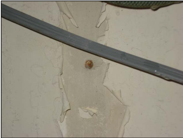
Peeling paint under a bathroom ceiling heater.
