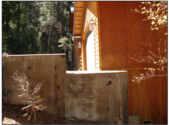
No guardrail for this 6' driveway edge.
