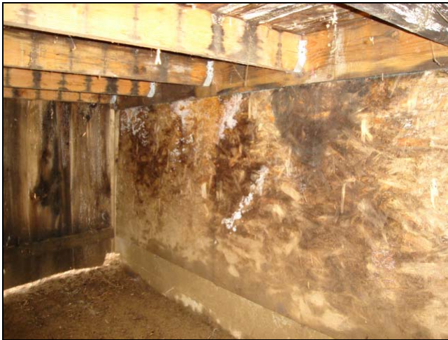
Possible fungus in this storage room under a deck.
