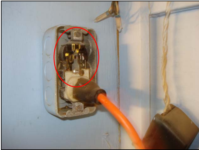
This is not good. The outlet itself is damaged.
