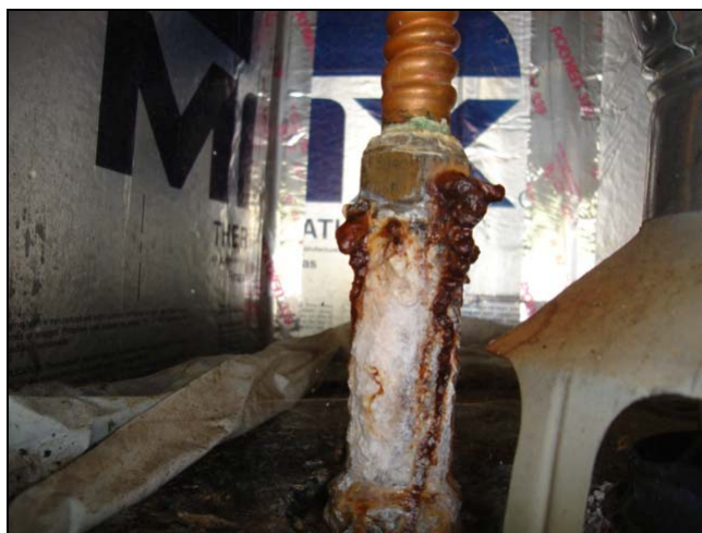
Corrosion and rust.
