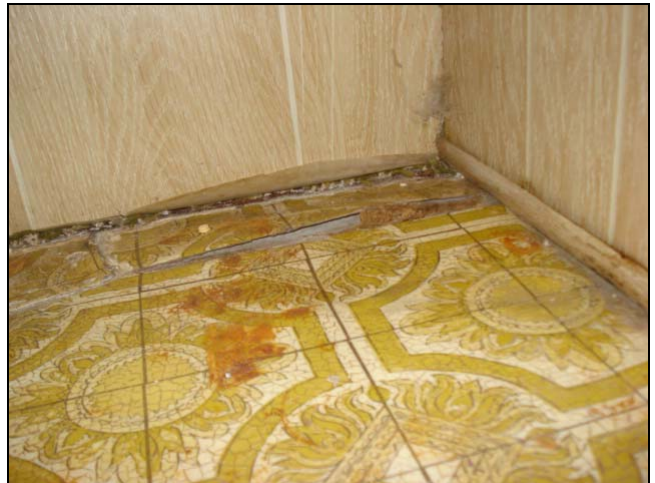
Loose and stained vinyl tile in a laundry room.
