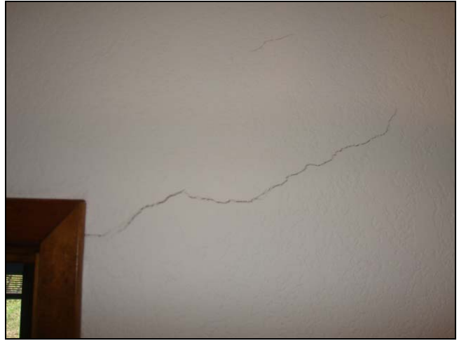
A stress crack.
