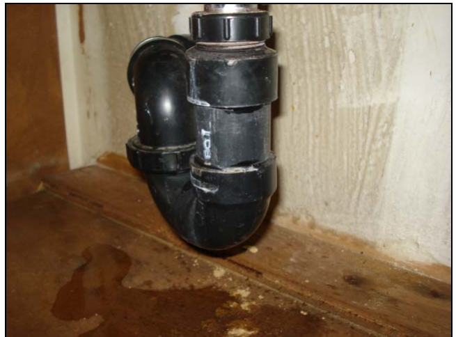
The leaking drain is damaging the cabinet base.
