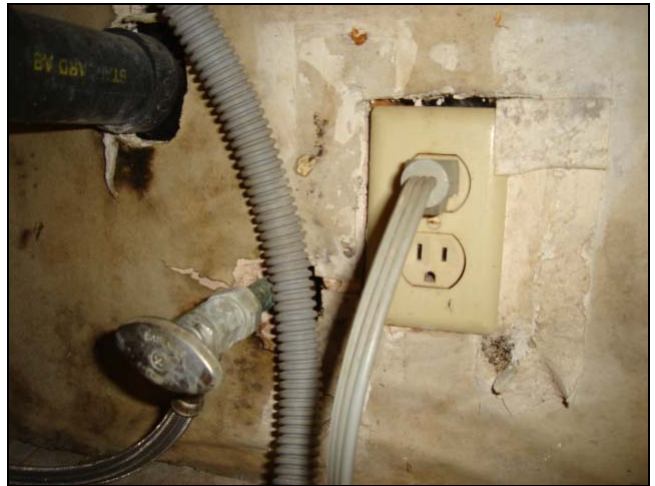
Severe deterioration under the kitchen sink. This may have been picked up while you were inspecting the walls as well.
