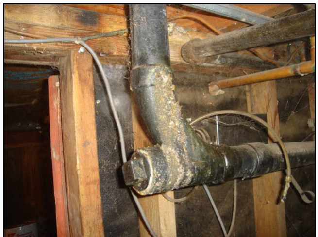
A cracked waste pipe was spewing an unknown material. Well, the material was known.
