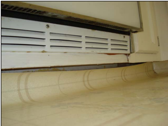
Curled vinyl under a dishwasher. Small brads or finish nails could be used to secure the vinyl.
