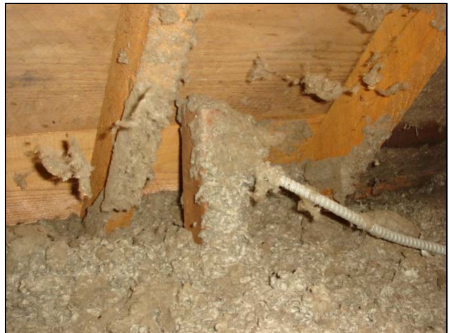
This is not an open junction box. This is a completely covered in insulation junction box.
