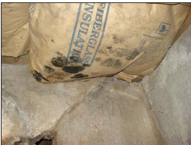
Evidence of organic growth in this insulation that was installed upside down.
