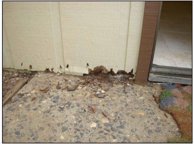
Deterioration in the T1-11. The siding should be at least 2" above the concrete.
