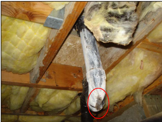
An active water leak under a shower.
