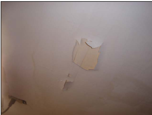
Peeling paint and water stains.
