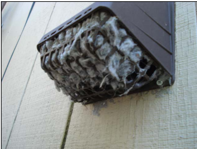
Diffuser plugged with lint.
