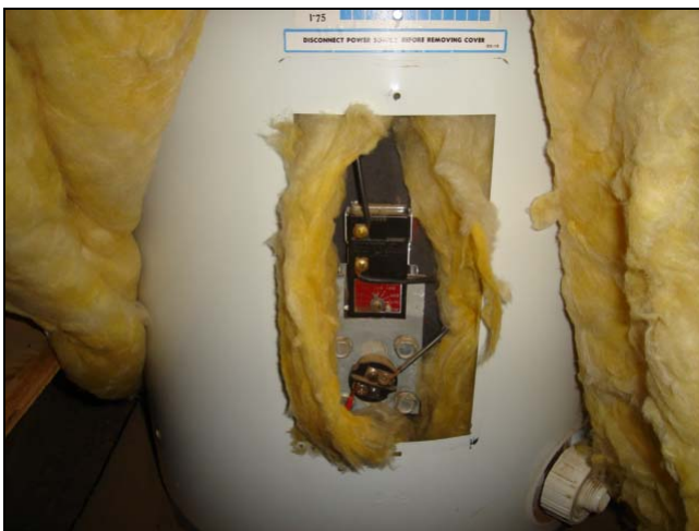
Missing cover plates.
