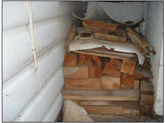
Painted log slag siding and firewood equals a bug super highway.
