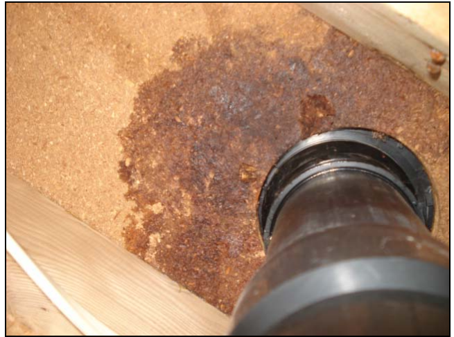
Water soaked sub flooring under a toilet.
