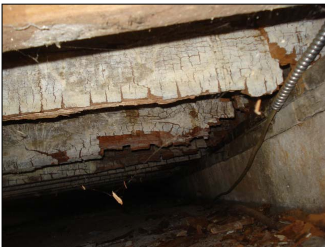
Severe deterioration in these joists.
