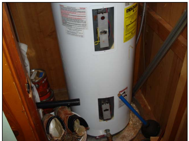
Missing cover plates.
