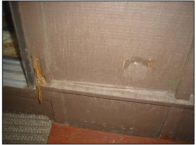
Damaged board and batten panel and trim.
