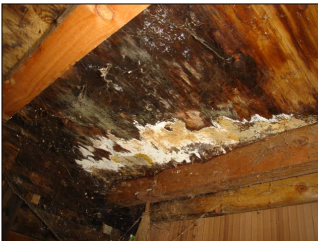
Severe deterioration and fungus in this sub floor.
