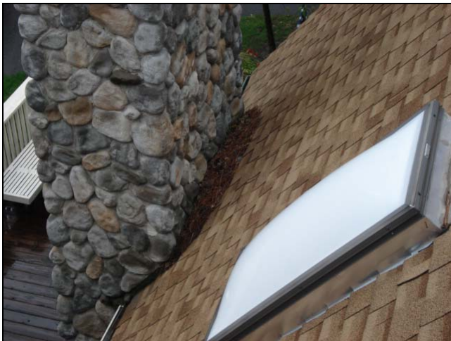
This chimney was over four feet wide. A cricket should be installed to divert water from behind it.
