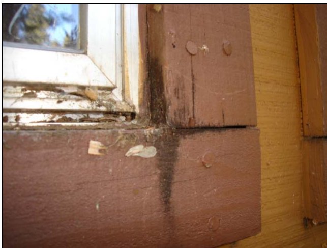
Wood trim deterioration, exterior.
