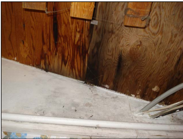
Possible organic growth around this roof leak.
