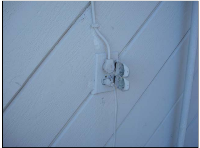
Extension cords being used for permanent wiring.
