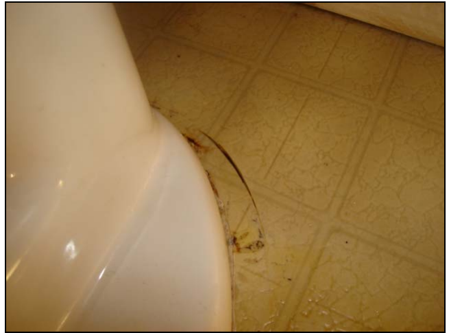
Cracked and deteriorated vinyl tile behind a toilet.
