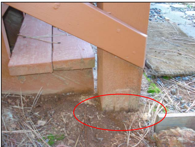
Wood to earth contact at a post.
