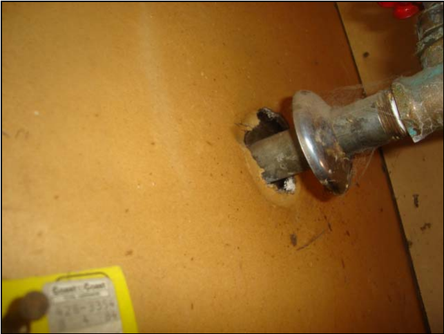
A loose escutcheon plate at an angle stop valve.
