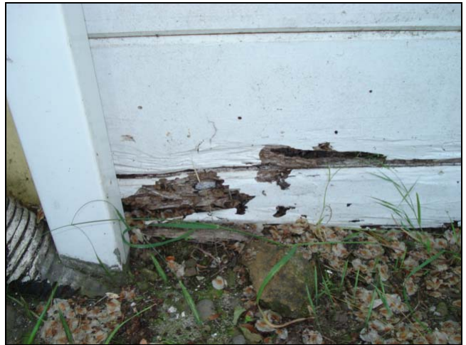
Note: Wood-to-earth contact and deterioration was noted at...
