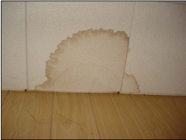
A water stain in a closet.
