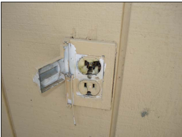
Missing cover and cracked receptacle.
