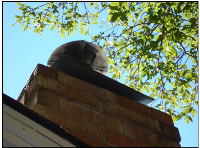
Foliage over a chimney should be cleared away.
