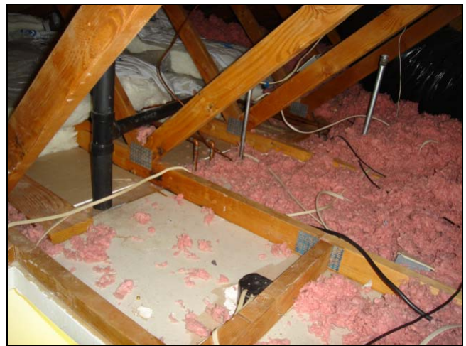
Missing blown in cellulose insulation.
