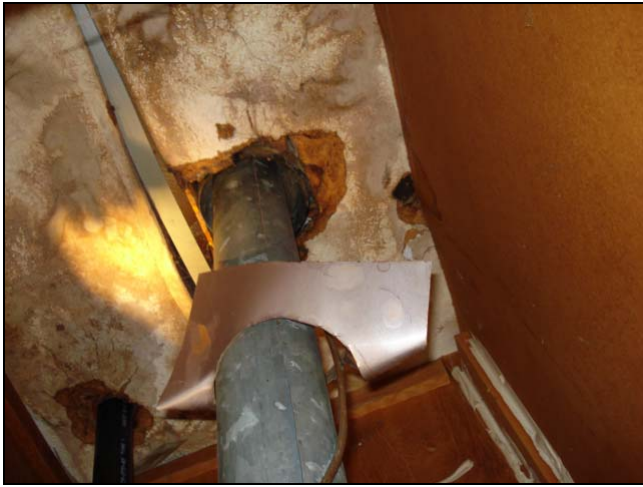
Damaged shielding revealed vent pipe in direct contact with flammable materials.
