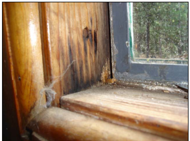
Deterioration and stains, interior.
