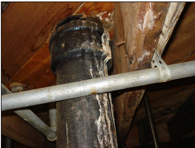
Evidence of a water leak under the toilet.
