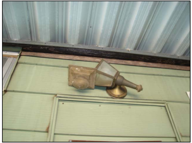
Loose light fixture.
