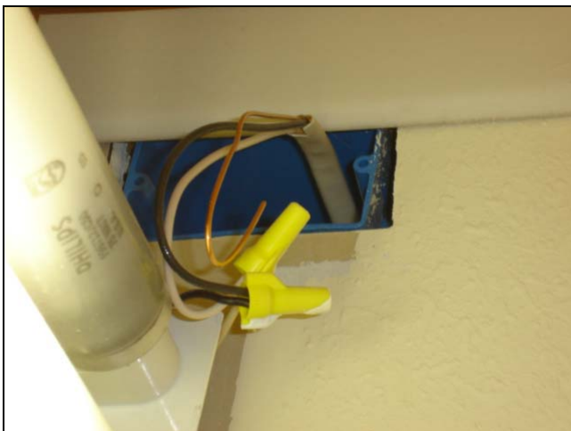
This splice was for a light fixture in a closet. The loose copper wire is the ground wire. I wonder why the ground wasn't hooked up?
