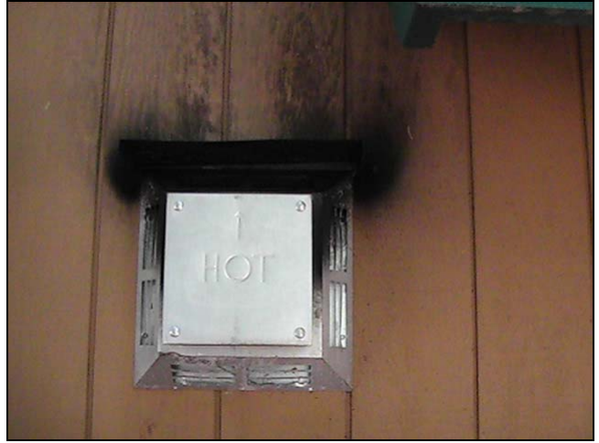
The excessive soot around this direct vent bonnet was possibly caused by natural gas orifice jets installed on a propane gas stove.
