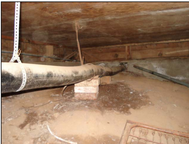
Sagging waste pipe will collect material in the low spots and could become clogged.
