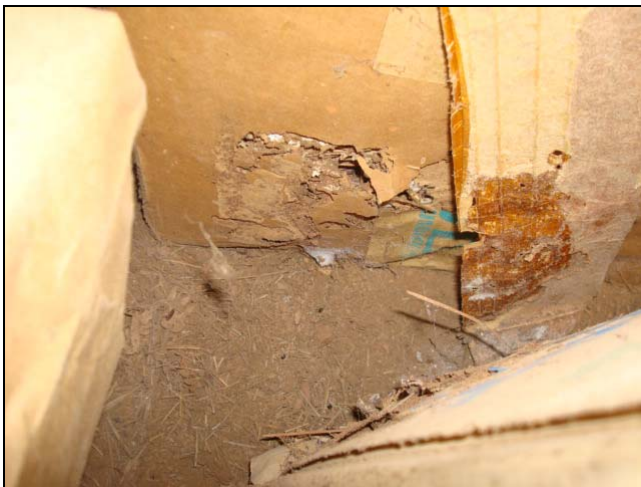
Termite damage. Remove all cardboard and wood debris from the crawl space.
