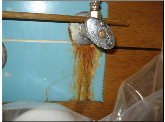
Rust under the angle stop valve. Water may have leaked into the wall.
