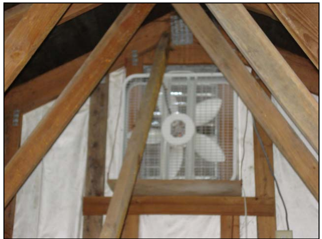
A great way to alleviate moisture and heat build-up in an attic space is to install a fan. This interior fan may not be a recommended model however.
