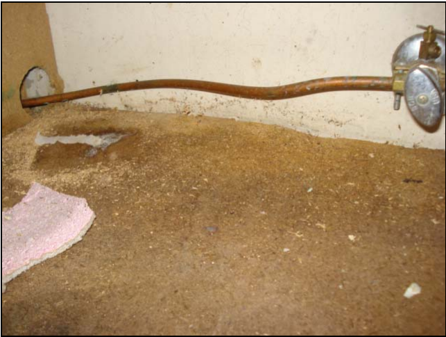
A leaking dishwasher supply line has damaged the cabinet base and stained the wall.
