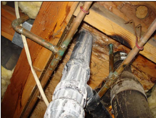
Water damage at the sub flooring under this drain pipe.
