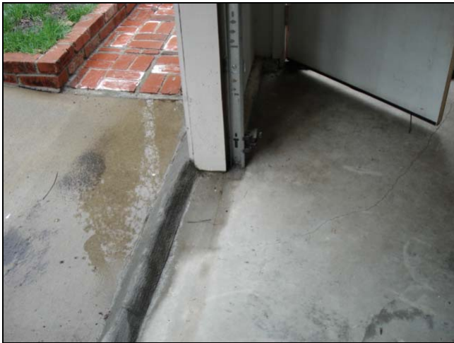
Water intrusion where the door seal had failed.
