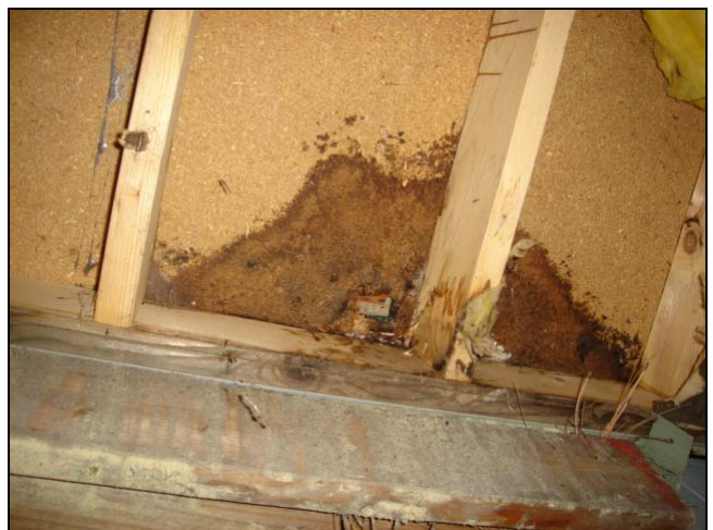
Water intrusion in this manufactured home.
