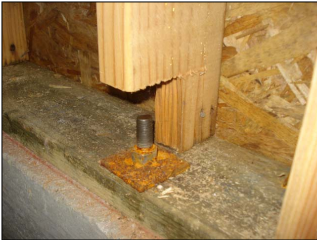
Over notched stud.
