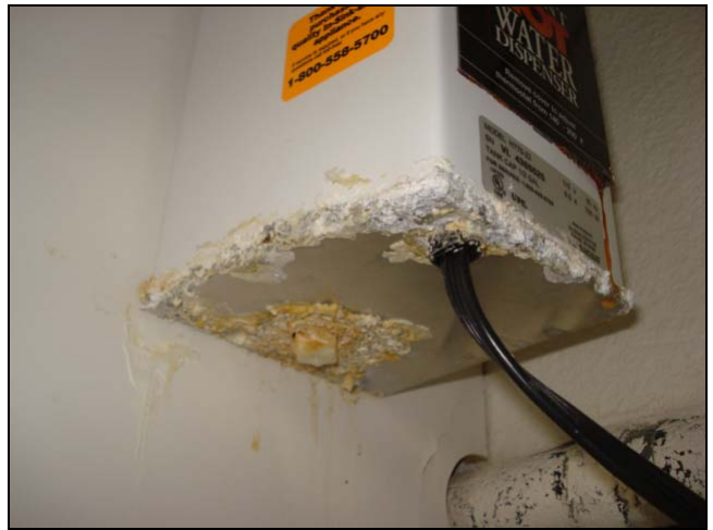
Corrosion on an instant hot water dispenser.
