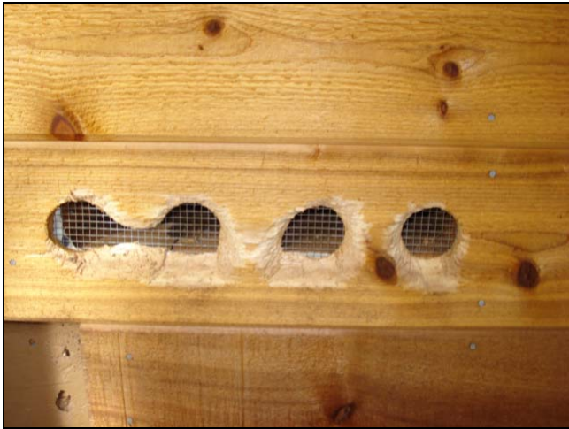
Something was digging its way into these vents until the homeowner installed the screen mesh.
