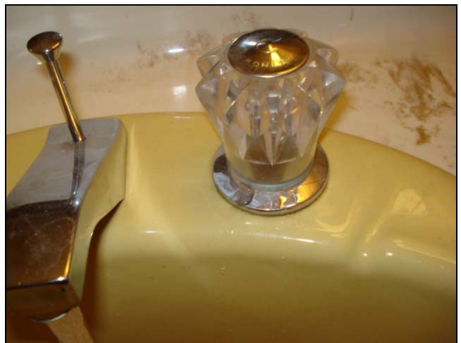
A leaking cold water control valve.
