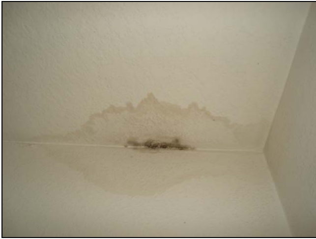
Organic growth and stains.
