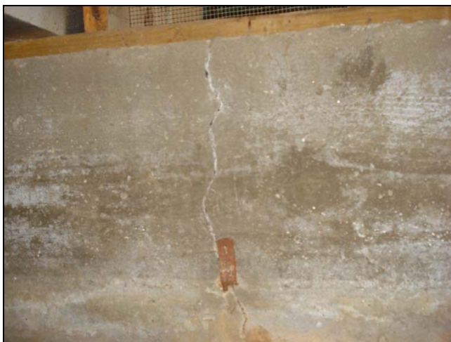
Foundation crack. Appears to be stable.
