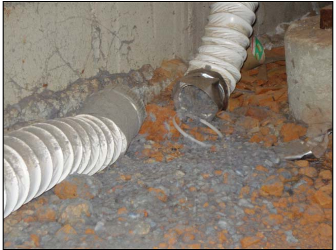
Damaged dryer vent pipe. Plastic pipe is not recommended.
