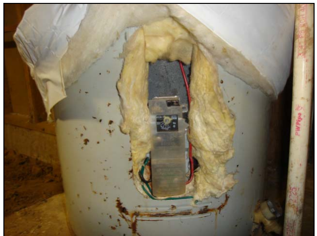
Missing cover plates.
