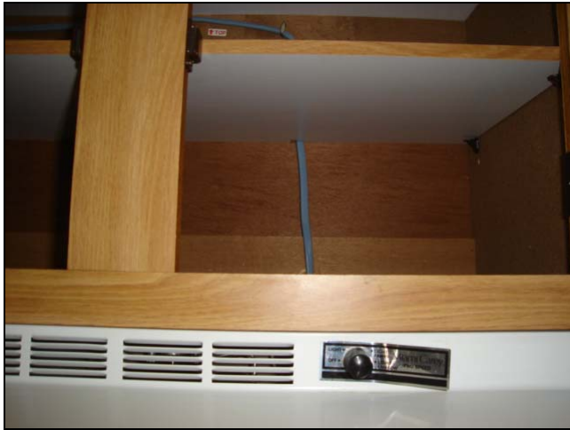
Exposed wiring in the cabinet over the stove exhaust fan.
