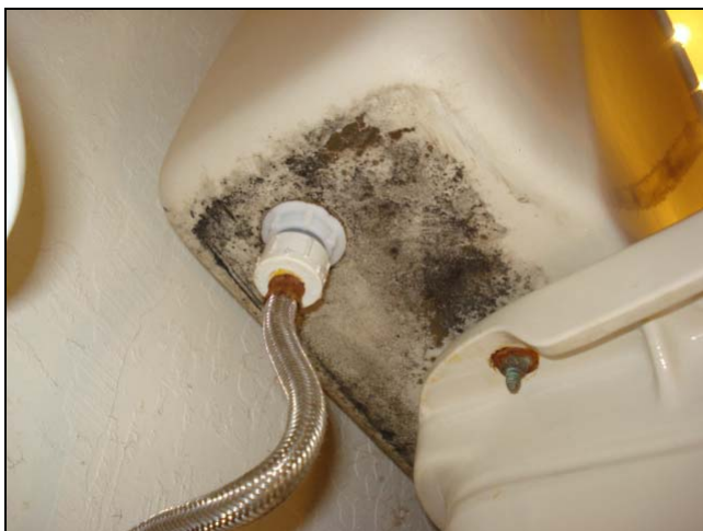
Mildew from condensation under the toilet tank.
