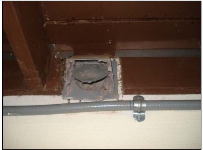
Diffuser plugged with lint.
