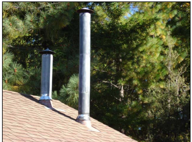
The tall pipe should have been braced.
