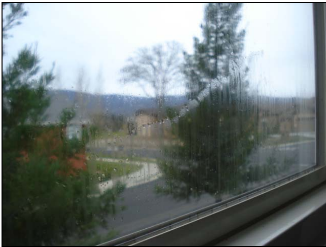
Condensation between the panes of glass.
