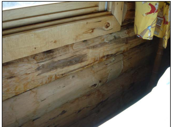
Water stains under a window in a log cabin.
