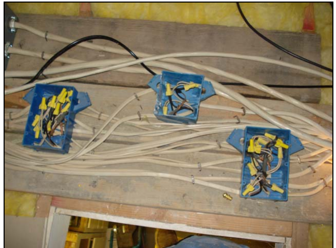
Looks scary but all that was needed were the covers.
