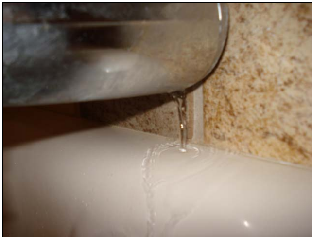
Leaking tub spout.
