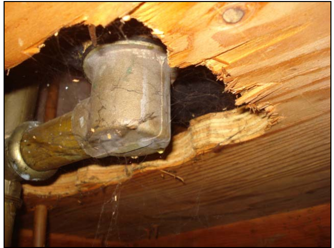
This tub drainpipe was leaking.
