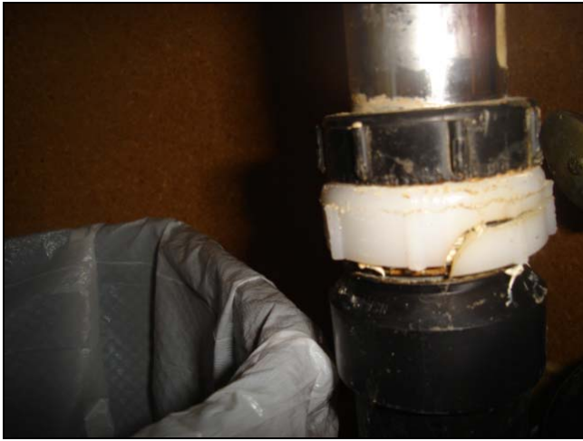
A cracked collar nut.
