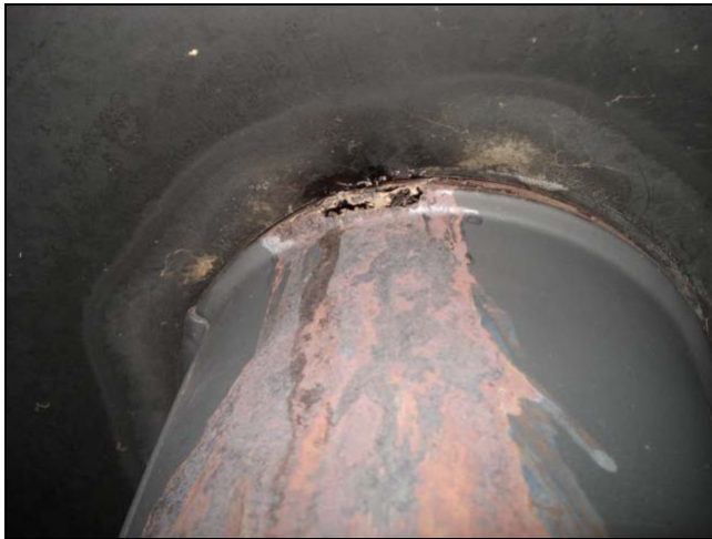
This damaged pipe will leak combustion gas into the living space. This is a HAZARD .
