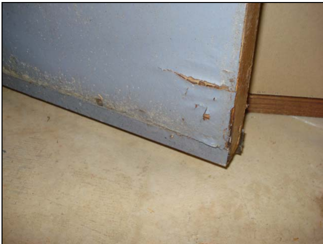
Deterioration in the door.
