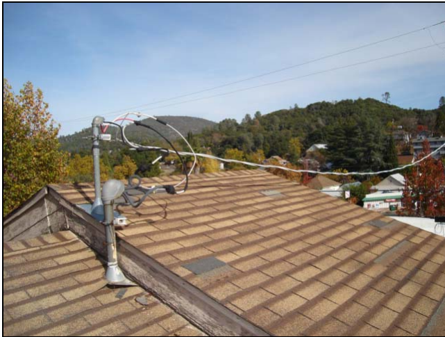
Service drop traverses a roof.
