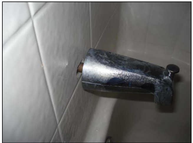
Recommend sealing the spout at the shower wall.
