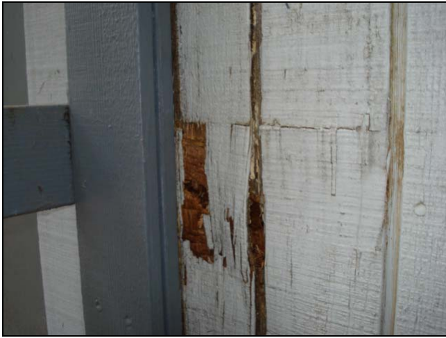
Deterioration in the T1-11.
