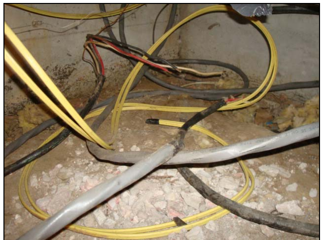
A wiring snake pit. These wires were abandoned when a room addition was built.
