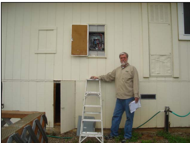
This sub panel was clearly too high. I am not sure how this got past the building inspector.
