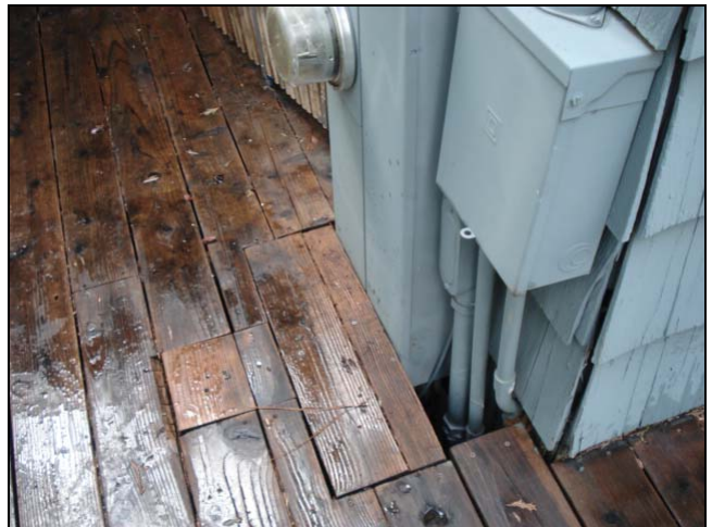
A deck board has to be lifted to open this cover. Snowfall common in this area will make this task almost impossible.
