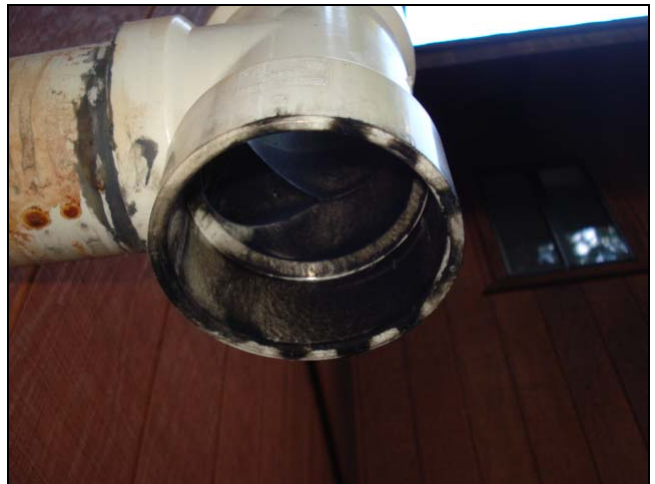
This is not a good sign on high efficiency furnace exhaust pipe. Wrong gas jet orifices perhaps?
