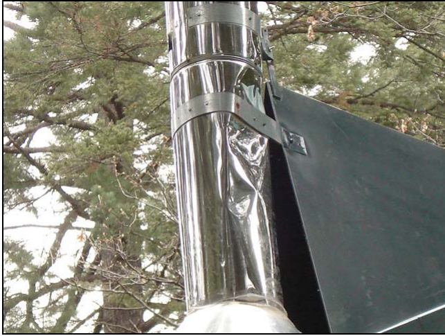
The damaged pipe could restrict the proper drafting. Recommend having a licensed Chimney Sweep inspect for further information.
