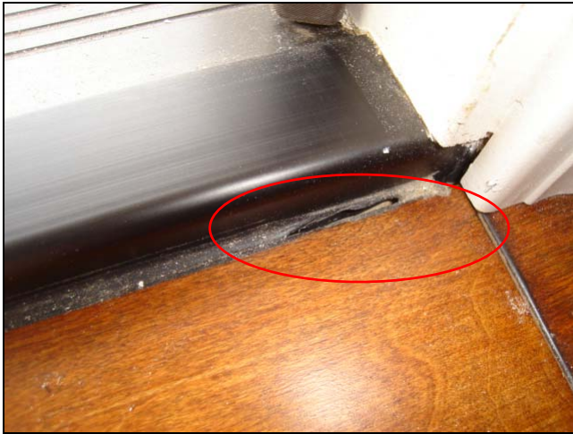
A gap at the threshold that should be sealed. Seal this gap and guarantee a report note is eliminated.
