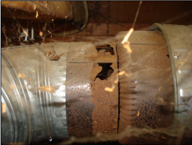
Holes in the flue pipe under a building is not good. This is a source of "Flue Gas Spillage."
