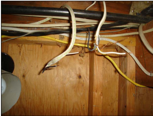
Un-terminated wiring was HOT! The tool shown at the right is provided in the Premier Package and is used to determine if the wires are hot without touching them.
