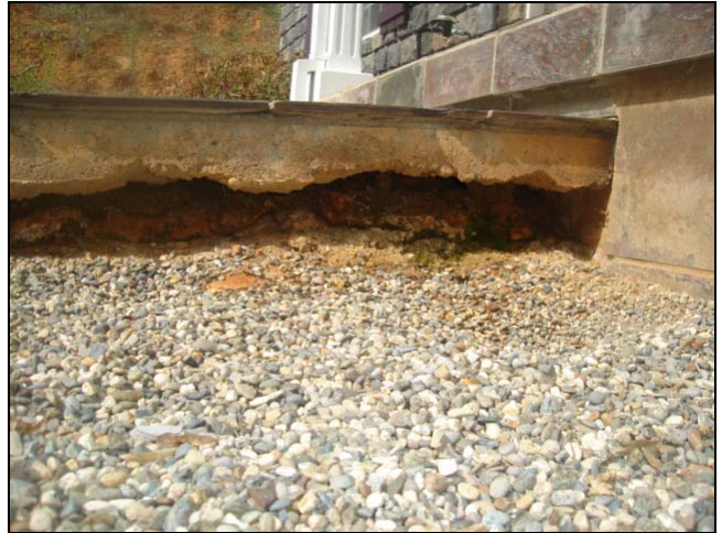
Erosion under a walkway.
