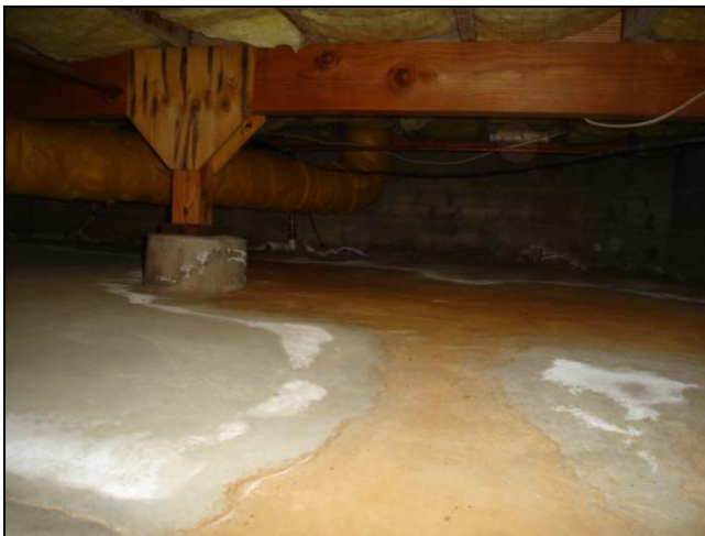
Evidence of flowing water under this building.
