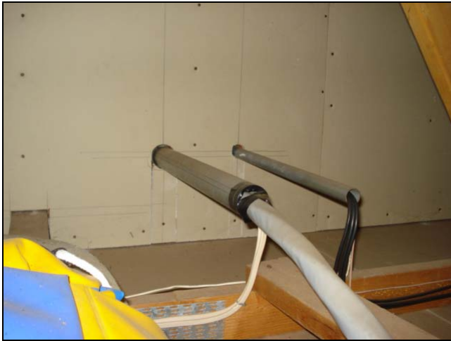
The small gaps around these pipes should be sealed.
