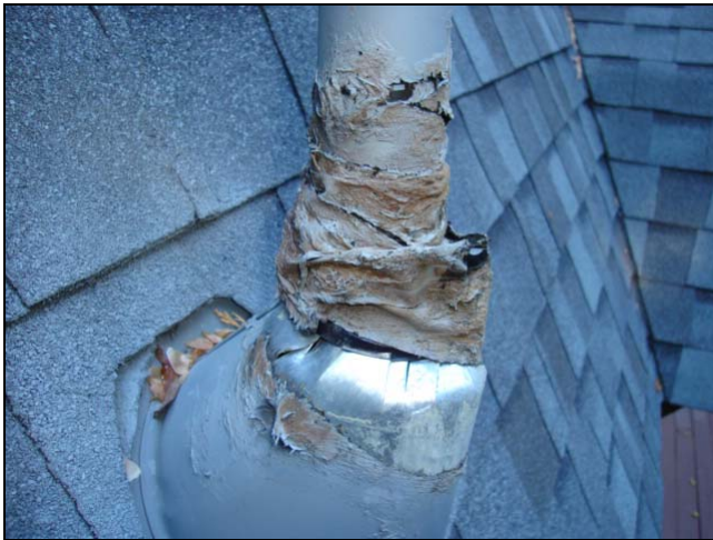
This is a plumbing vent boot. This one leaked.
