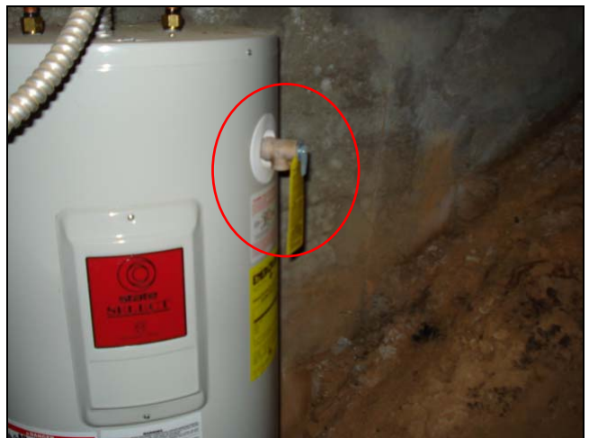
TPR valve with no discharge pipe.
