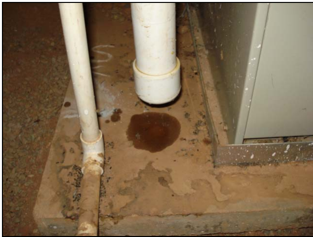
A water leak from a condensate pipe.
