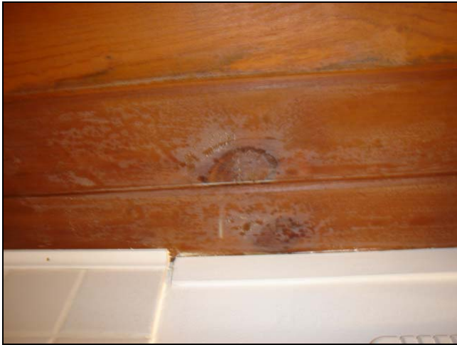
Stains from condensation in a bathroom.
