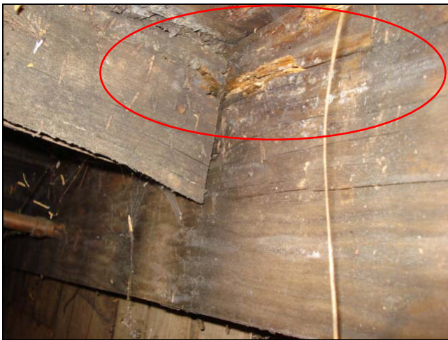
Deterioration in this deck beam.
