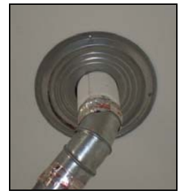
Vent pipe collar
