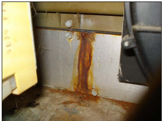
Rust from a leaking housing.
