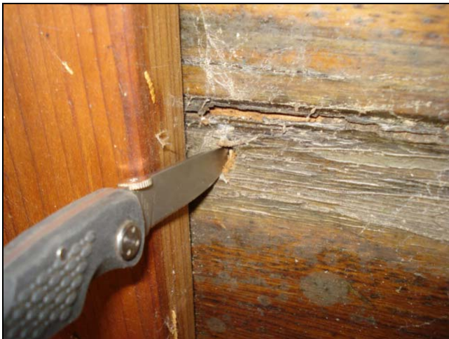
Stains and beginning signs of deterioration.
