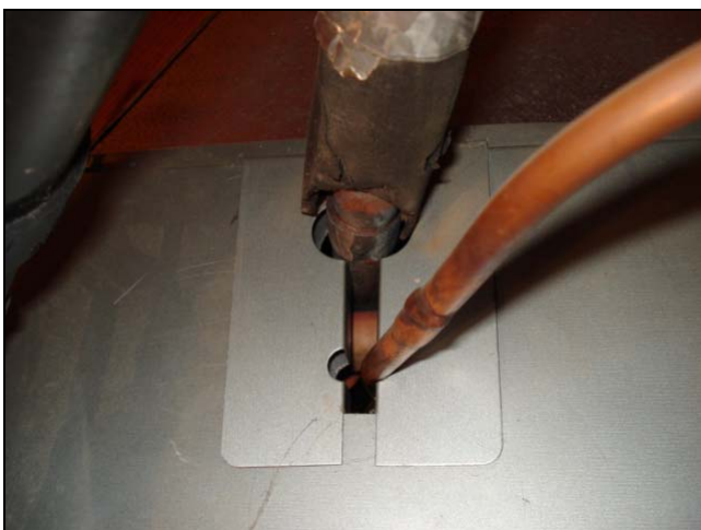
Gaps around these A/C lines should be sealed.
