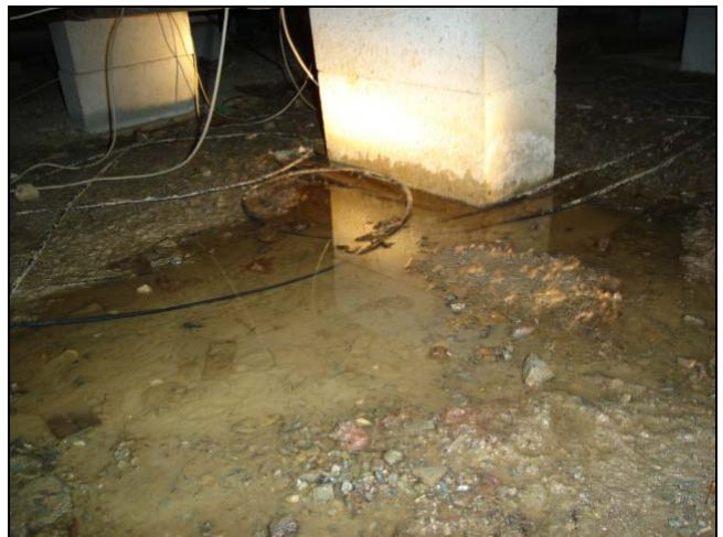
Standing water is not good.
