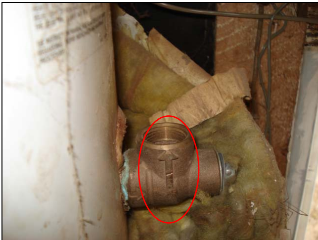
I guess the installer thought the arrow meant "up".
