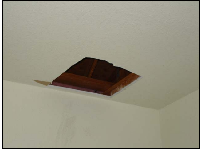
An opening in the fire envelope of the garage.
