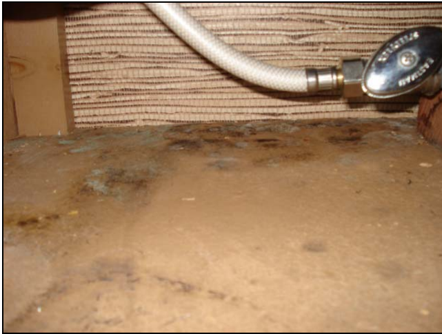
Organic growth in the cabinet base.
