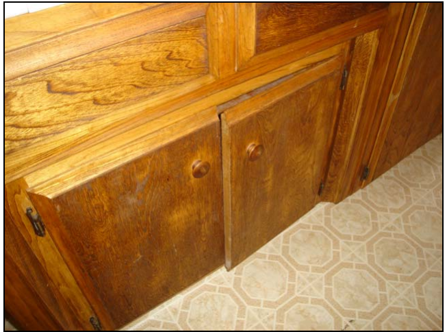
The doors did not properly close.
