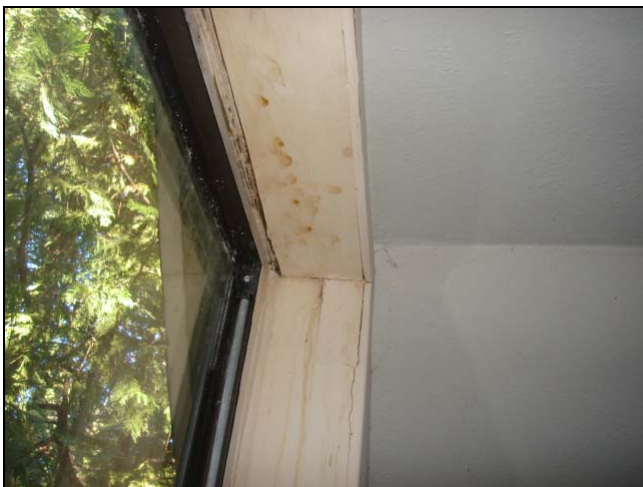
Water leaks over the window. Possible damage at the header in the wall. Water intrusion at the exterior trim from poor flashing.
