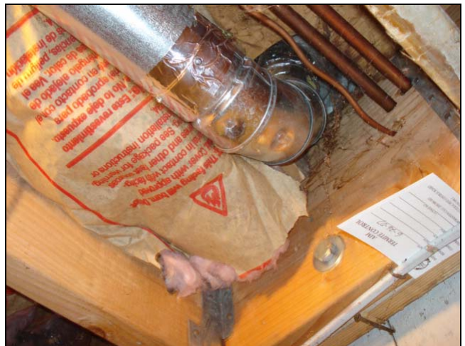
The insulation was installed upside down and in direct contact with the heater flue pipe.
