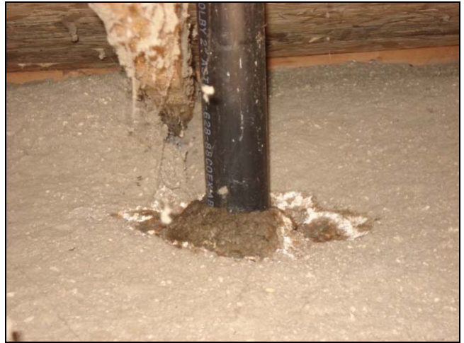
This is a plumbing vent pipe that had a leaking vent boot.
