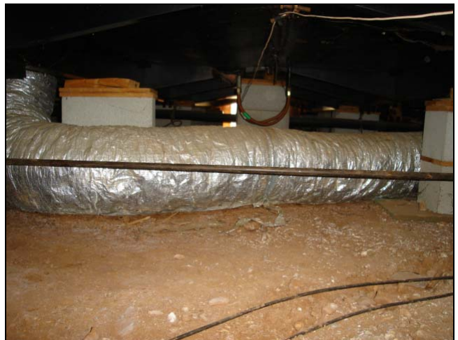
The HVAC ducting should be suspended above or isolated from the soil.
