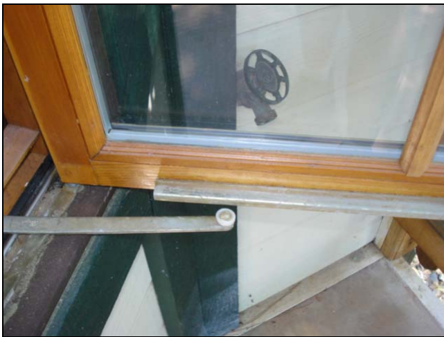
Loose casement mechanism. This window was impossible to secure unless someone was at the exterior and pushed the window closed.
