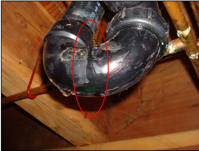
An active water leak. The green fluid is antifreeze used to winterize this empty cabin.
