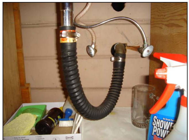
Is this a "U" trap? The radiator hose should have a smooth continuous inner surface. Yeah right.
