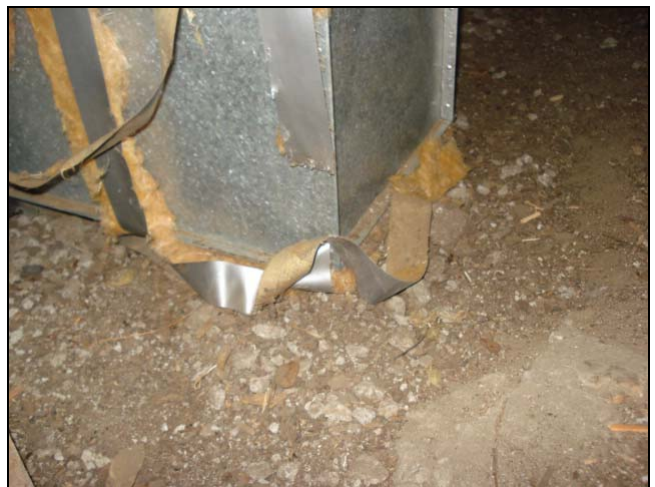
Loose vinyl duct tape is common. Conditioned air was leaking into the crawl space. Also, the soil should be cleared away from the housing.
