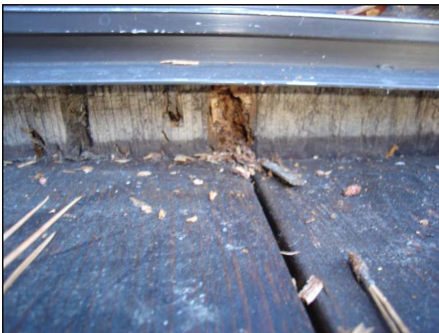
Deterioration between the decking and siding. This problem regularly occurs under patio doors.
