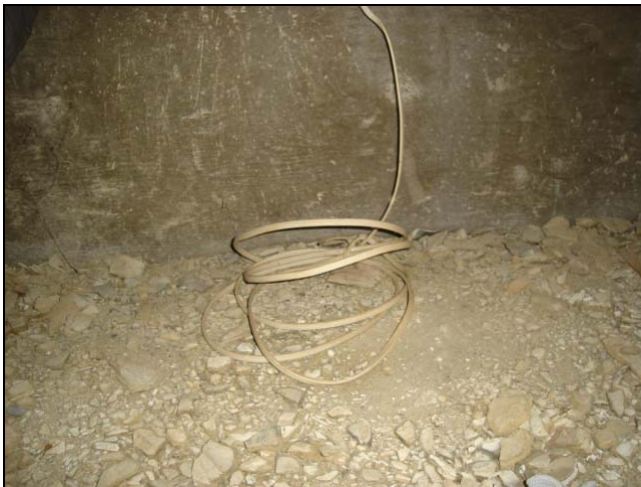
Another loose cable. At the very least, put a tag on it that says "For future wiring" or something.
