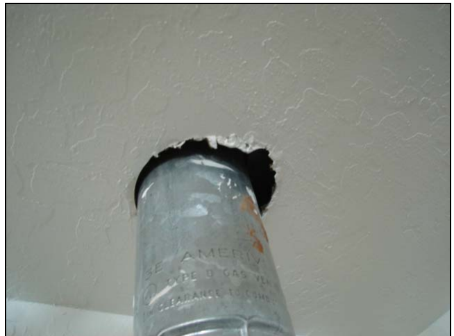
A penetration through the firewall around a water heater vent pipe. The collar pictured in the margin above would have been appropriate here.
