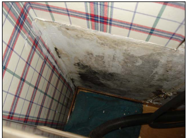
Organic growth behind a washer. The washer drain hose leaked and soaked the wall. Nobody ever looks back here.
