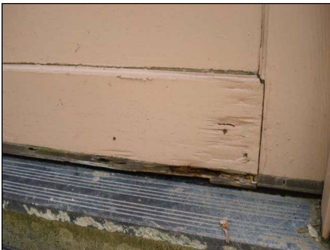
Damaged lower panel will be noted by a termite inspector as well as the home inspector.
