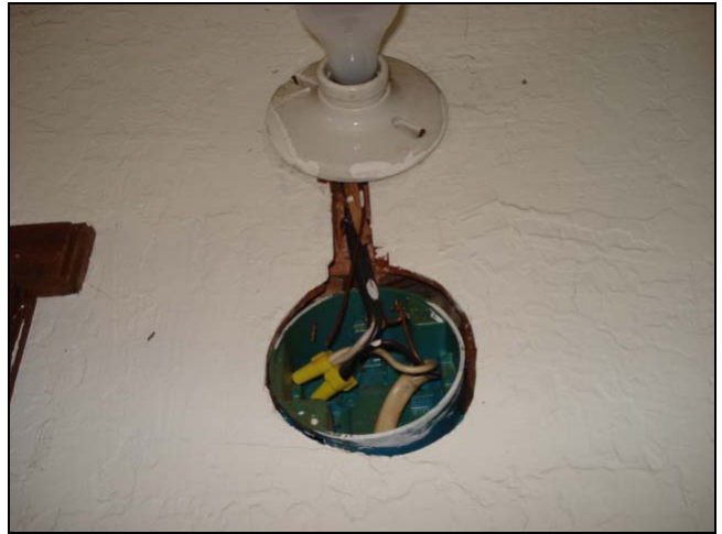
I guess the light fixture just wasn't high enough...
