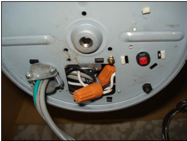
Missing electrical coverplate.
