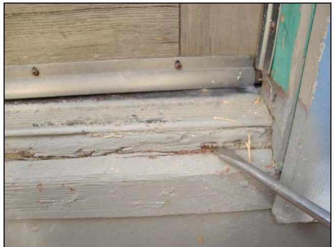
Deterioration in the threshold.
