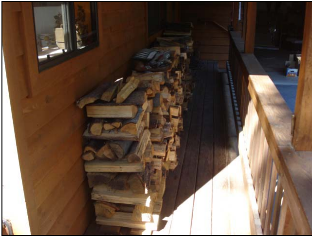
Firewood and stained lap siding. Not a good storage idea.
