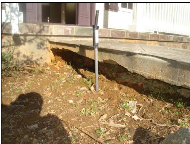
Erosion under a walkway.
