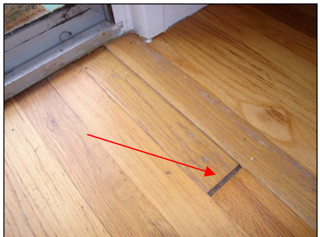
A slipped wood plank.
