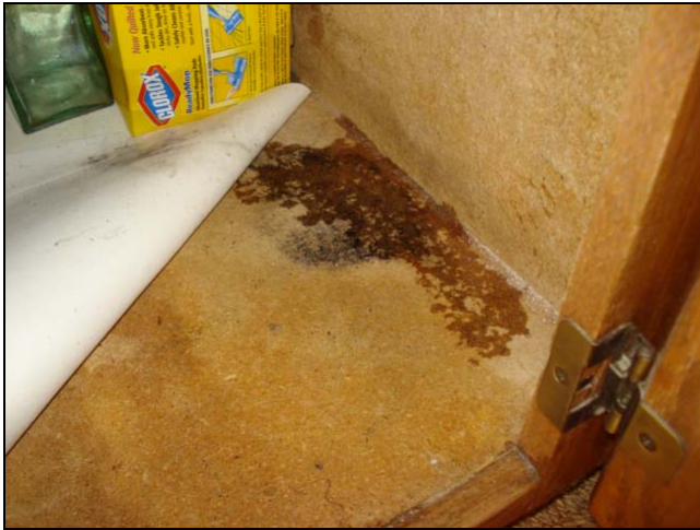
Water or soap spill.
