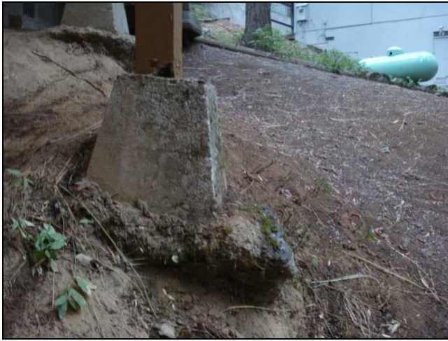
Erosion around a deck pier.
