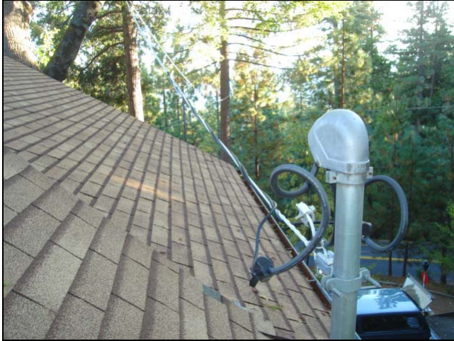
Service drop traverses a roof.
