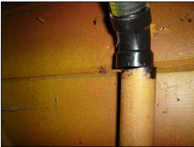
A loose drain pipe.
