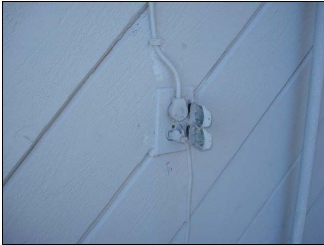
Extension cords being used for permanent wiring.
