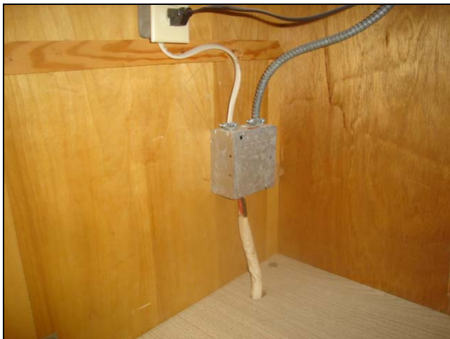
Exposed wiring under an electric cooktop cabinet.
