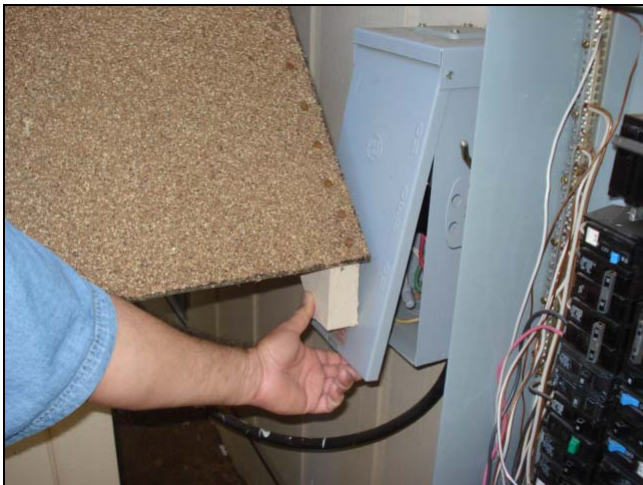
The storage shed blocked the access to this box.
