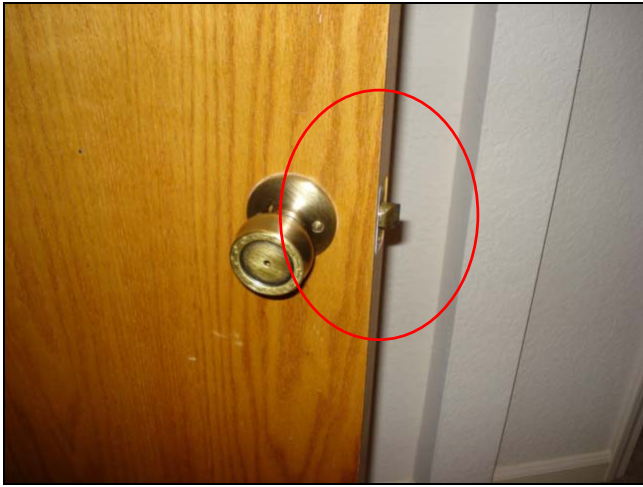
This door latch is installed backwards.
