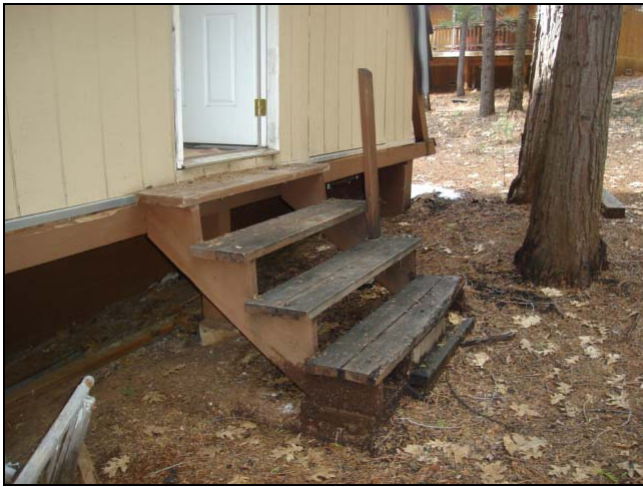
No railing for these 4 steps.
