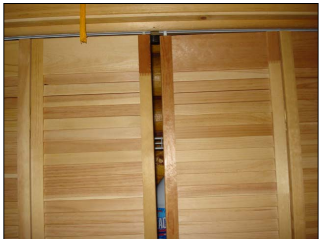
The closet doors do not quite reach.
