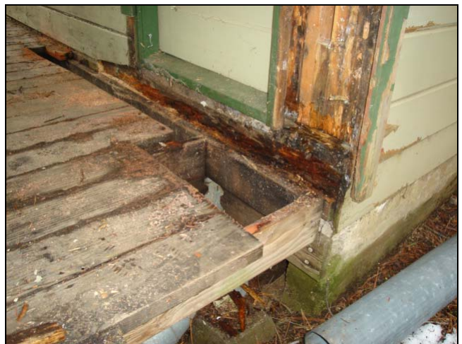
Deterioration between the decking and siding.
