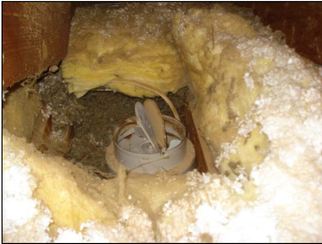
This bathroom fan pumps directly into the attic.
