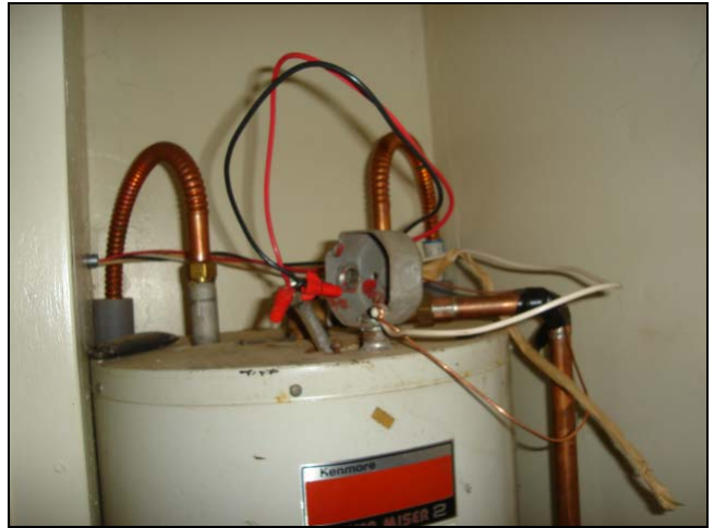
A wiring mess.
