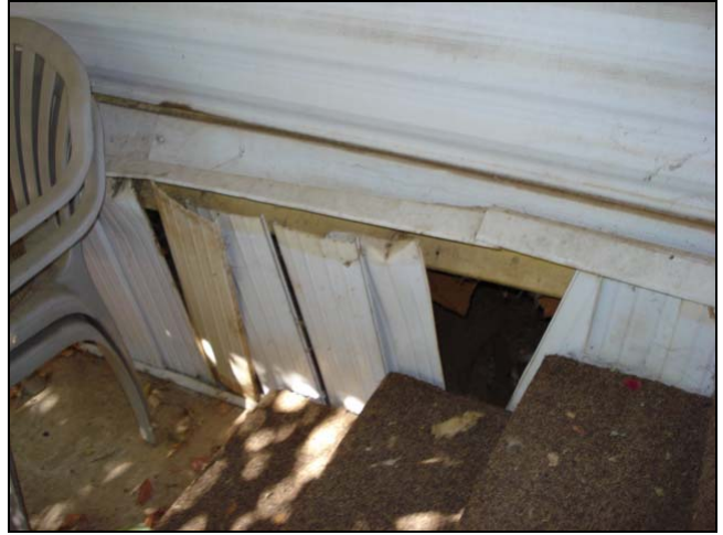
Loose metal skirting.
