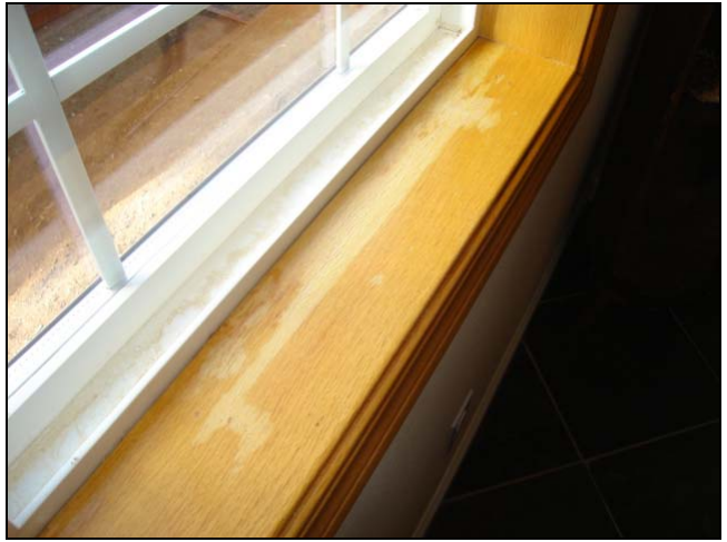
Stain in the sill possibly due to condensation.
