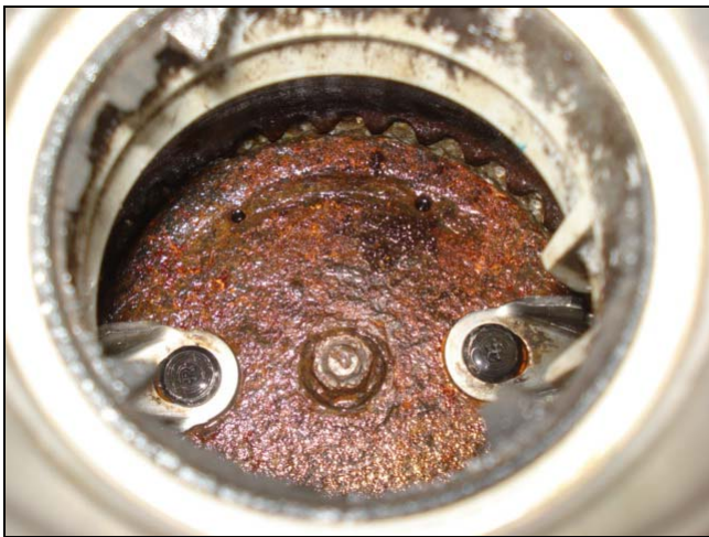
Wiped out weir gasket.
