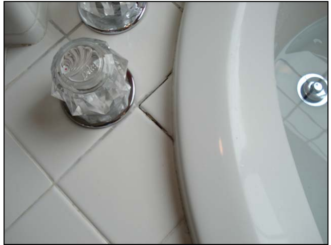
Missing tile grout.
