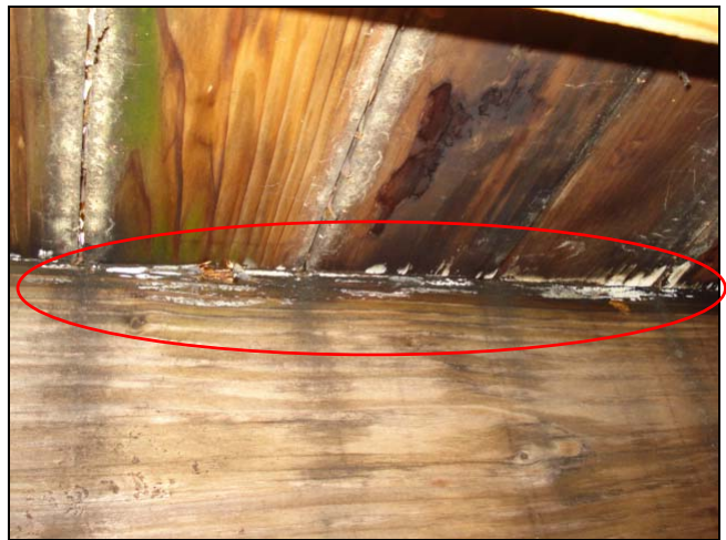
Possible fungus (organic growth) in this joist and the deck boards.
