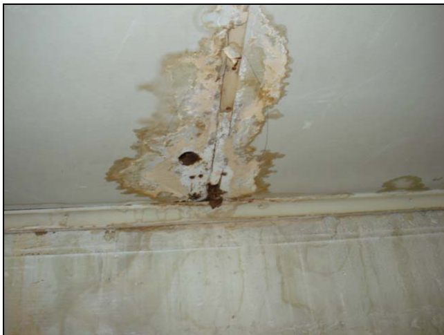
Severe stains and some deterioration.
