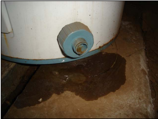
Drain valve leaking.
