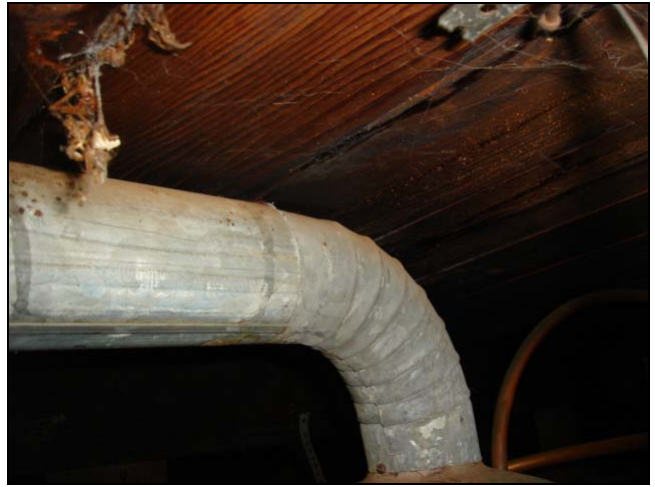
HAZARD: This water heater vent pipe has scorched the sub floor.
