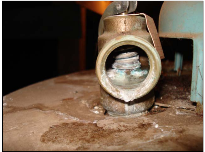
Leaking TPR valve with no pipe.
