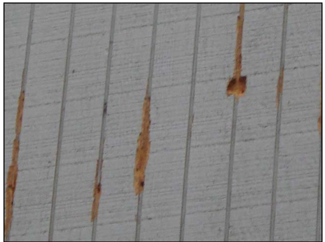
Wood pecker damage.
