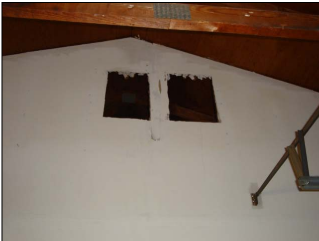
Access to the attic space. Such openings compromise the fire wall. Advancing fire will be drawn into this space directly over the living area.
