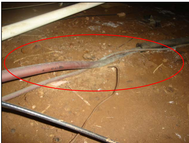
A/C liquid and high pressure lines should be lifted out of the soil and properly insulated.
