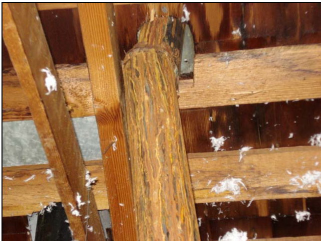
This kind of excessive rust on a flue pipe was a rare observation.
