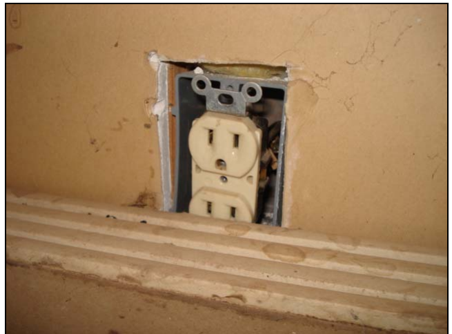
Are you kidding? Trim board installed over an outlet. How could this happen?
