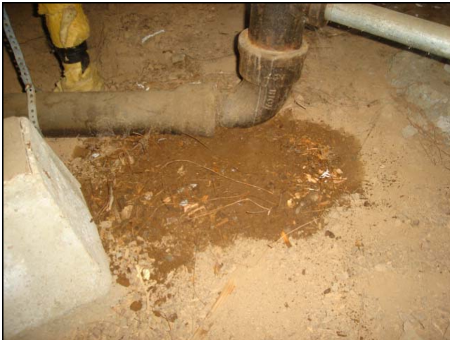
Wet spots in the soil beneath water and waste pipes is a good way to spot leaks.
