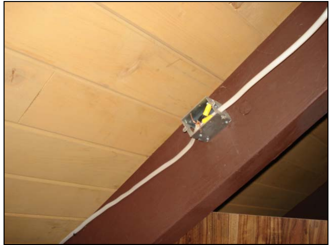
Open junction box, non utilized ground wire and exposed wiring at the beam of this cabin's loft.
