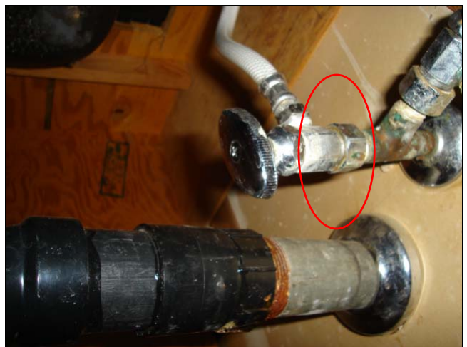
A leaking angle stop valve. Notice the ABS and galvanized waste line plumbing materials.
