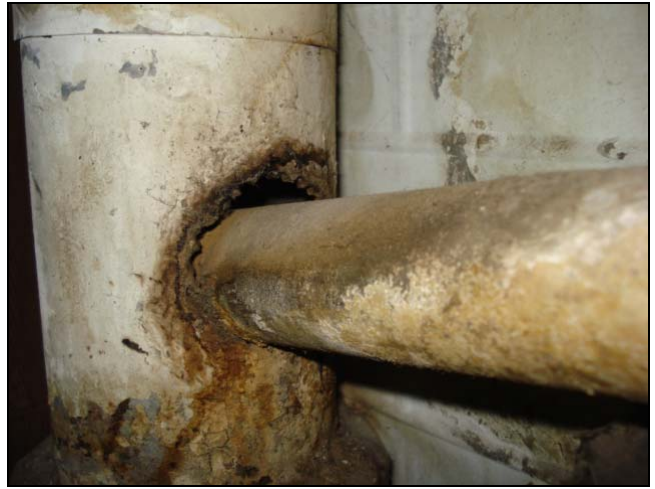
Someone cut a hole in this cast iron sewer drain to add this waste line.
