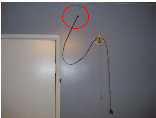
This extension cord was run through a wall and was plugged into the light fixture.
