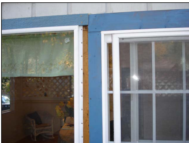
Missing window trim and caulking equals water intrusion and additional damage to inner walls.
