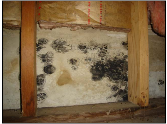
Possible mold. I have to say “possible mold” because I am not licensed or qualified to say that it is mold. This goes back to the information I gave you about how home inspectors have to use the proper verbiage to stay out of trouble.
