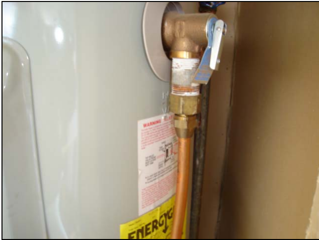
TPR with undersized drainpipe.
