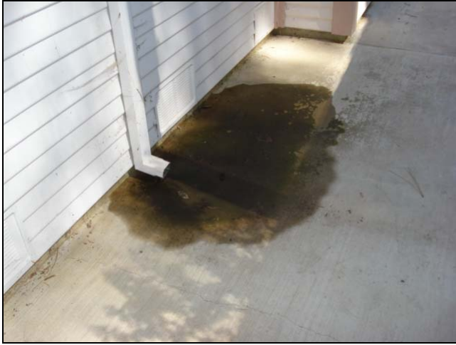
Standing water at a downspout.
