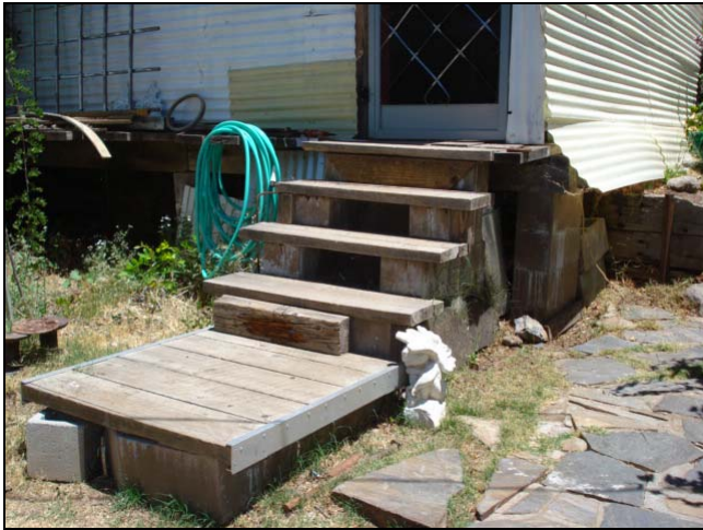
No railing for these 4 steps.
