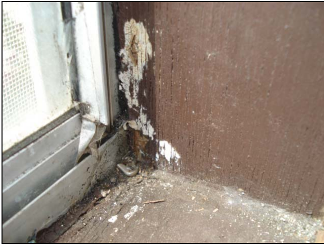
Organic growth and deterioration.
