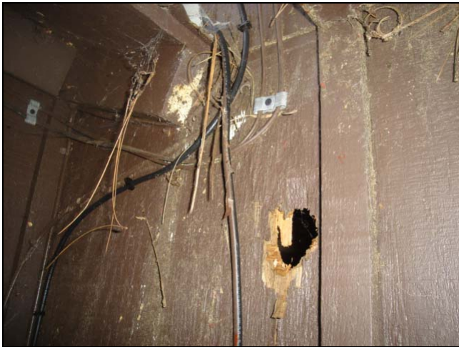
Wood pecker damage.
