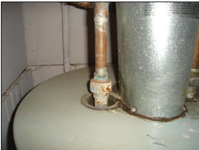
Water leak at the fittings.
