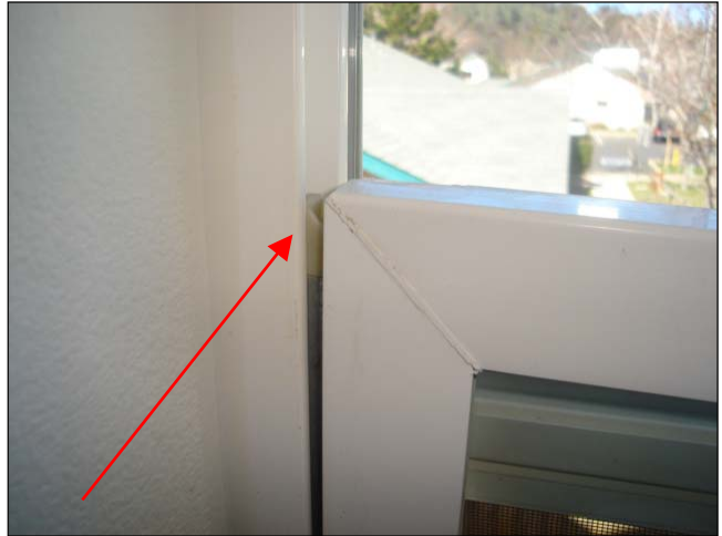
Window loose in the frame.
