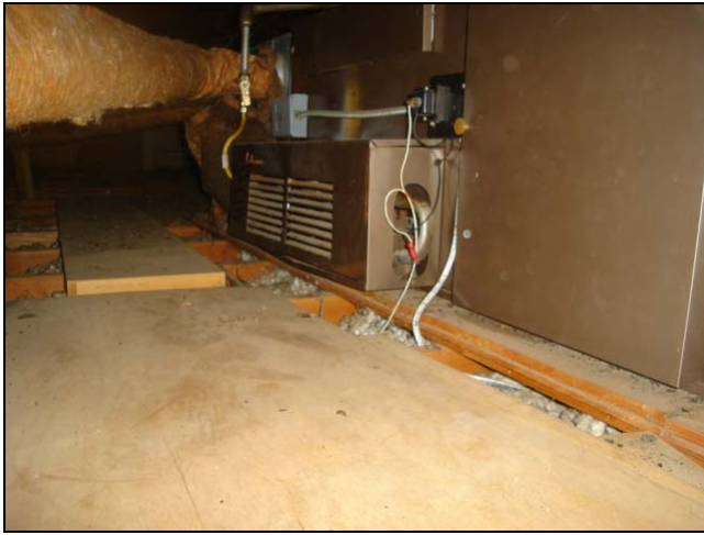
Furnace sitting directly on a plywood paltform.
