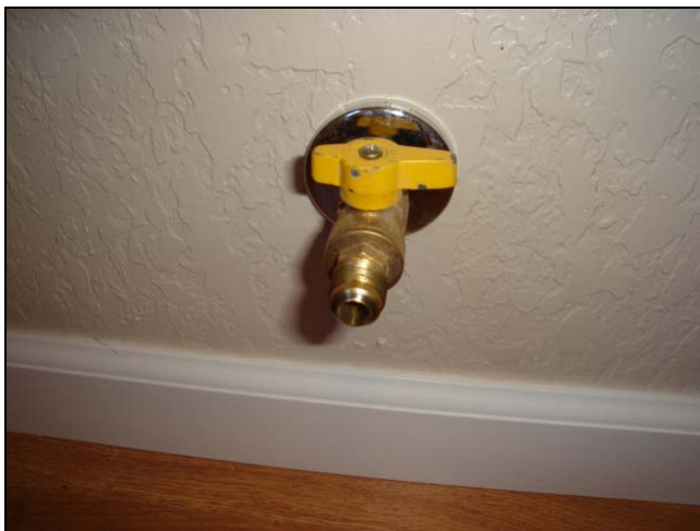
Missing gas vavle cap.
