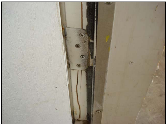
Cracked doorjamb at the hinges.
