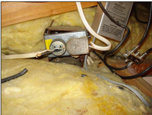
Electrical wiring being used as an extension cord.
