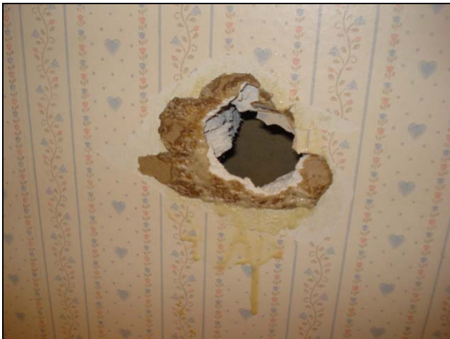
Doorknob damage in a bathroom.
