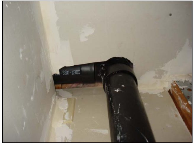
This plumbing pipe penetration compromised the fire envelope.
