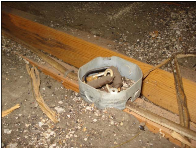
Open junction box.
