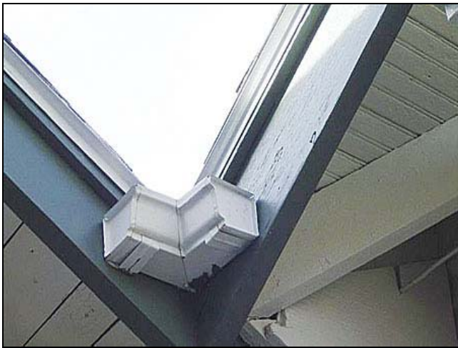
A goofy gutter.
