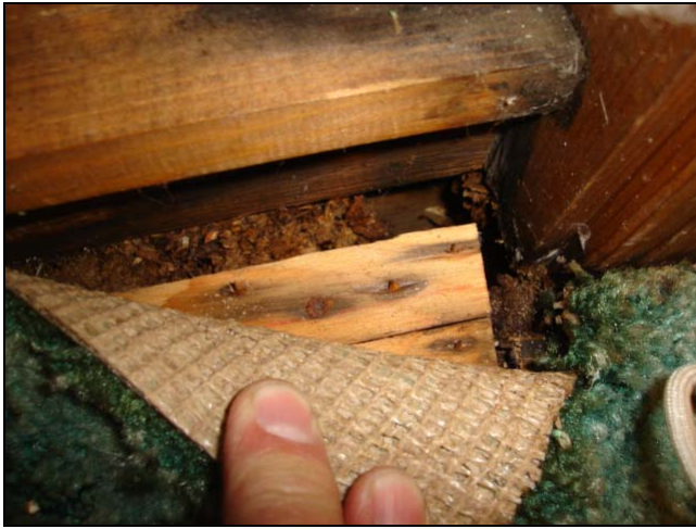
Soaked carpet and deterioration at an exterior door.
