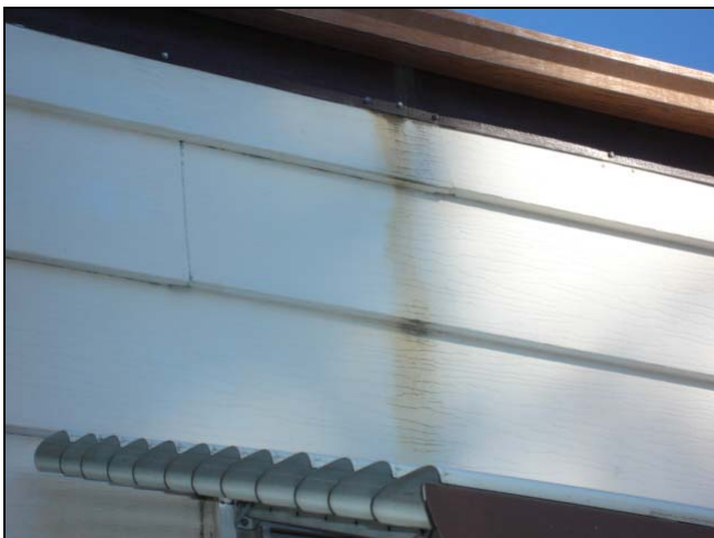
Vinyl stained from a leaking roof flashing.
