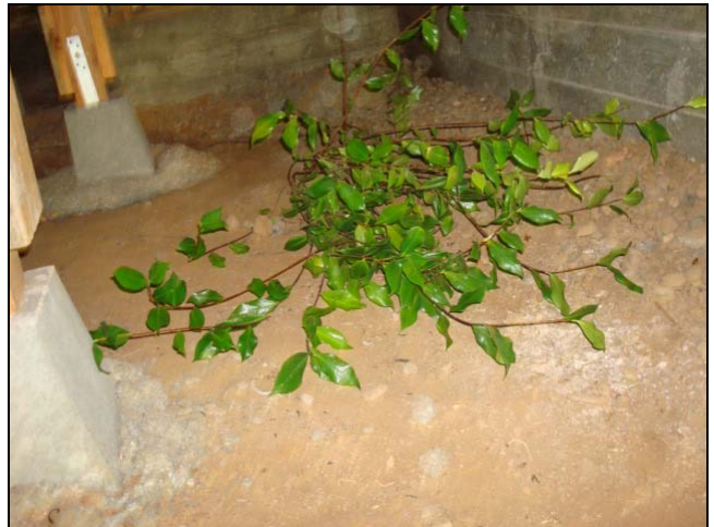
All those water leaks help the little plants to grow.
