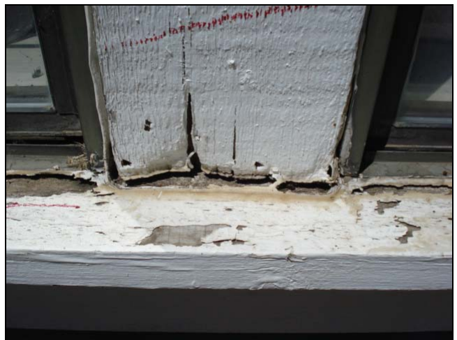
Trim damaged with a flat topped trim board underneath.
