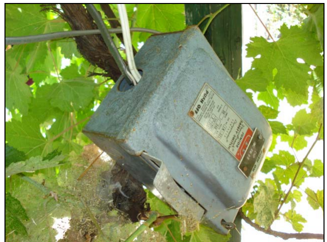
A very loose utility box.
