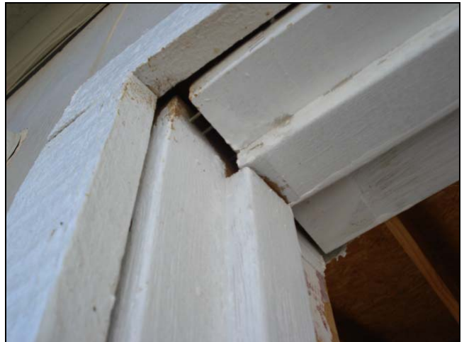
Jamb split open.
