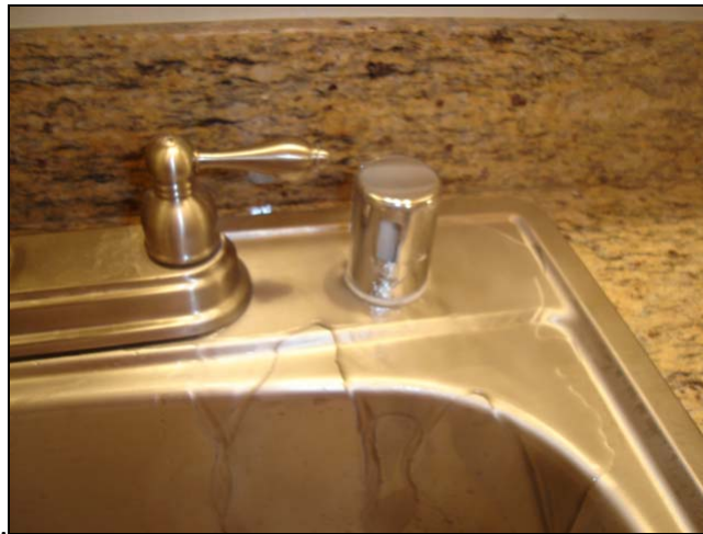
Water leaking out of the air gap fixture.
