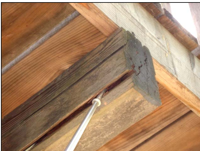
Decay in a beam.
