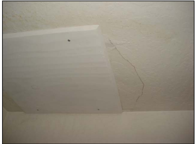
A stress crack at this ceiling patch.
