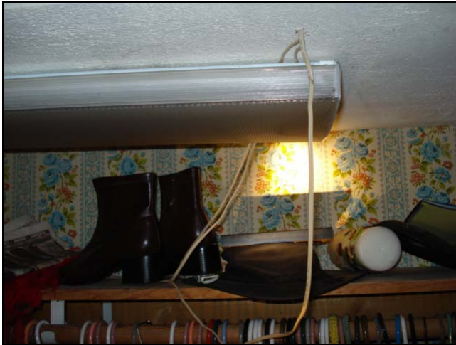
Interesting wiring configuration in this closet.
