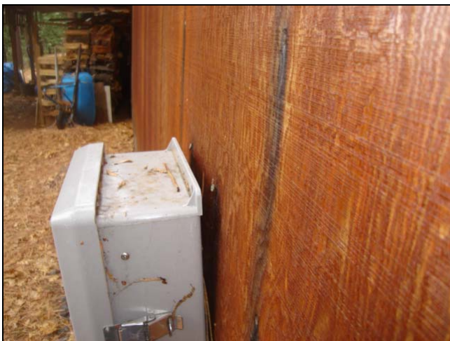
A loose utility box.
