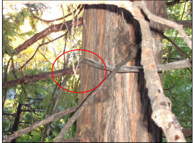
The tree branch is pulling the power line upwards.
