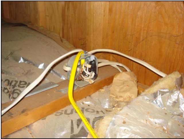
Open junction box. You know all about these.
