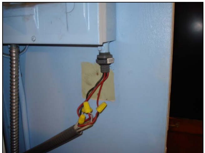
An open splice should be enclosed in a junction box.
