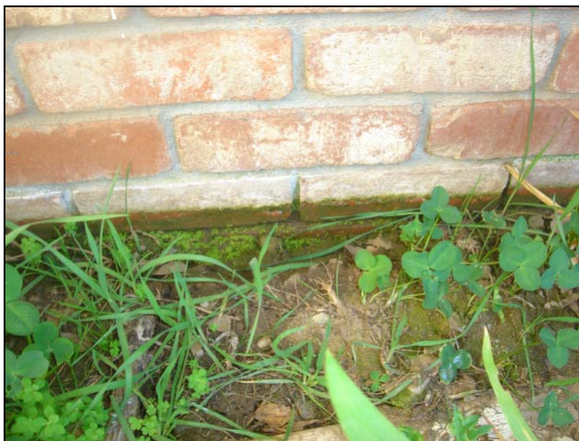
Brick wall wicking up moisture.
