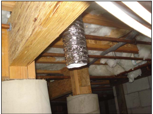
Dryer vent pipe terminates in the crawl space.
