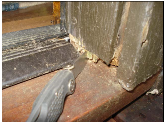
Deterioration in the jamb.
