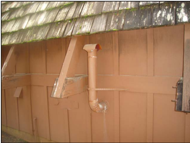
The flue pipe should not terminate under the eave.
