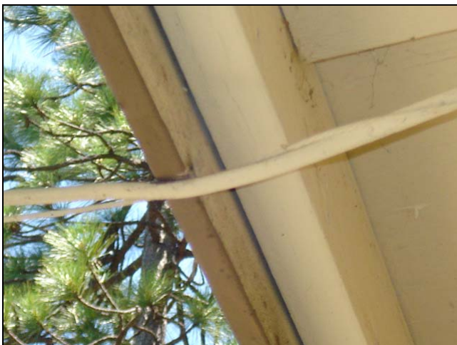
Exposed wiring rubbing against this fascia board.
