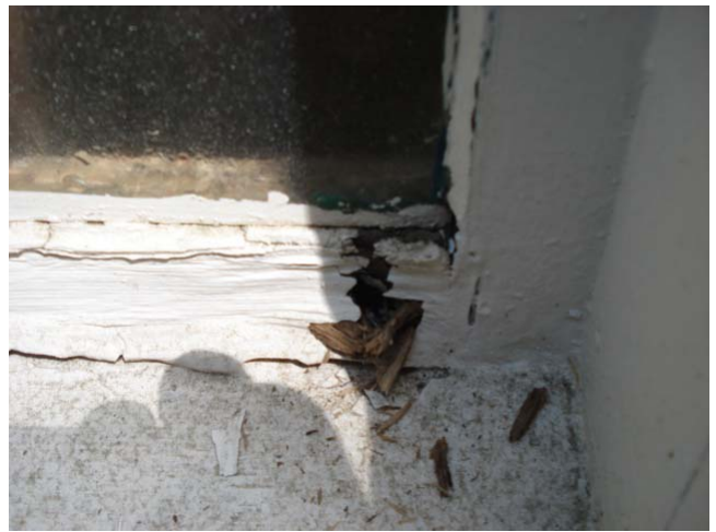
Wood frame deterioration, exterior.
