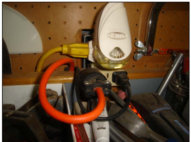
I know it's hard to tell, but there was a missing cover plate on this outlet junction box. I guess the air freshener was there to mask the smell of melting wires. Extension cords in use for permanent wiring too.
