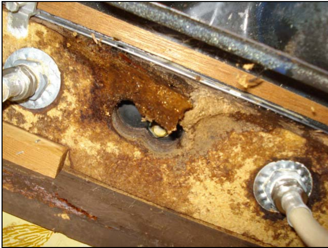
Deterioration under a kitchen countertop at the faucet connections. You have to look towards the faucet connections to see these problems.
