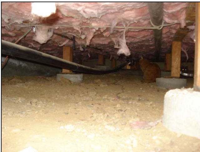
Sagging waste pipe.
