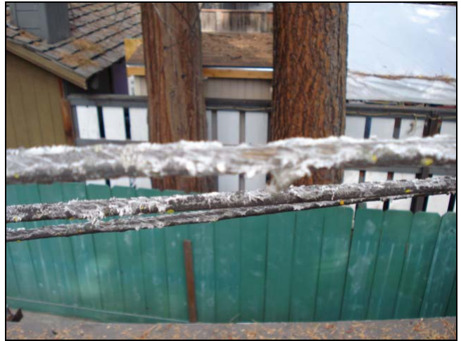
Frayed service drop wires.
