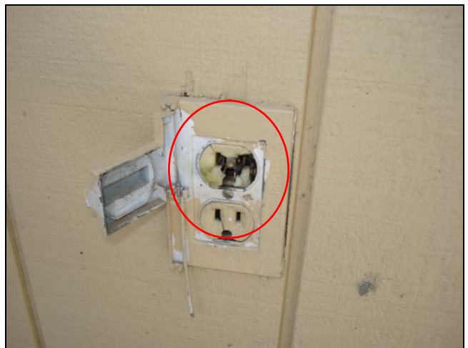
Very dangerous outlet.
