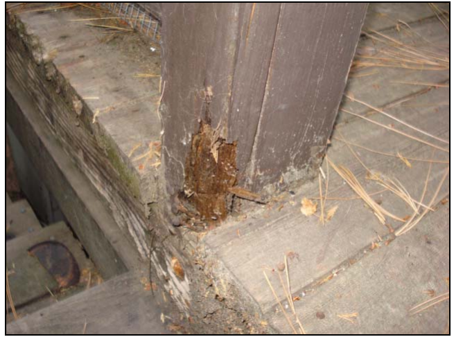
A deteriorated post.
