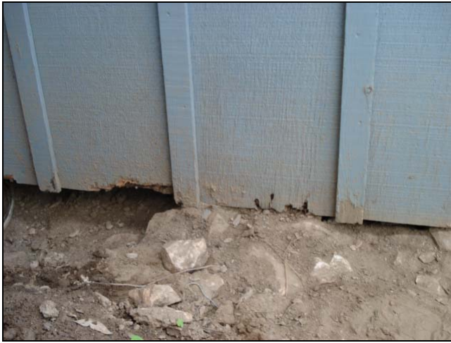
Note: Wood-to-earth contact and deterioration was noted at...
