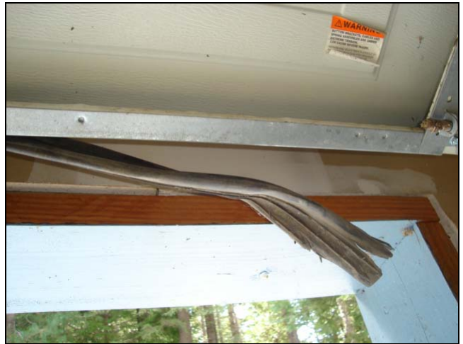
The failed door astragal seal.
