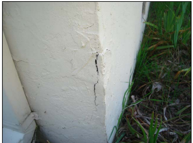
Cracked stucco corner will allow water intrusion.
