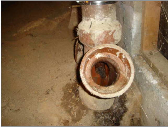
An open sewer pipe.
