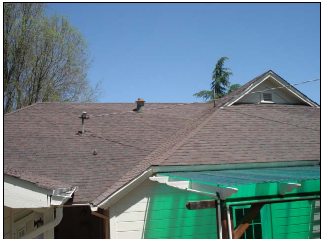
Service drop traverses a roof.
