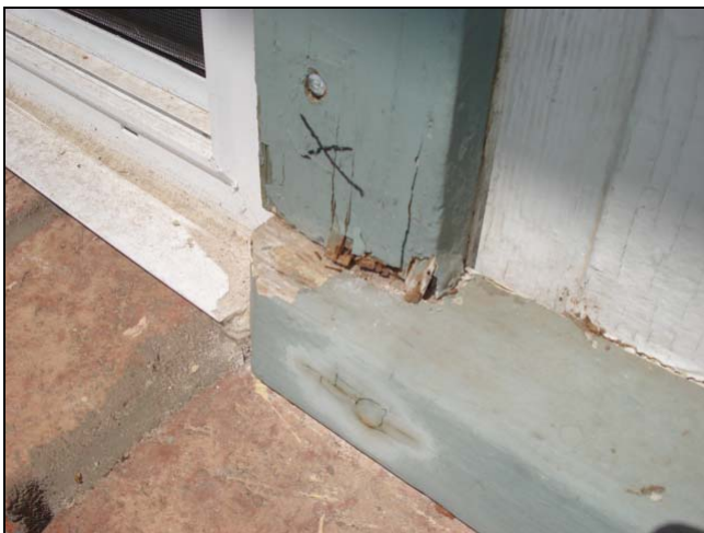
Trim damage. The ever common flat topped trim board.
