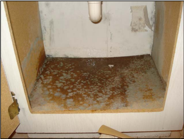
Severe organic growth under this sink from a water leak.
