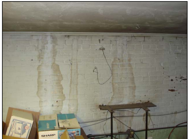
Masonry wall with water stains.
