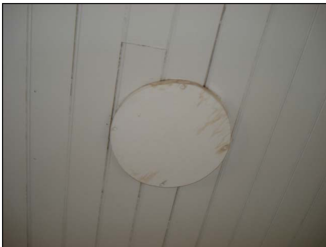
Patching for a former stove pipe.
