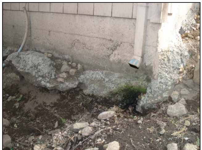
Erosion around the foundation footing.
