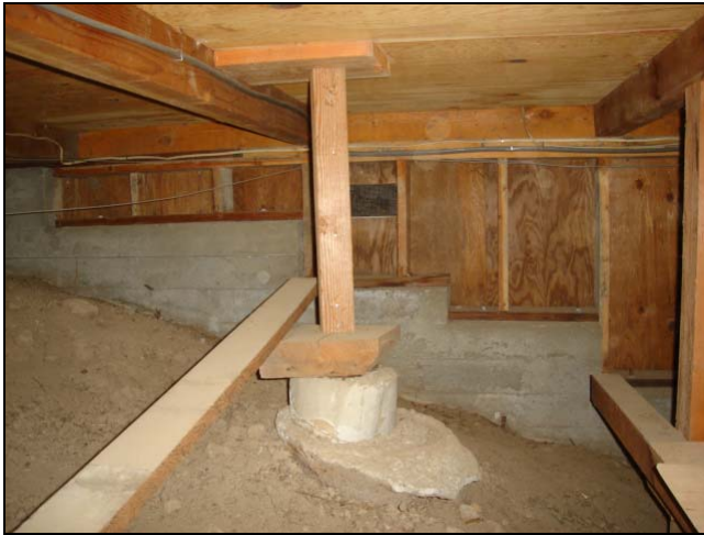
A make shift brace and severe erosion around this pier.
