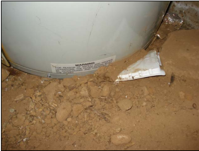
Dirt should be cleared away from the appliance.
