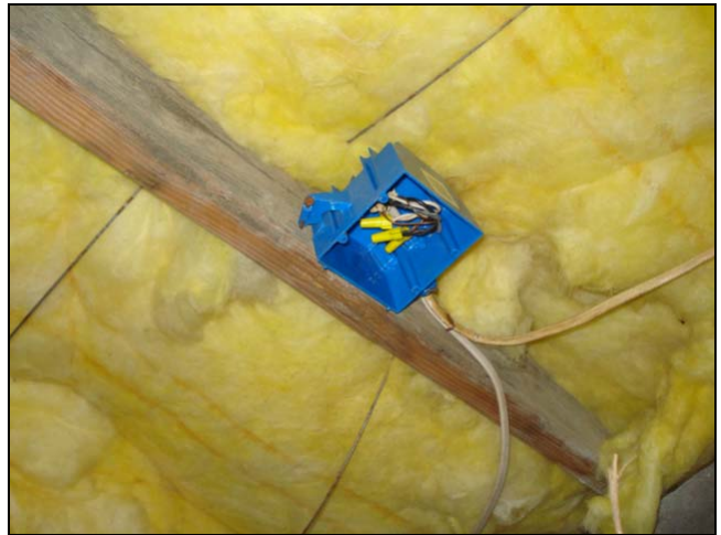
Missing cover plate on a junction box.
