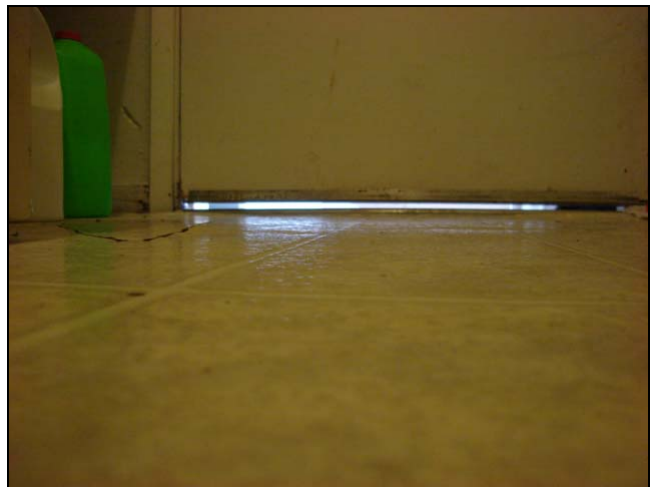
No weatherstrip at the door sweep.
