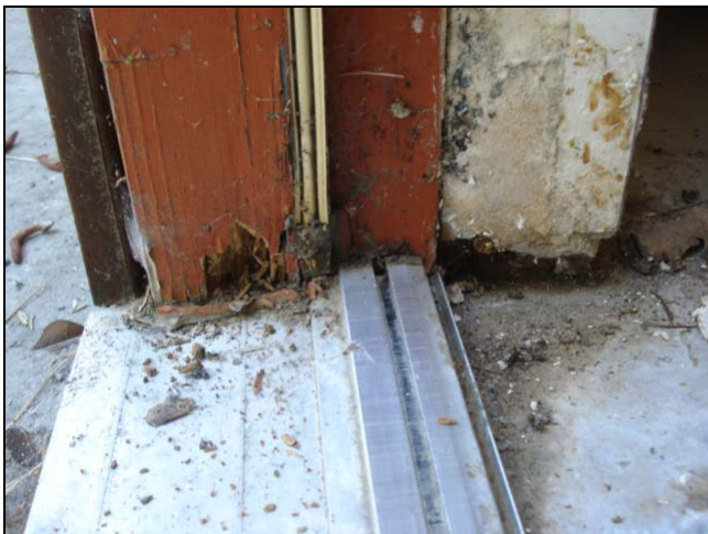
Deterioration in the jamb.
