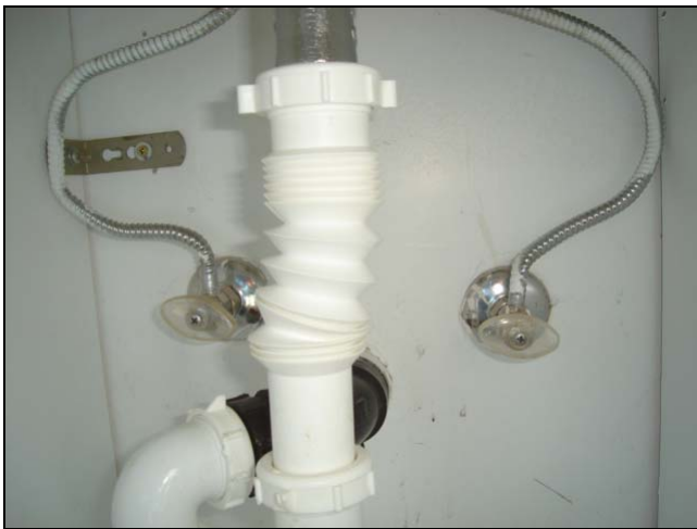
More corrugated plastic pipe.
