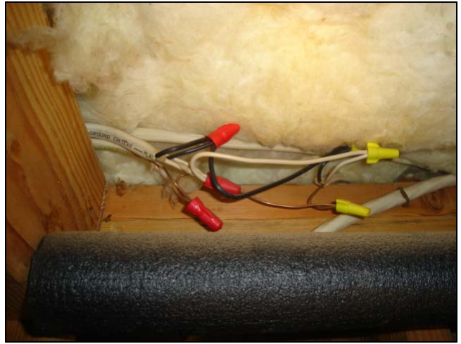
Open splice. There are usually more open splices in the crawl space than in the attic.
