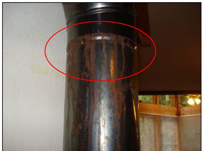
Here is what happens when the pipe is installed upside down. You can see how the upper pipe is slipped over the lower.
