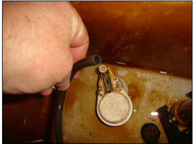
A loose bowl supply line hose was worn and could not be reinstalled.
