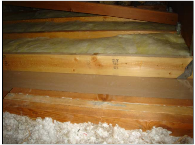
A combination of insulation material types was common. Here we see fiberglass batting and blown in cellulose. Missing insulation is noted.
