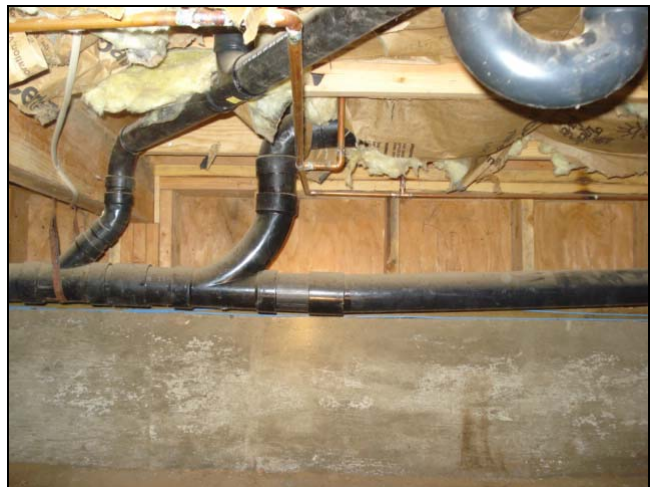
This low spot or "saddle" could become clogged with waste material. Plus water does not flow uphill.
