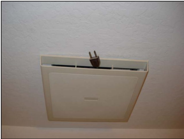
Note: The bathroom ceiling fan was not operable at the time of this inspection.
