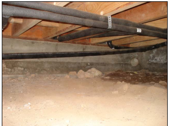
Water intrusion in a corner of the crawlspace. The ABS waste line needs more support as well.
