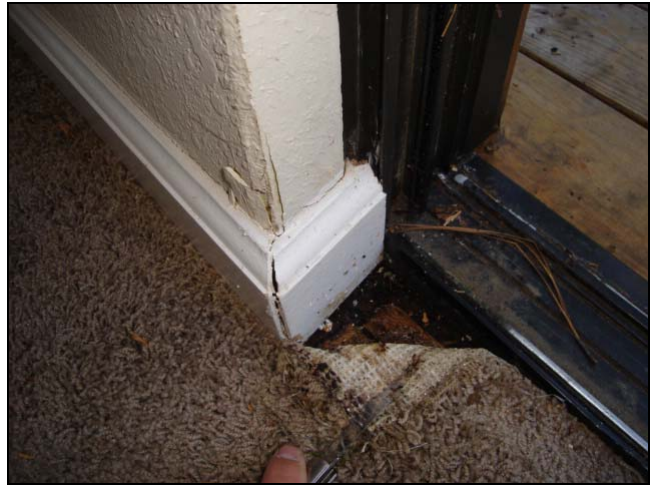
Soaked carpet and wet sub floor at a patio door.
