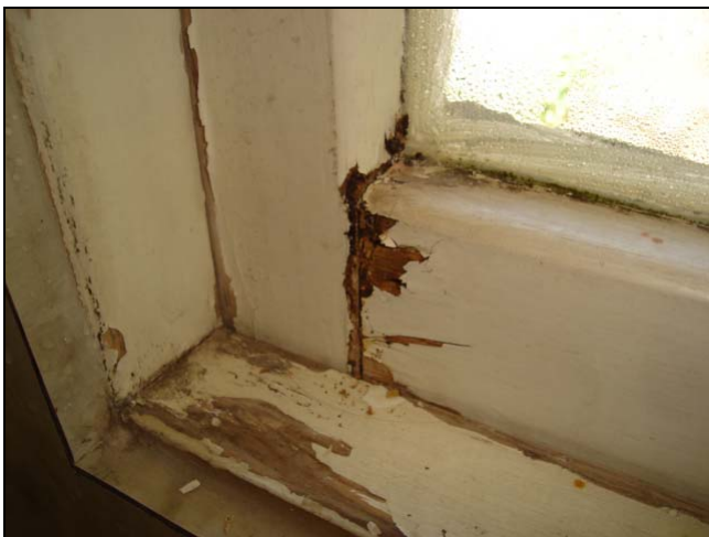
Wood frame deterioration, interior.
