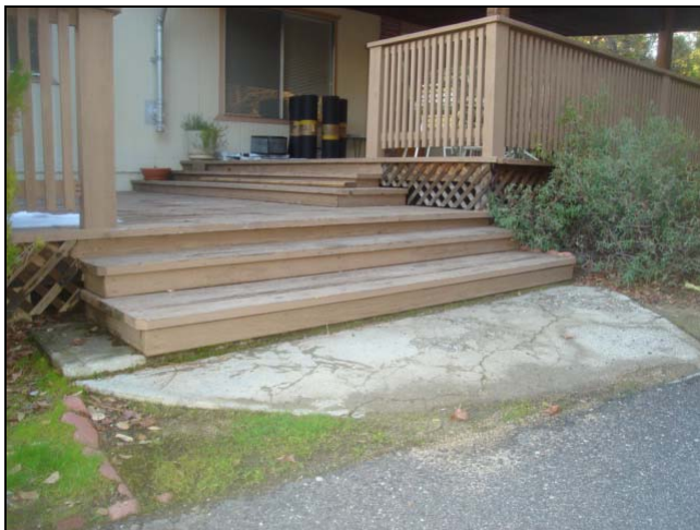
Uneven step height at several steps.
