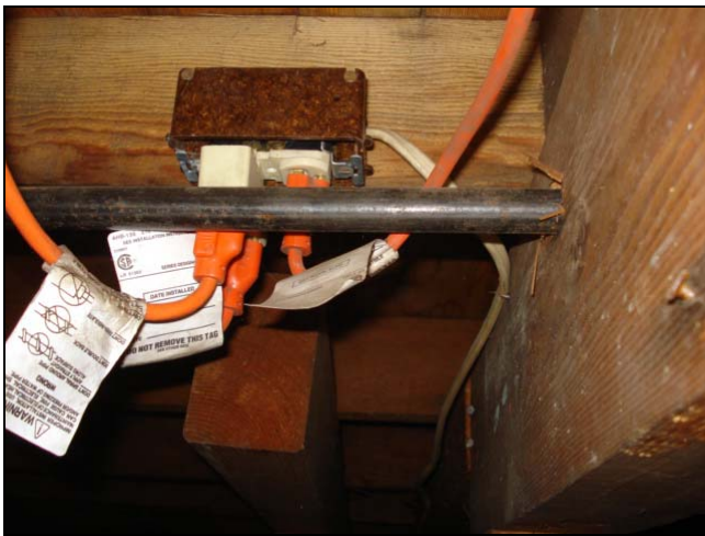
Extension cords being used as permanent wiring.
