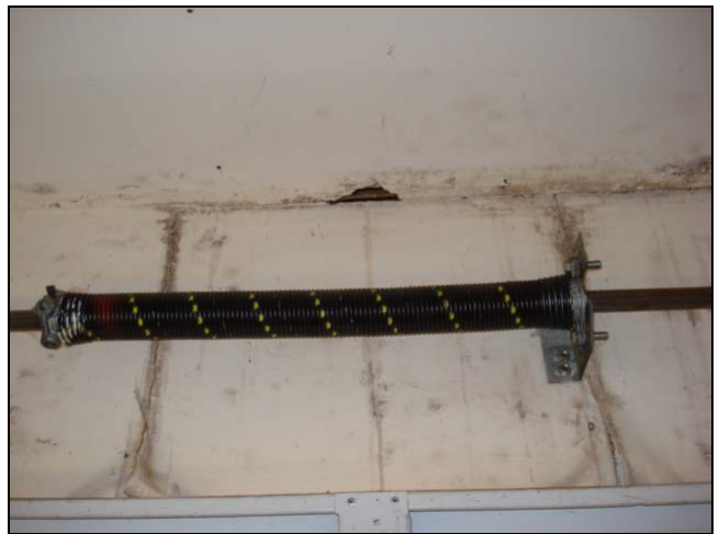
Some serious growth and deterioration where this garage roof had failed.
