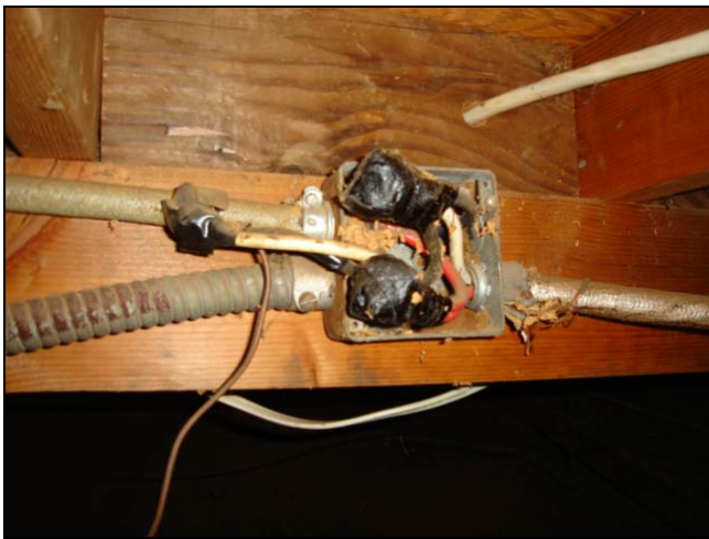
Ugly splices in an open junction box.
