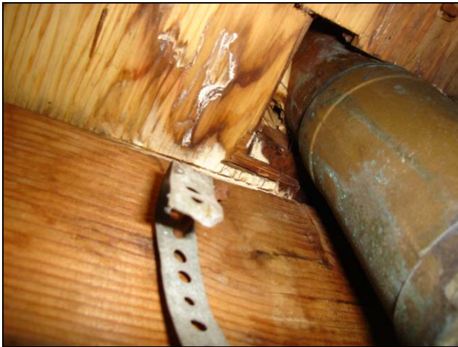
Evidence of a water leak under the toilet.
