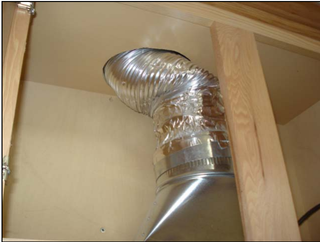
Corrugated vent pipe.
