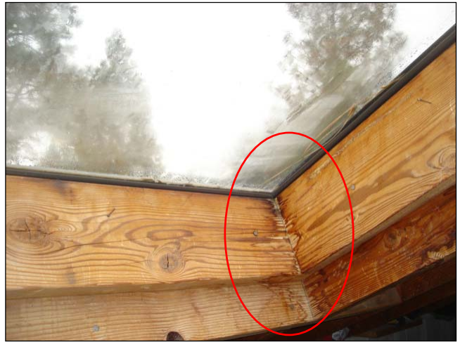
Skylight water stains.
