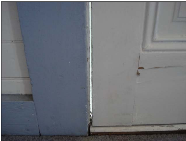
An air gap. Needs weatherstrip.
