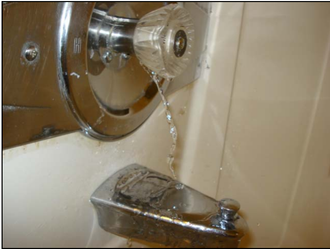
Leaking shower control valve.
