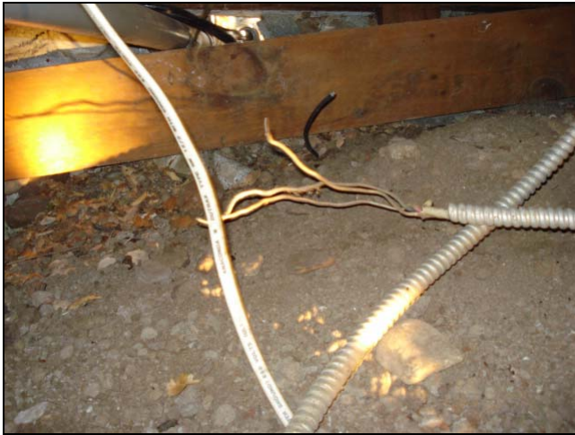
This wire was hot!
