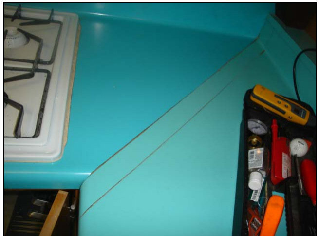
Mismatched laminate and swelling at a miter joint.
