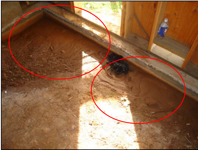
Evidence of flowing water.
