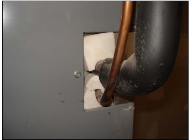
Air leaks around A/C lines again.
