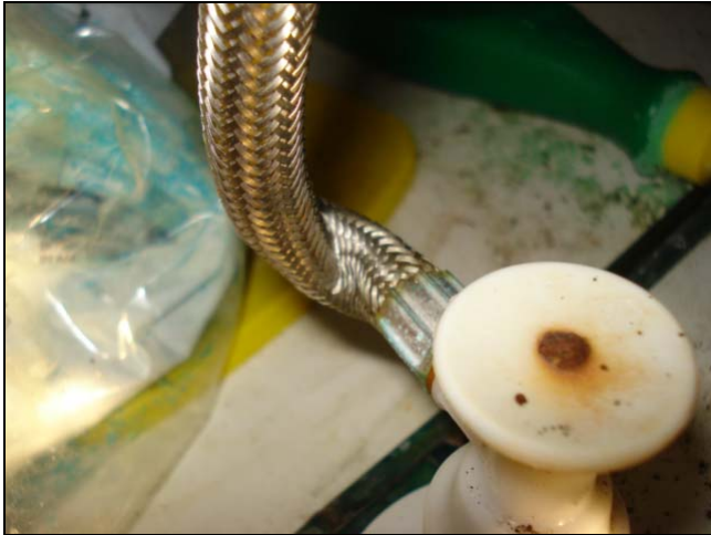
A twisted supply line. Probably will not be a problem but it should be corrected.
