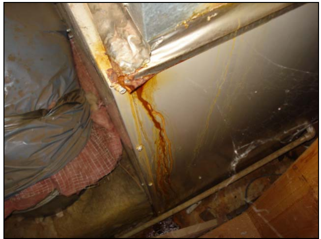
A condensate leak creates rust. That vinyl duct tape just couldn't hold it back.
