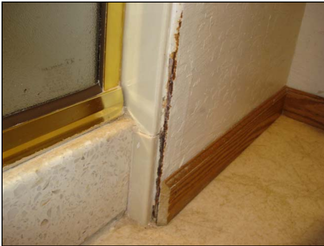
Deterioration at a shower door. The shower door leaked and water soaked into the wall.
