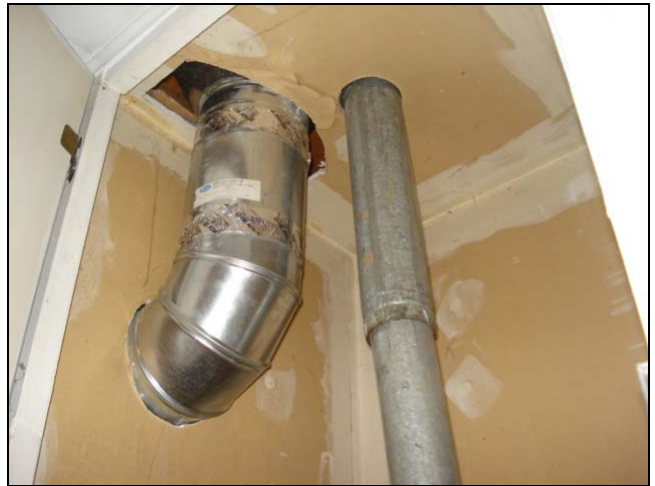
These vent pipes were not properly sealed where they passed through the firewall.
