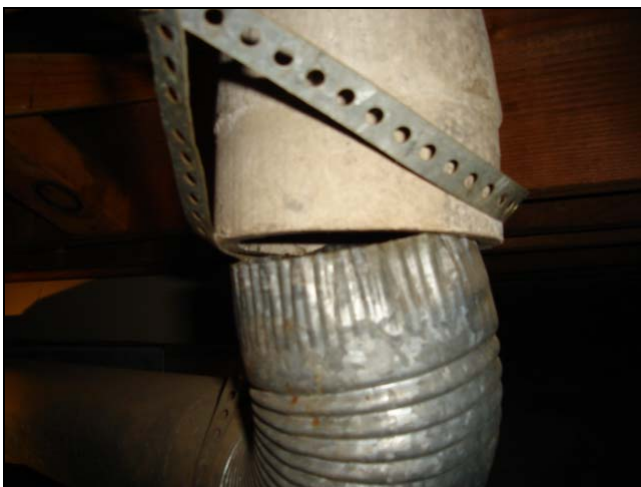
This loose stove pipe has come loose from an asbestos covered pipe. The grey colored upper pipe could be asbestos coated.
