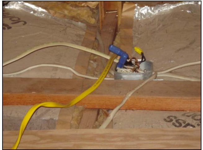
Open junction boxes are an automatic note. The box is designed to contain potential sparks and help arrest the spread of fire.
