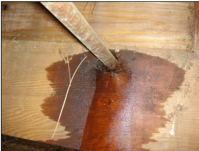
The copper water supply line split open inside this beam after a freeze.
