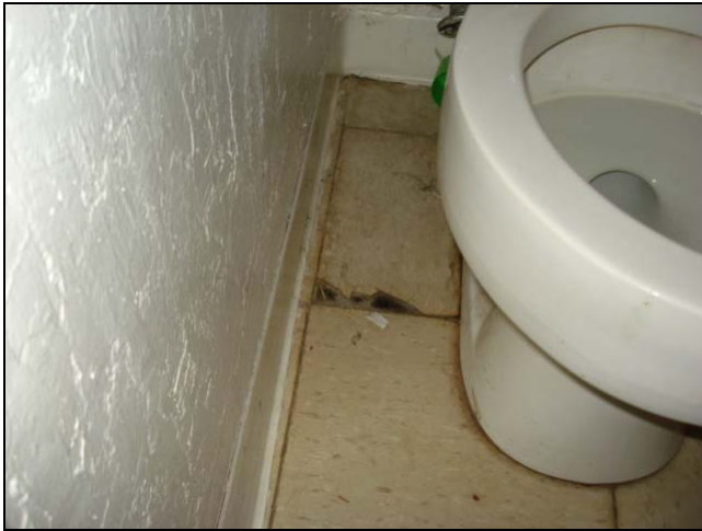
Water stains and chipped vinyl tile at the base of a toilet.
