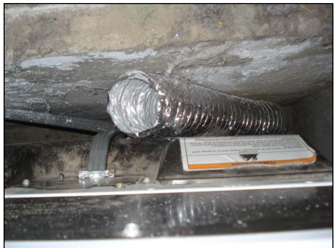
Disconnected vent pipe and lint build-up.
