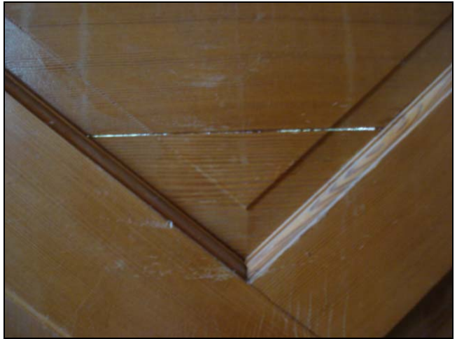
Crack in a raised panel exterior door.
