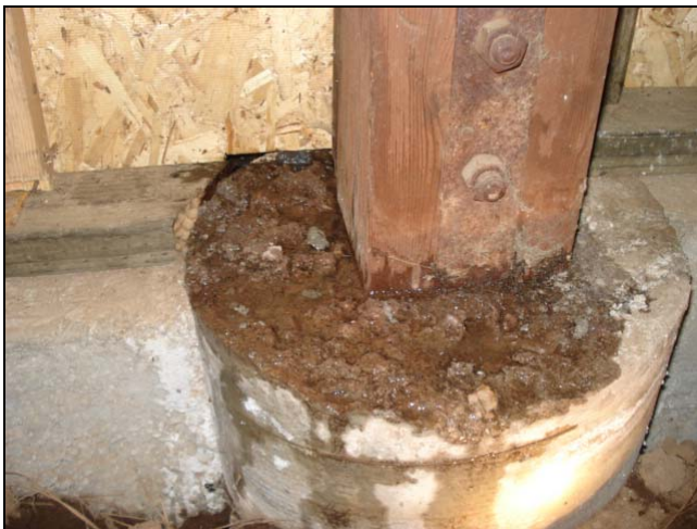
Water intrusion at a pier.
