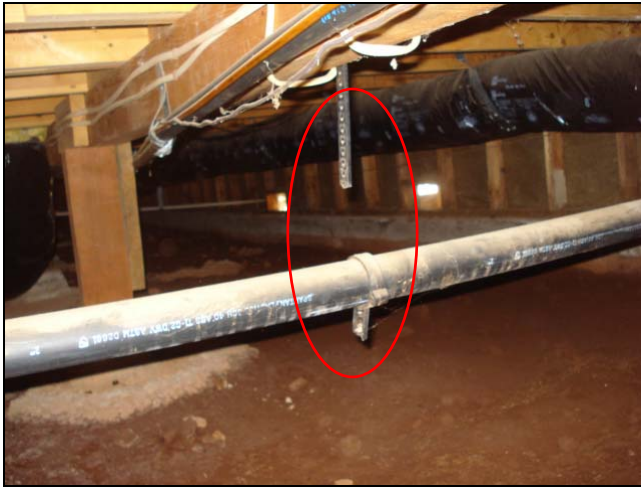
A broken waste pipe hanger.
