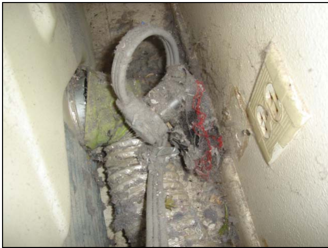
Excessive lint encased 220-volt outlet receptacle.
