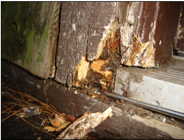
A deteriorated post.
