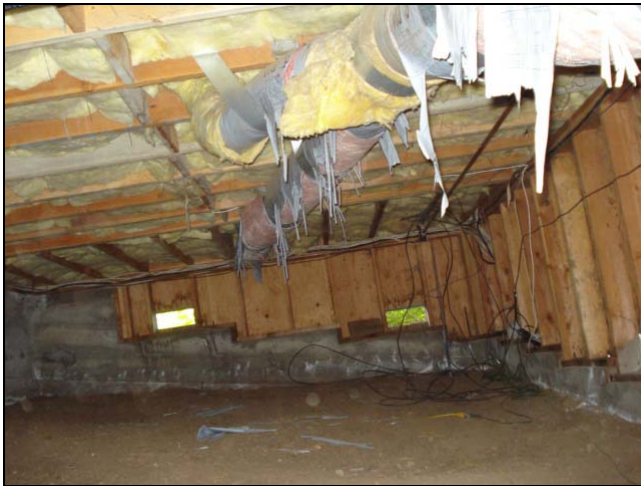
Shredded HVAC duct covering.
