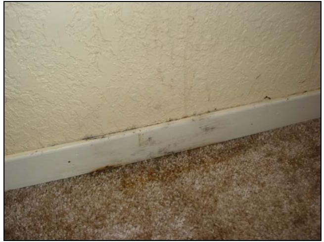
Water stain and possible mold where a window was left open.
