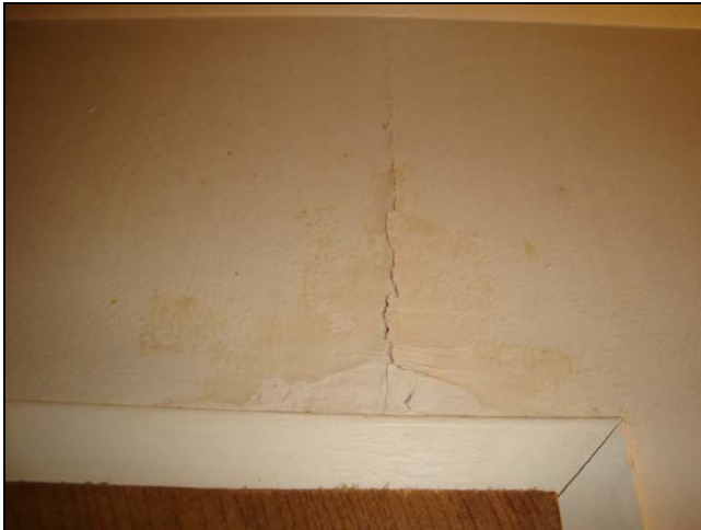
A settlement crack.
