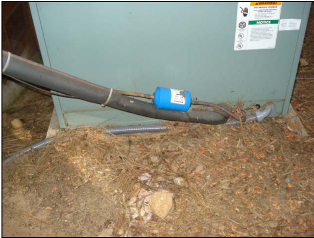
Leaves and debris collecting around an A/C condenser.
