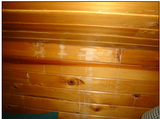
Old water stains appear to be “bleached.”
