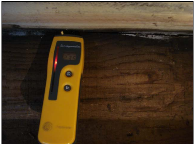
A red light on this moisture tool indicates an active water leak.
