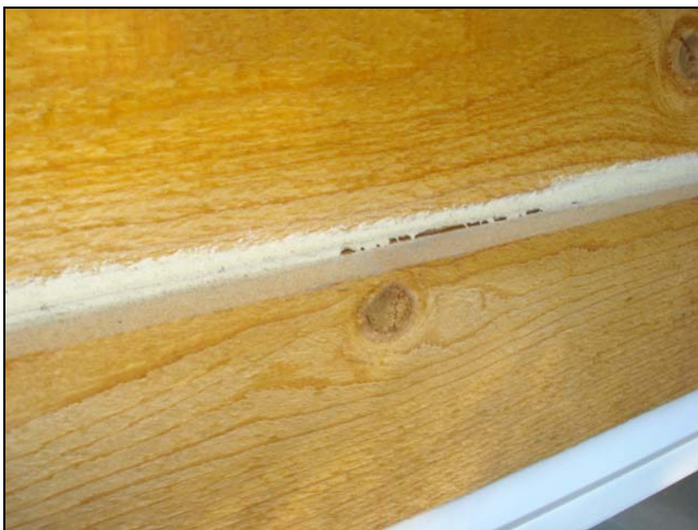
The caulking has pulled loose over this window on a brand new cabin home.
