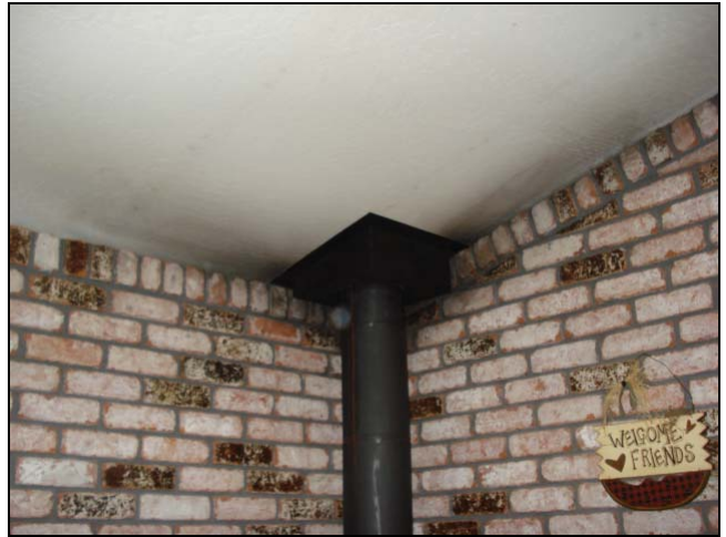
Soot on the ceiling indicates a severe combustion leak into the living space. This is a HAZARD .
