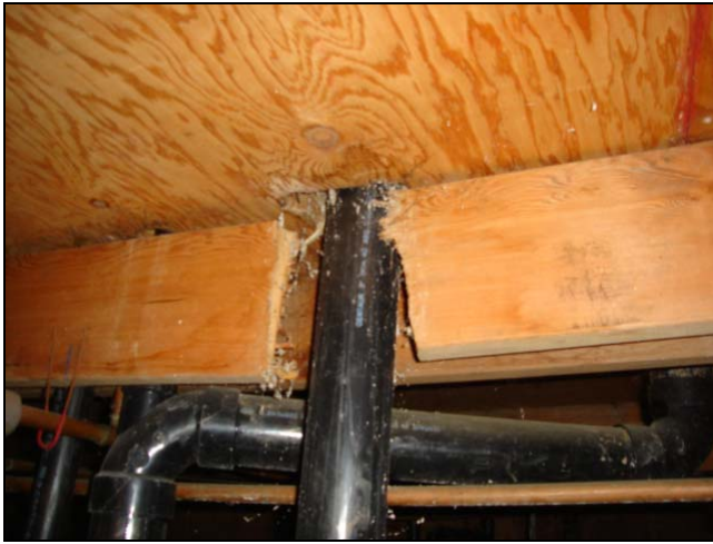
Compromised joist. Looks like this one had a sistered joist behind it however.
