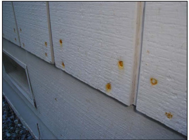
These rust stains are a tell tale sign of moisture behind the wall. I understand the termite contractor bid $40,000 to repair the damage in the siding of this building.
