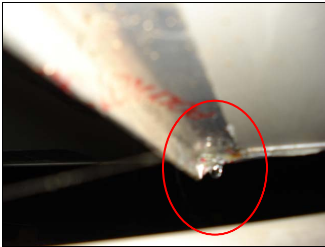
Water dripping out of an evaporator housing. This moisture should be routed to the exterior of the building.
