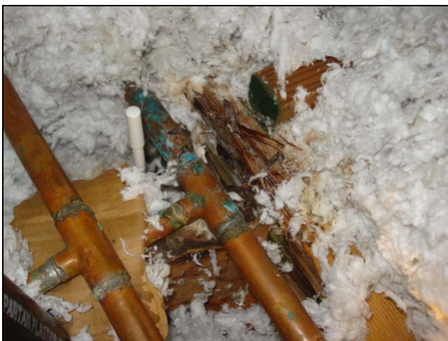
A leaking copper water pipe. These attic pipes can be subject to freezing. When these split open, it's a big mess.
