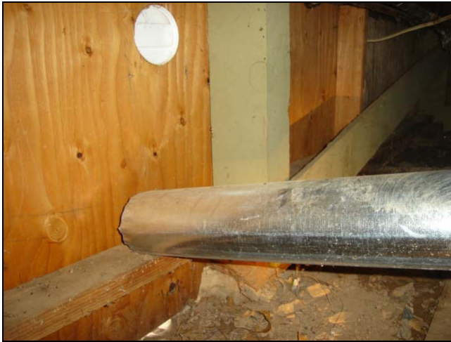
The dryer vent pipe has fallen loose from the diverter.
