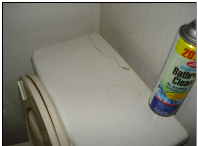
Cracked toilet tank lid.
