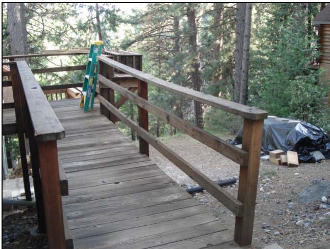
"Ladder" style rails.
