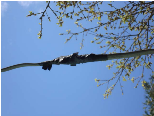
Open air splice.
