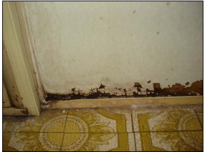
Severe deterioration and possible mold at this laundry room wall.
