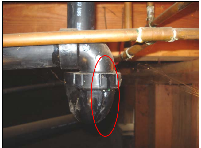
An active water leak.
