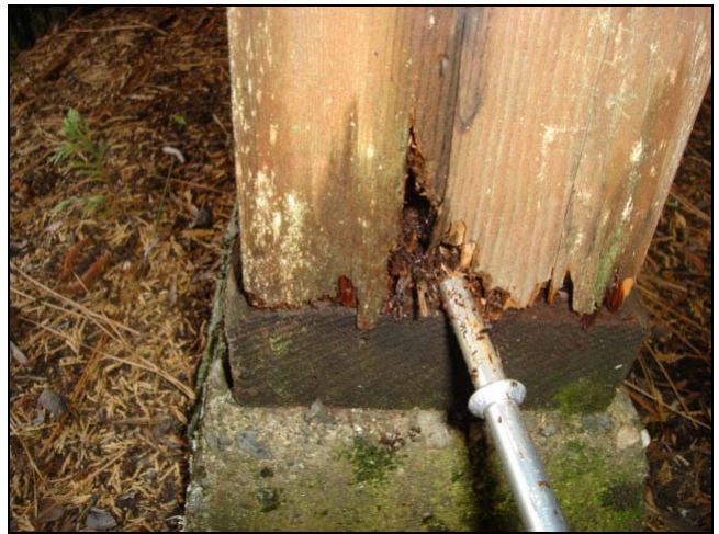
A deteriorated post. A ski pole makes a great probe tool.
