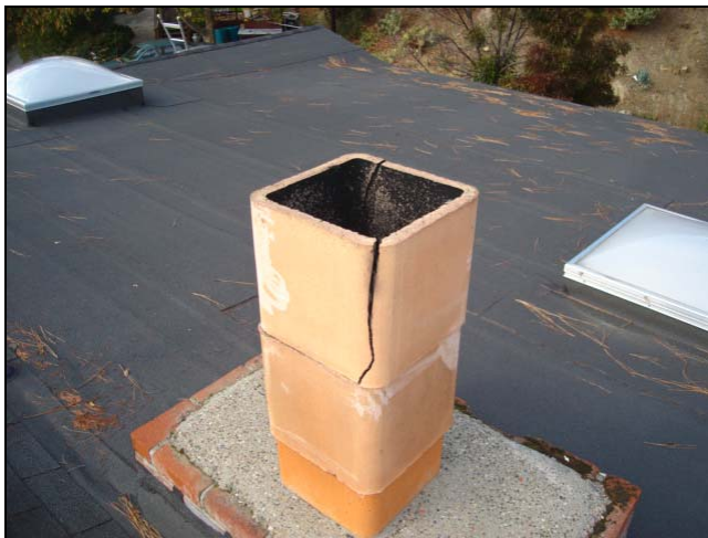
Cracked tiles and no spark arrestor.
