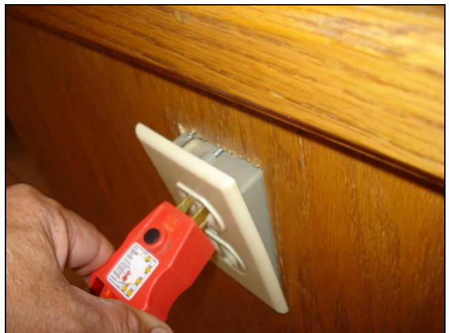
Loose junction box.
