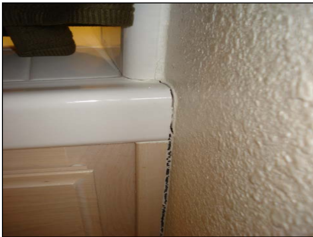
Cabinet pulling away from a wall. These reason for this problem can be very complicated. Call for information if this is your issue.
