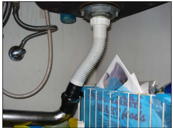
Corrugated plastic pipe and electrician's tape do not comply with modern building standards.
