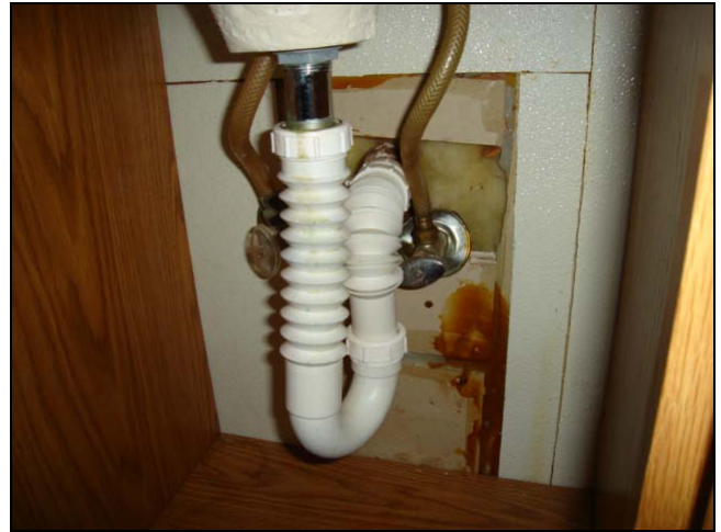
Corrugated plastic pipe is not a proper material for this application. The drainpipe should have a smooth continuous inner surface.
