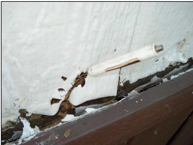
Severe deterioration in this hardbord material. Notice the flat topped trim board.
