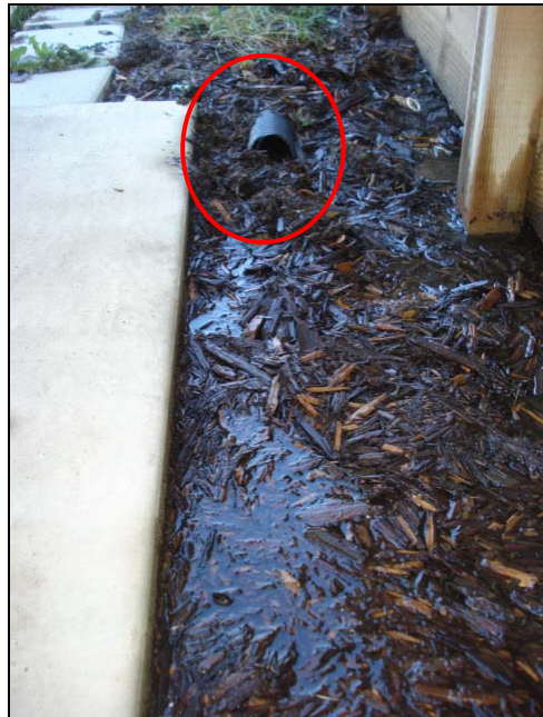
This drainpipe did quite reach far enough to make it to lower ground.
