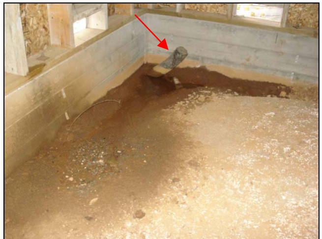
Standing water in a corner of the crawlspace. Maybe they should shorten that drainpipe in the corner.
