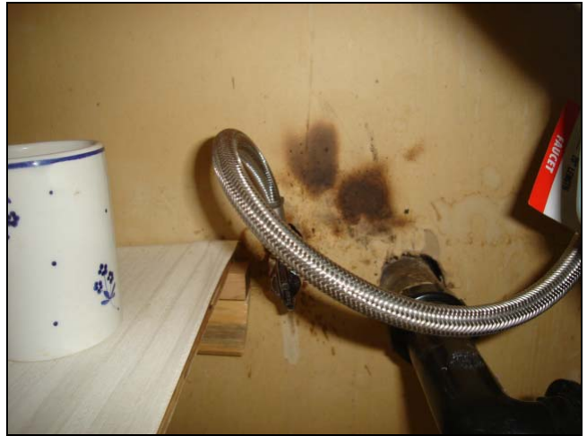
Scorch marks under a bathroom sink. Not a problem, just unsightly.
