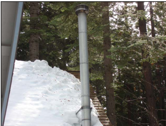
This pipe should have additional bracing installed.
