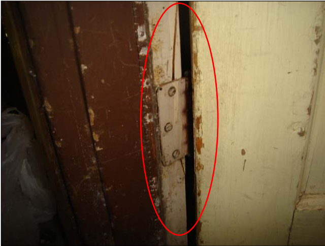
Cracked doorjamb at the hinges.
