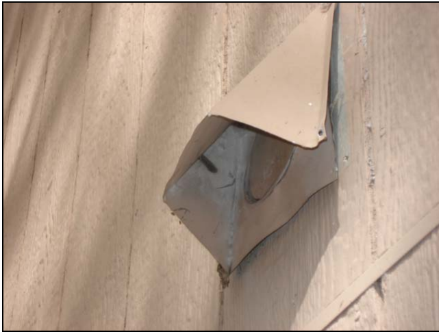
Loose diffuser cover.
