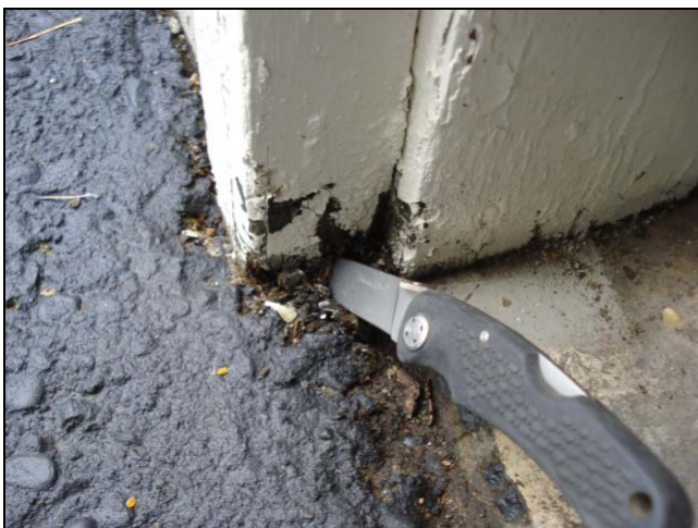
This type of damage at a garage big door trim is common.
