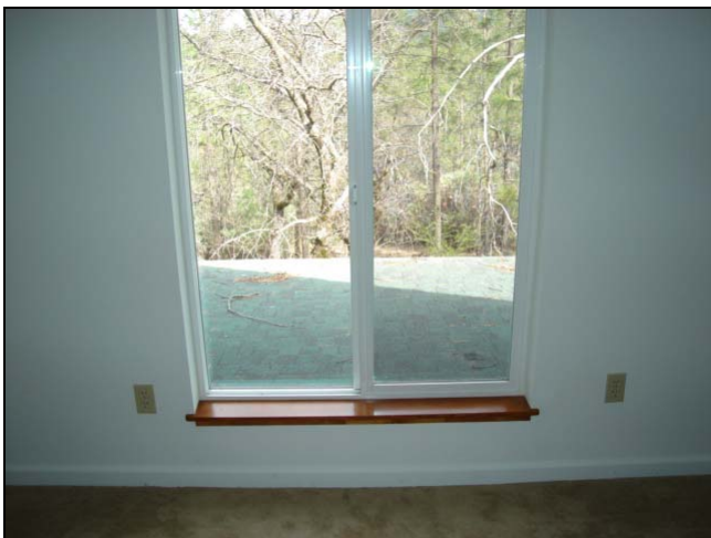
Low proximity to the floor. Tempered glass required.
