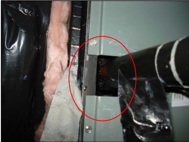
Loose tape created a massive air leak in this unit.
