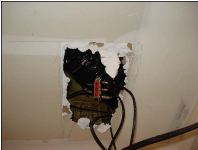
This cable TV installation compromised the firewall.
