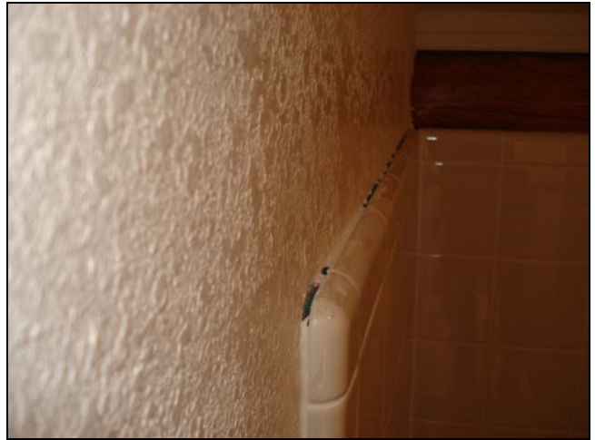
Gaps in the caulking at the top of the shower should be sealed. This may have been picked up while you were inspecting the walls.
