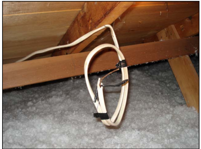
Non-terminated wire. Was it hot? Who cares! It should be properly terminated or removed.
