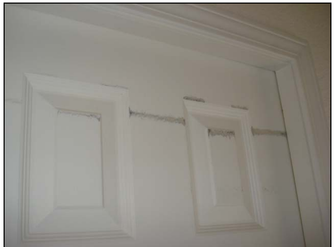
A scuffed pocket door. The door drags at the inside of the frame.
