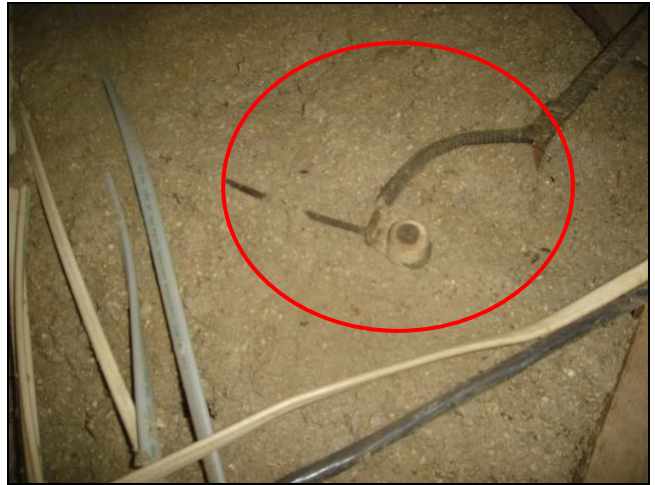
If knob and wires are in use, they must not be covered with insulation.
