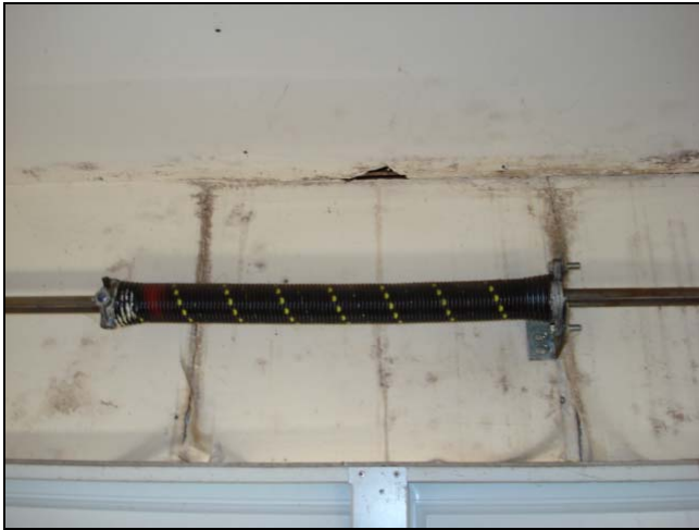
Possible mold and deterioration in a garage due to a leaking roof.
