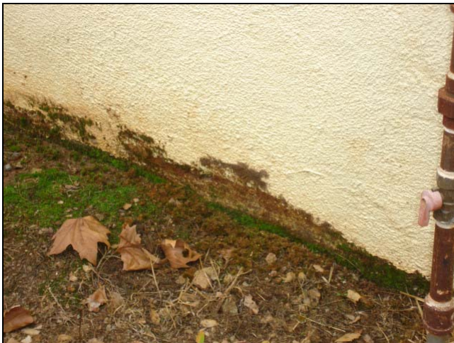
Classic old time application. Stucco travels down the wall and foundation below the grade.
