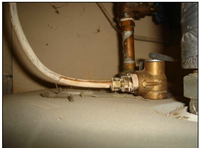
TPR with undersized drainpipe that should slope downwards. The discharge pipe should match the size of the TPR valve.
