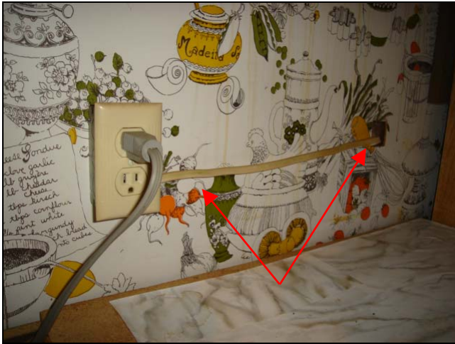
A tap into the back of an outlet to power something in the wall. Not good.
