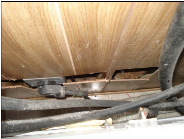
Cut outs in the paneling behind the washer and dryer.
