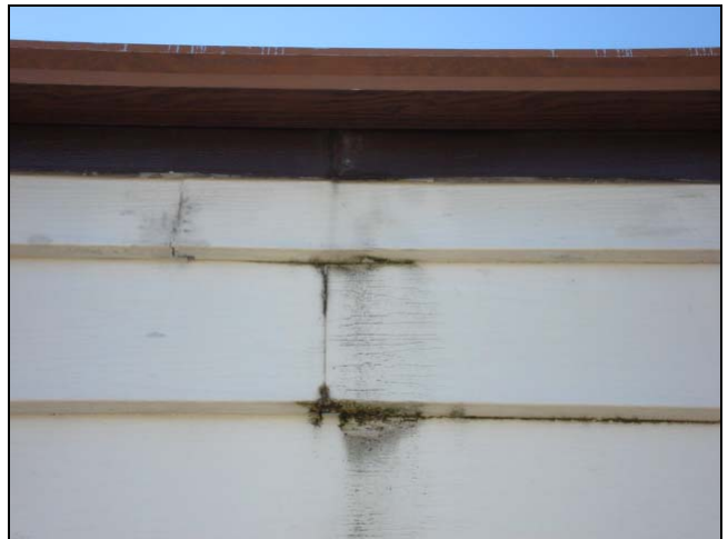
Vinyl stained from a leaking roof flashing.
