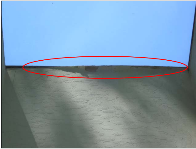
Peeling paint in a skylight
