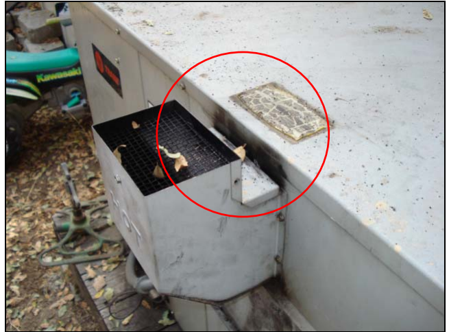
Soot at the exterior of the package unit furnace housing.
