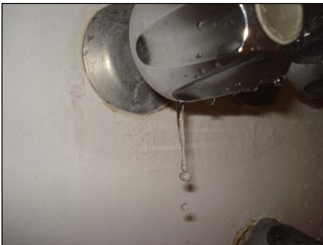
Leaking tub control valve.
