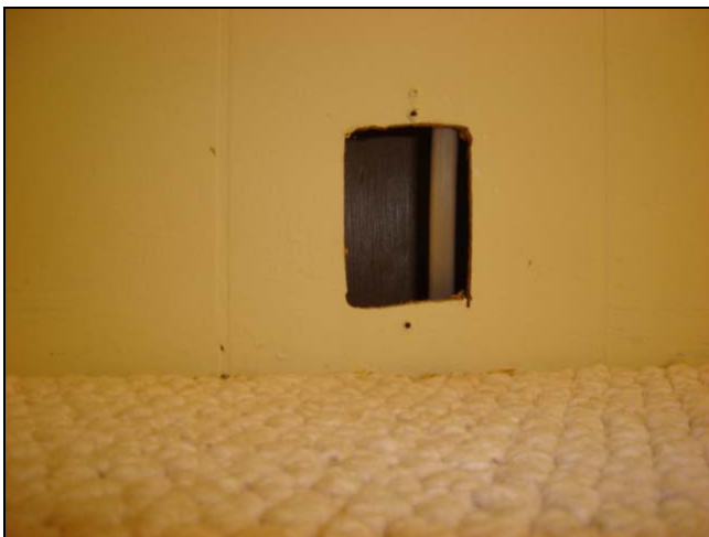
A hole in the paneling.
