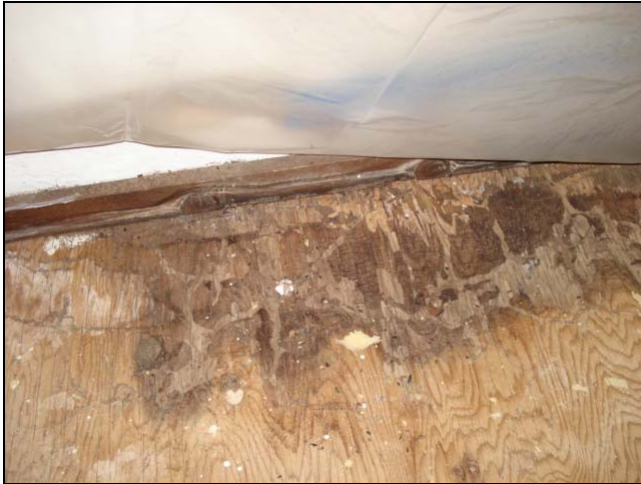
Water intrusion in the plywood subfloor at a patio door.
