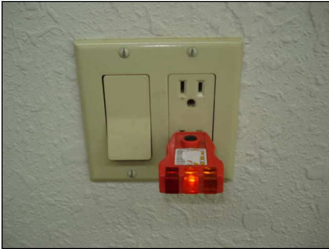
This indicates an Open Ground condition.
