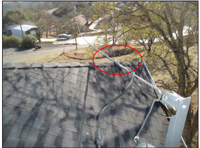
Service drop is physically touching this roof.
