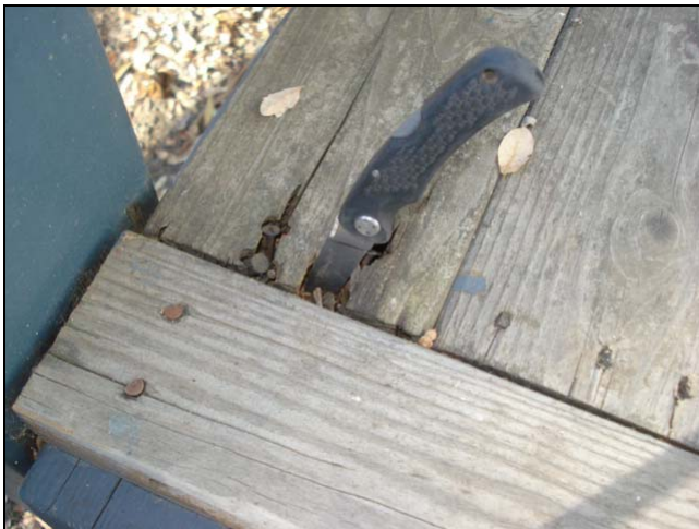
Deteriorated deck board.
