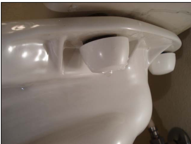
Moisture dripping off the toilet connections due to condensation.
