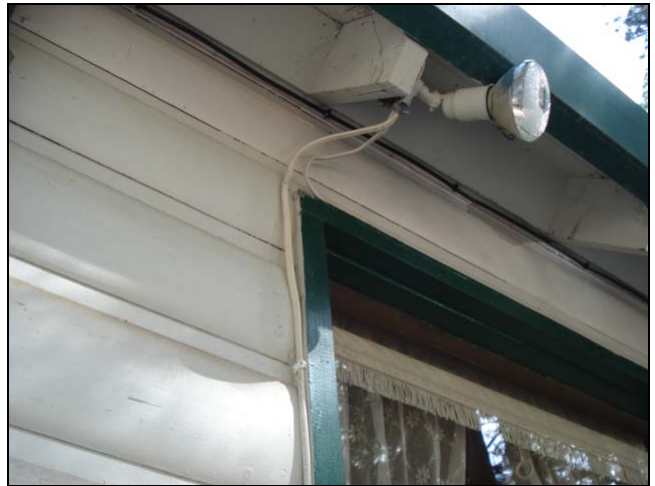
Exposed wiring at an exterior light fixture.
