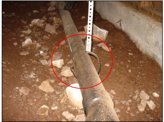
A loose waste pipe hanger.
