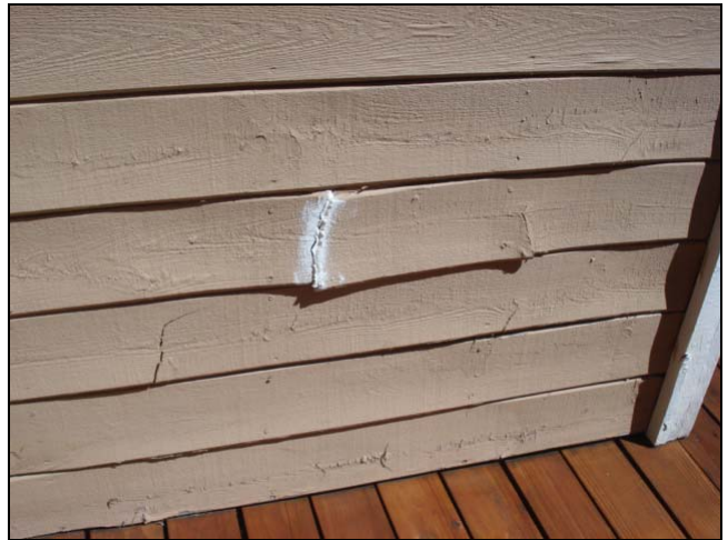
Warped and cracked lap siding.
