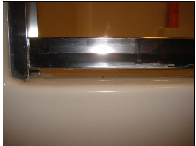
The bypass shower door track was loose.
