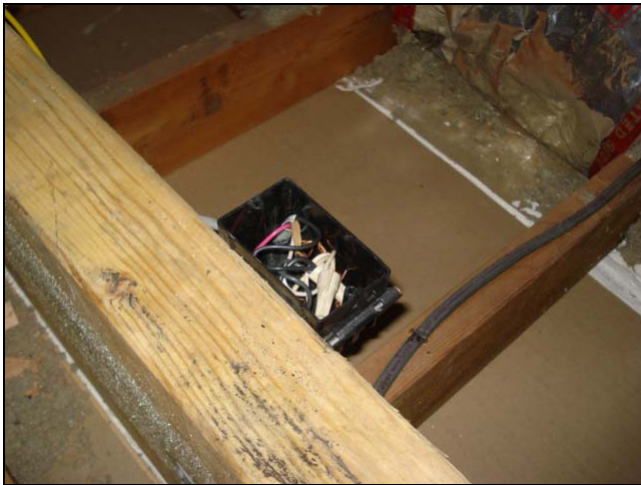
Open junction box.
