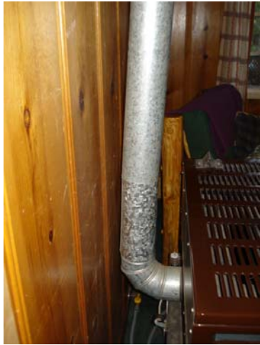
This single wall pipe was too close to the wall.
