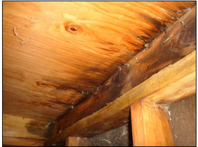
Water leak from above.
