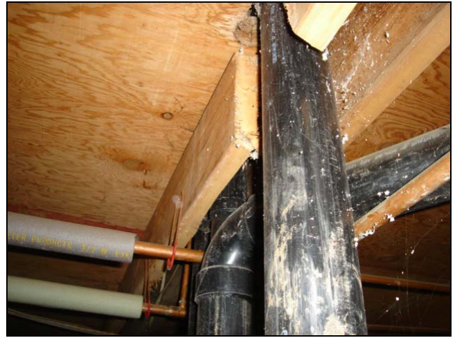
Same joist, different angle.
