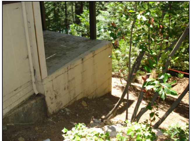
No guardrail for this ledge over 30 inches high.
