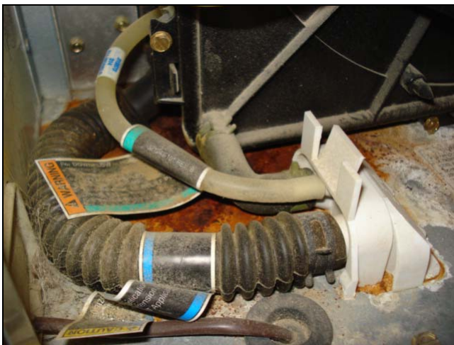
Rust from a leaking housing.
