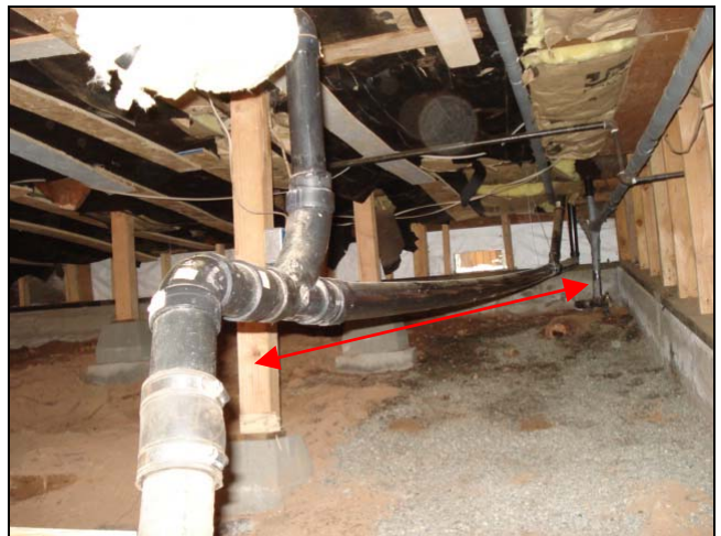
Sagging waste pipe with no support hangers.
